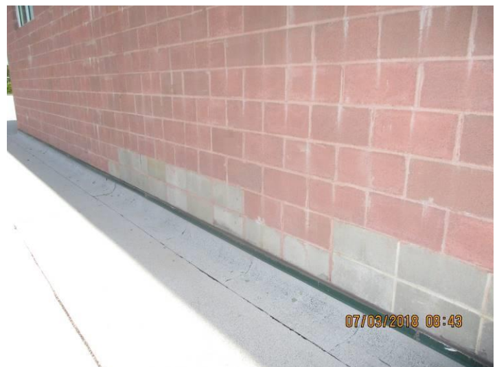
# 32: Closer view of uncoated CMU from Photograph No. 31.
