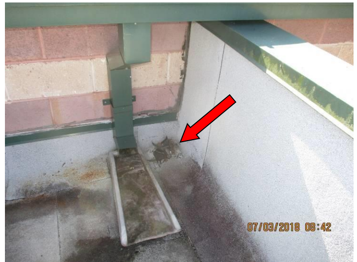
# 30: Downspouts and splash blocks are in-tact. Pre-molded plastic closures from the standing seam roof have blown loose and are stacked up in the corner.
