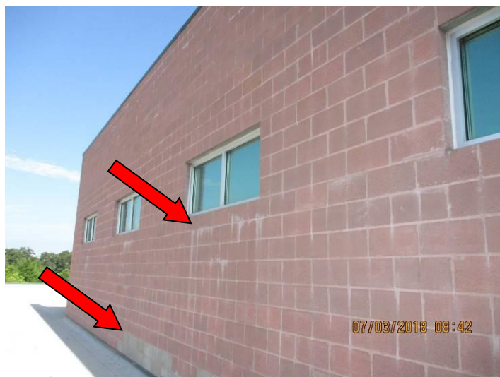
#31: Efflorescence is present throughout the wall, indicating water migrating through the coated CMU. CMU is uncoated at the base of the wall.
