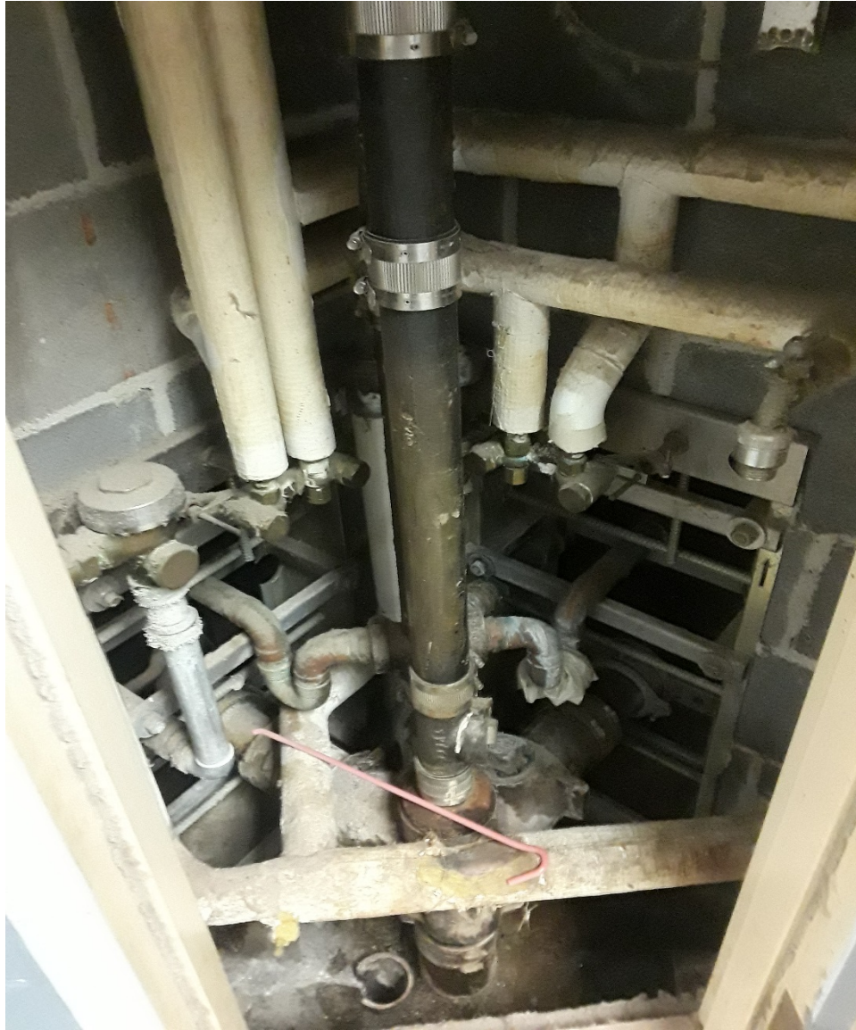
Photograph 9 Non-asbestos fiberglass pipe insulation and elbows in jail water closet.
