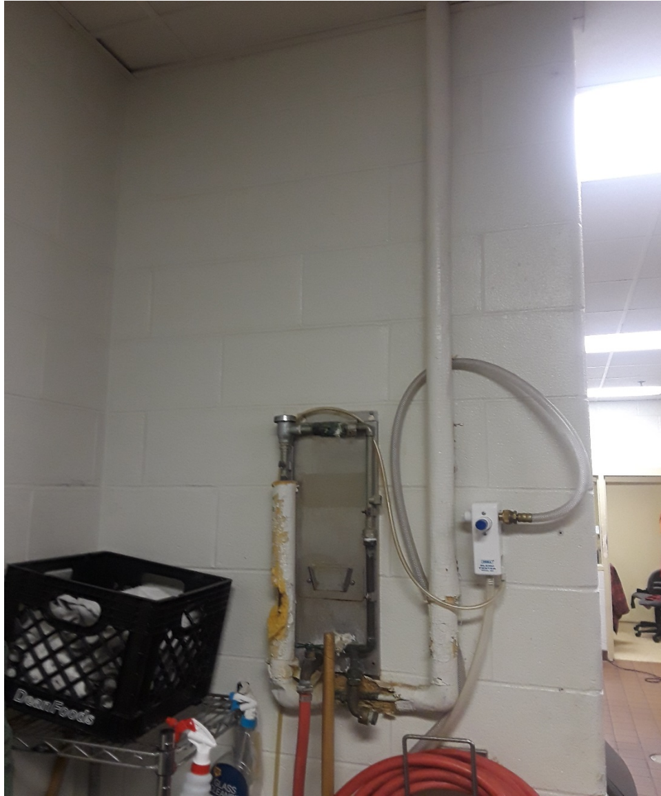
Photograph 8 Non-asbestos fiberglass pipe insulation and elbows in jail kitchen area.
