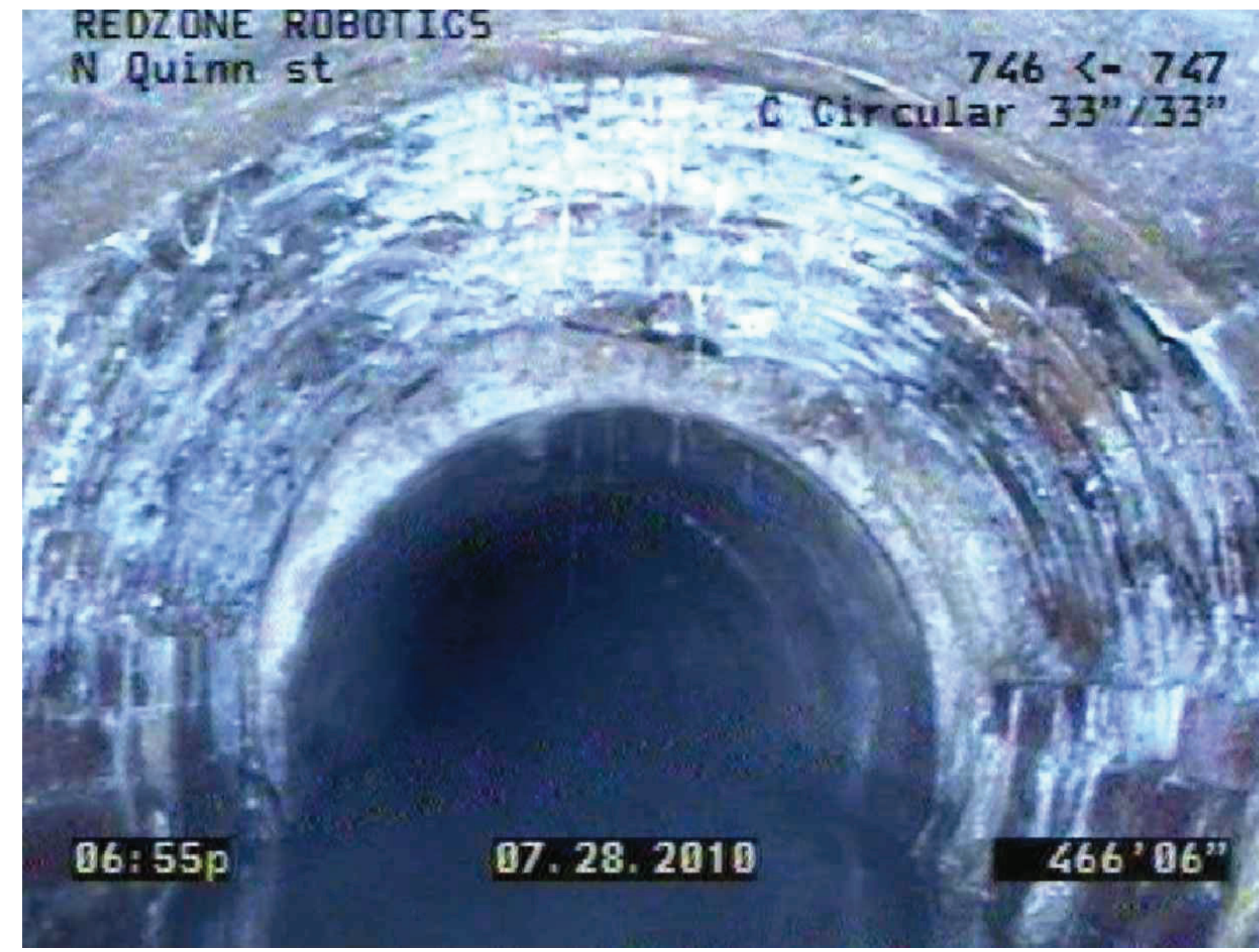
PHOTO 6 CORRUGATED METAL ON TOP OF MH 747
