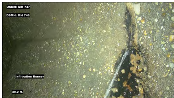
Photo: MH747_D_MH746_IR_39.2.jpg, VCR No.: 1 39.2FT, Infiltration Runner, at 02 o'clock, within 8 inches: YES
