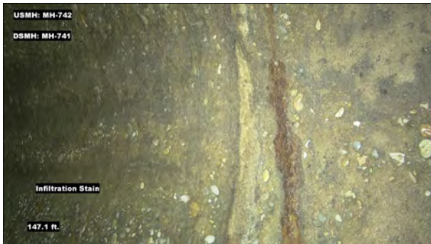
Photo: MH742_D_MH741_IS_147.1.jpg, VCR No.: 1 147.1FT, Infiltration Stain, at 02 o'clock, within 8 inches: NO
