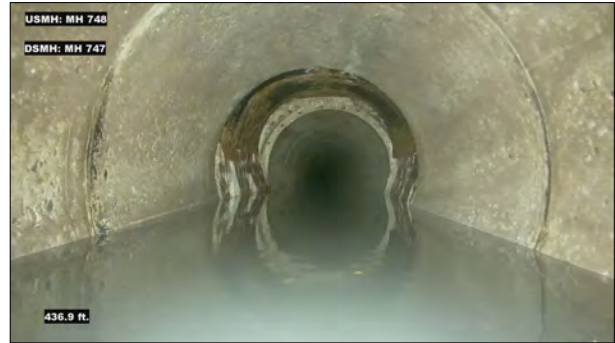
Photo: MH748_D_MH747_SAV_436.jpg, VCR No.: 1 436FT, Surface Aggregate Visible, from 08 to 04 o'clock, within 8 inches of joint: YES, Finish
