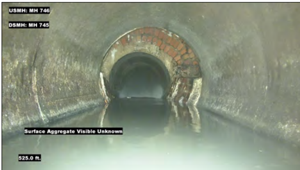
Photo: MH746_D_MH745_SAVZ_525.jpg, VCR No.: 1 525FT, Surface Aggregate Visible Unknown, from 07 to 04 o'clock, within 8 inches: NO
