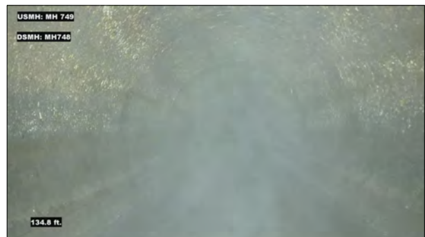
Photo: MH749_D_MH748_SAV_134.jpg, VCR No.: 1 134FT, Surface Aggregate Visible, from 09 to 03 o'clock, within 8 inches of joint: NO, Start
