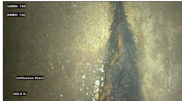
Photo: MH745_D_MH742_IS_365.8.jpg, VCR No.: 1 365.8FT, Infiltration Stain, at 02 o'clock, within 8 inches: YES
