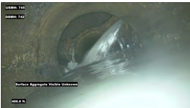
Photo: MH745_D_MH742_SAVZ_406.6.jpg, VCR No.: 1 406.6FT, Surface Aggregate Visible Unknown, from 09 to 03 o'clock, within 8 inches: NO
