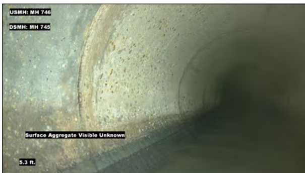
Photo: MH746_D_MH745_SAVZ_5.3.jpg, VCR No.: 1 5.3FT, Surface Aggregate Visible Unknown, from 07 to 04 o'clock, within 8 inches: NO
