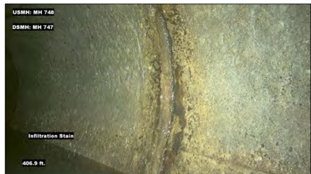
Photo: MH748_D_MH747_IS_406.9.jpg, VCR No.: 1 406.9FT, Infiltration Stain, from 03 to 05 o'clock, within 8 inches: NO
