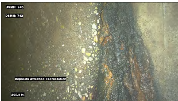
Photo: MH745_D_MH742_DAE_365.8.jpg, VCR No.: 1 365.8FT, Deposits Attached Encrustation, 5% of cross sectional area, at 03 o'clock, within 8 inches: YES
