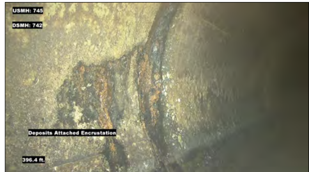
Photo: MH745_D_MH742_DAE_396.4.jpg, VCR No.: 1 396.4FT, Deposits Attached Encrustation, 5% of cross sectional area, at 10 o'clock, within 8 inches: YES
