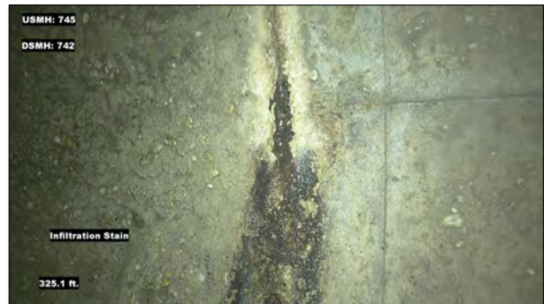
Photo: MH745_D_MH742_IS_325.1.jpg, VCR No.: 1 325.1FT, Infiltration Stain, at 02 o'clock, within 8 inches: YES
