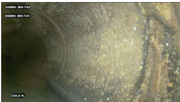
Photo: MH742_D_MH741_DAE_336.jpg, VCR No.: 1 336FT, Deposits Attached Encrustation, 5 %of cross sectional area, from 07 to 05 o'clock, , within 8 inches of joint: YES
