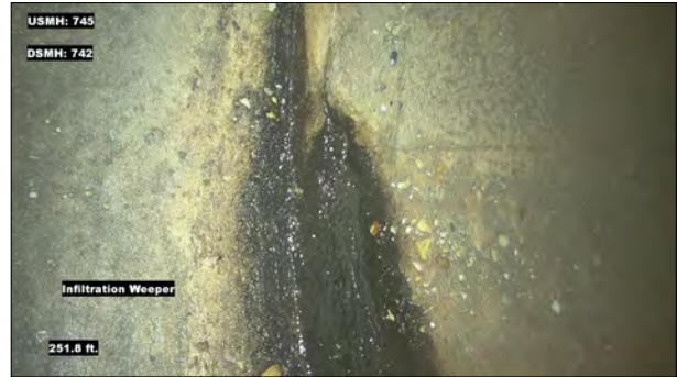
Photo: MH745_D_MH742_IW_251.8.jpg, VCR No.: 1 251.8FT, Infiltration Weeper, at 11 o'clock, within 8 inches: YES
