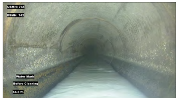
Photo: MH745_D_MH742_MWM_84.3.jpg, VCR No.: 1 84.3FT, Water Mark, 25% of cross sectional area
