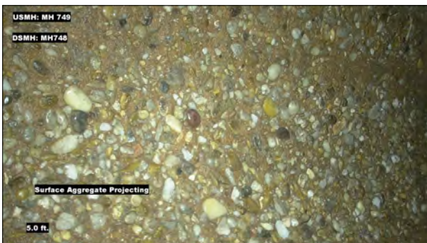
Photo: MH749_D_MH748_SAP_5.jpg, VCR No.: 1 5FT, Surface Aggregate Projecting, from 07 to 05 o'clock, within 8 inches: YES
