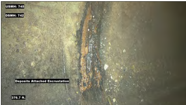
Photo: MH745_D_MH742_DAE_376.7.jpg, VCR No.: 1 376.7FT, Deposits Attached Encrustation, 5% of cross sectional area, at 11 o'clock, within 8 inches: YES
