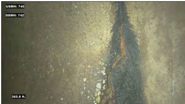
Photo: MH745_D_MH742_CC_365.jpg, VCR No.: 1 365FT, Crack Circumferential, from 08 to 05 o'clock, within 8 inches of joint: NO
