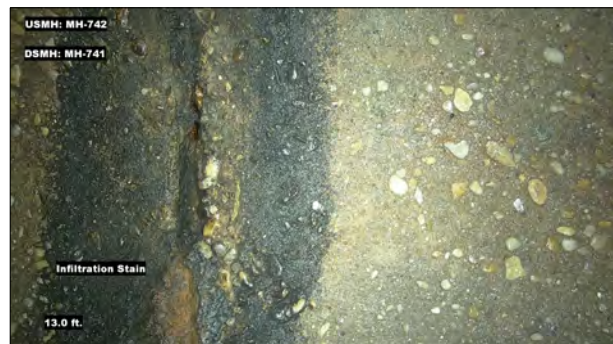
Photo: MH742_D_MH741_IS_13.jpg, VCR No.: 1 13FT, Infiltration Stain, at 04 o'clock, within 8 inches: YES
