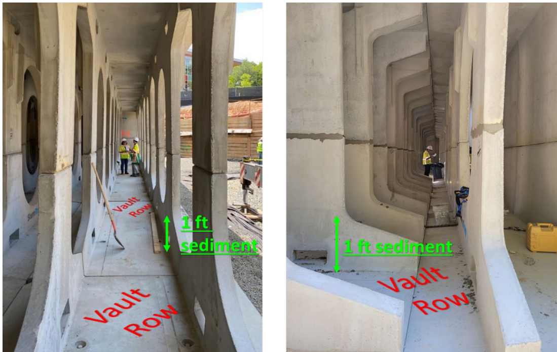
Figure 6. The vault rows and time trigger for maintenance (1 foot of sediment captured in the vault row).
