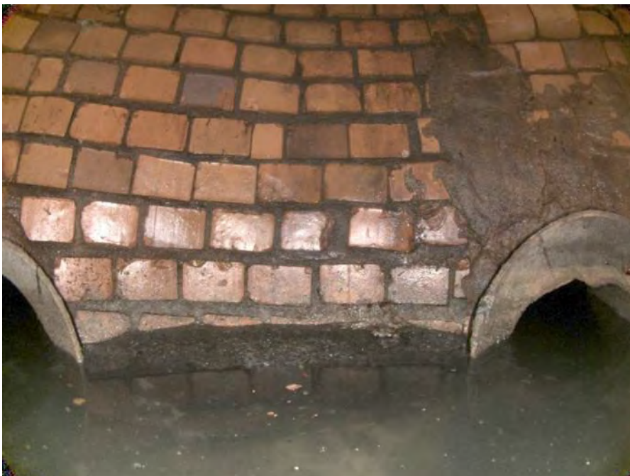
1818_a75925b2-5868-48ca-b1fe-f6e0ecc4562_8e3fa862-3c75-4213-aac0-620618a96e8d_P11.jpg, 00:00:36, 8.66 Infiltration Stain from 7 o'clock to 12 o'clock, within 8 inch
