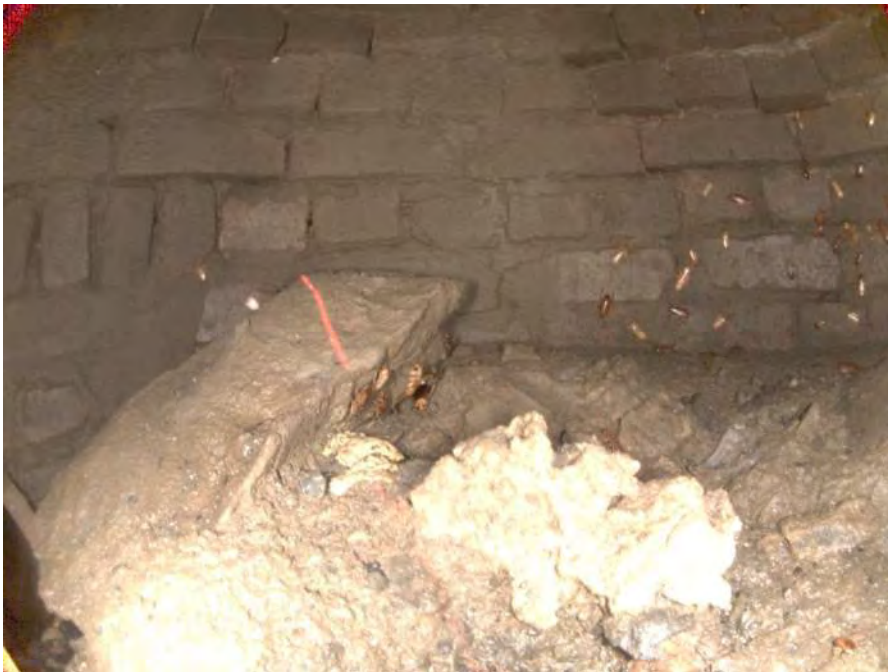
1821_b79fd861-dd10-4846-a6c3-82d3d499c9c7_0bc5d1de-e242-4391-b787-4bef6b28f7b0_PI1.jpg, 00:00:17, 3.83 Obstruction Construction Debris, 35% of cross sectional area from 12 o'clock to 12 o'clock
