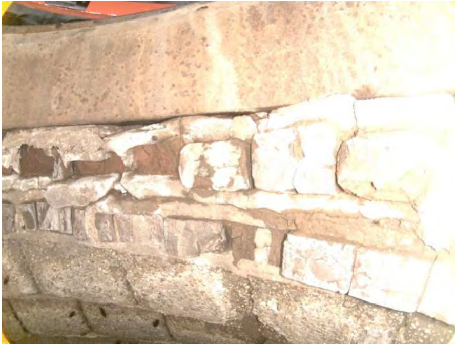
1835c_f2d6f72e-14ab-43ef-906b-8e360bc88926_92e8571e-9460-4688-88e8-b2a276872e7c_P11.jpg, , 0.94 Missing Mortar Large from 12 o'clock to 11 o'clock, Start
