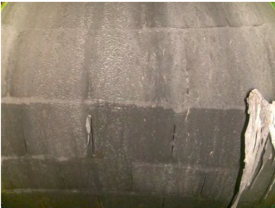
1837c_166883a2-6c9f-44dc-8d3b-993be20f6dc6_1649f046-1a82-498d-82e2-e1f4de576c6f_PI1.jpg, 00:00:13, 2.11 Missing Mortar Large from 12 o'clock to 12 o'clock
