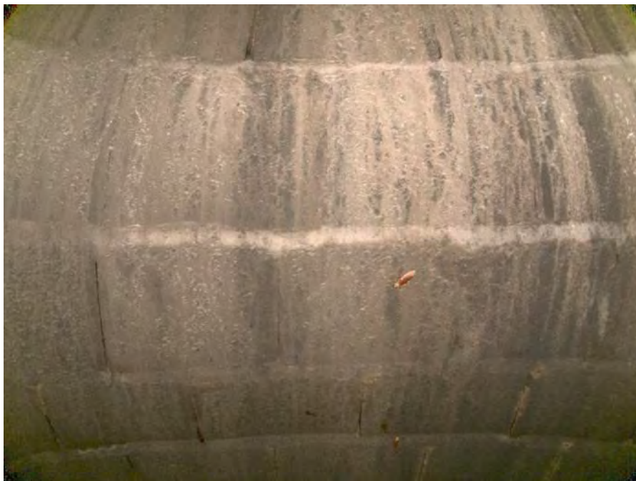
1839_f7a2e778-f07c-460d-8979-384ad1d2d1b3_2ceee7b3-5cb1-48fb-b1bd-03d0ef3fc47e_P11.jpg, 00:00:17, 2.77 Missing Mortar Large from 12 o'clock to 12 o'clock
