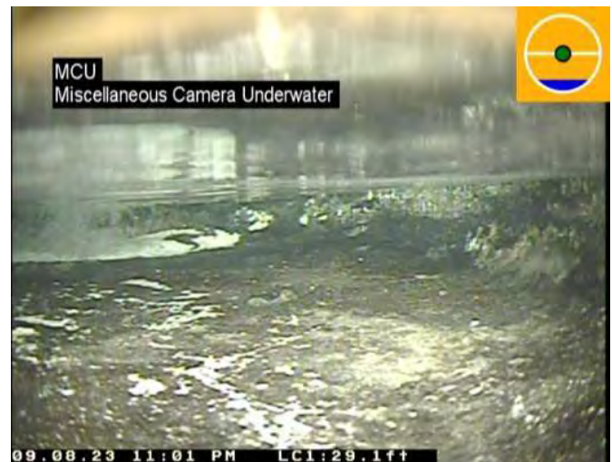
Distance: 29.1 ft. Grade: 4 Condition: Miscellaneous Camera Underwater Remarks: CAMERA UNDERWATER BEFORE MH
