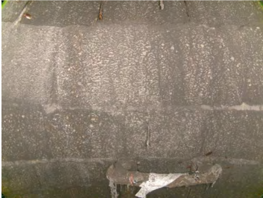
1838_4d464b94-a957-4557-a7ae-8bb14bf4d783_e264c322-c1cf-4ac7-a7cc-1ded439b5dae_PI1.jpg, 00:00:15, 2.72 Missing Mortar Large from 12 o'clock to 12 o'clock
