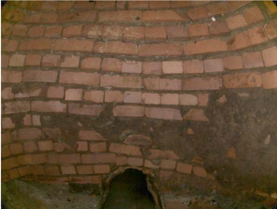
1833a_415896af-f5e7-4861-970c-902a07ead962_ea4a1f46-26fb-4252-8332-37380d041f3c_P11.jpg, 00:00:27, 5.72 Missing Mortar Large from 12 o'clock to 12 o'clock
