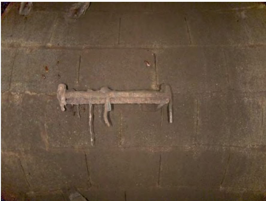
1841a_7e3e94ed-5602-4c81-88a8-bfb0bb428782_daacd105-63d3-4004-8c79-a586eef84f9f_P11.jpg, 00:00:30, 7.10 Deposits Attached Ragging, 5% of cross sectional area from 8 o'clock to 12 o'clock, within 8 inch
