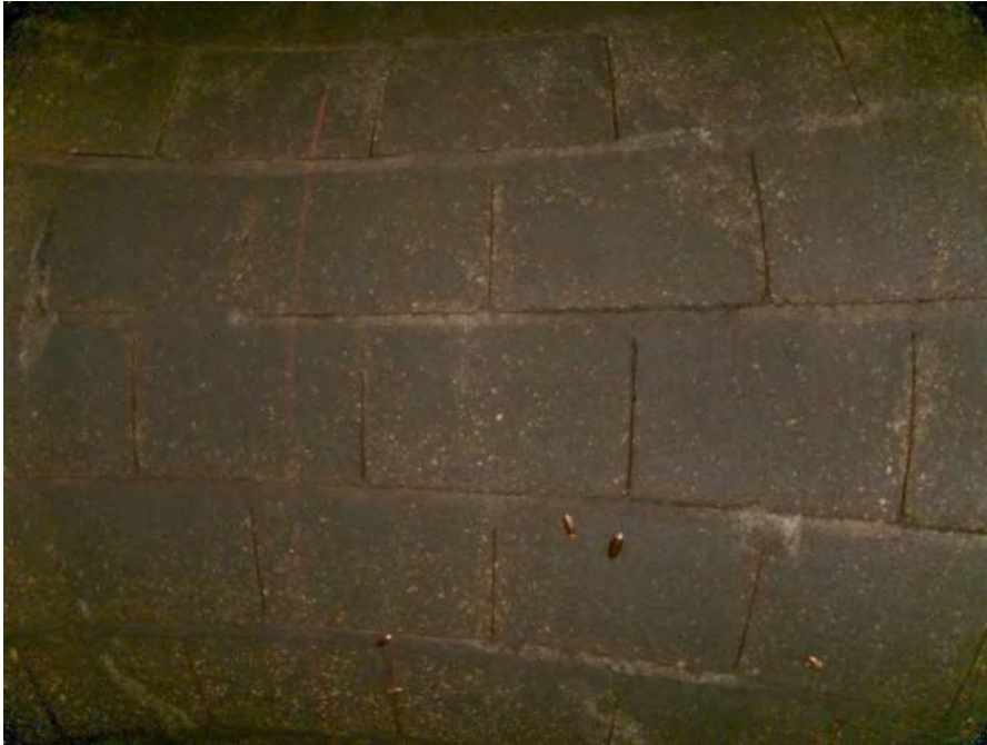
1842_98b1de5e-0e50-41ed-b476-ff581fdb636e_ec832979-62f8-4c91-8da5-8ac031d99ae4_P11.jpg, 00:00:32, 6.40 Surface Damage Aggregate Visible from 12 o'clock to 12 o'clock, within 8 inch
