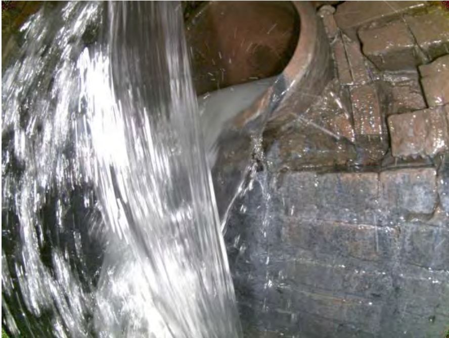
1828b_5154b3dc-7153-4625-bad4-be8d5b792f69_bcfea9bc-7934-4eb7-bd36-91ffe877c936_P11.jpg, 00:00:44, 9.50 Missing Mortar Large from 12 o'clock to 12 o'clock
