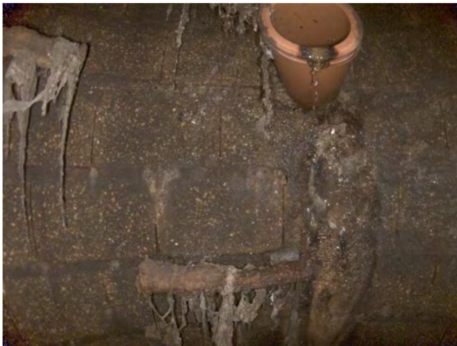
1837c_166883a2-6c9f-44dc-8d3b-993be20f6dc6_18e86ff1-c566-4871-a18d-85e9d3777971_P11.jpg, 00:00:29, 6.29 Infiltration Weeper from 10 o'clock to 11 o'clock, within 8 inch
