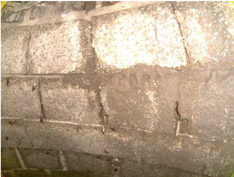
1835c_f2d6f72e-14ab-43ef-906b-8e360bc88926_c2591e1a-3356-420c-b13d-3df3d302536e_P11.jpg, 00:00:13, 2.32 Missing Mortar Large from 12 o'clock to 12 o'clock
