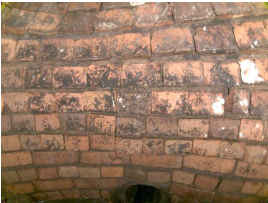
2193c_2b27c63e-1844-43c6-8c49-44849fa40c9a_7338876b-4b2d-4dae-8d83-3970418e4892_P11.jpg, 00:00:14, 2.15 Missing Mortar Large from 12 o'clock to 12 o'clock
