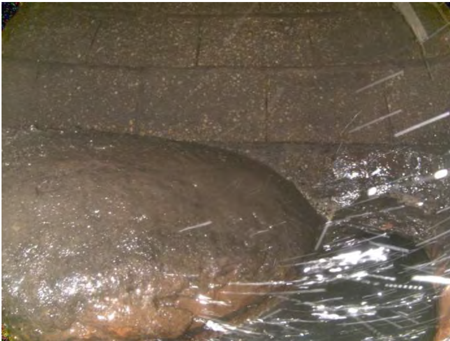
1838_4d464b94-a957-4557-a7ae-8bb14bf4d783_bcf02ece-7deb-4f88-be2a-457d033fda34_P11.jpg, 00:00:38, 8.39 Infiltration Weeper from 5 o'clock to 7 o'clock, within 8 inch
