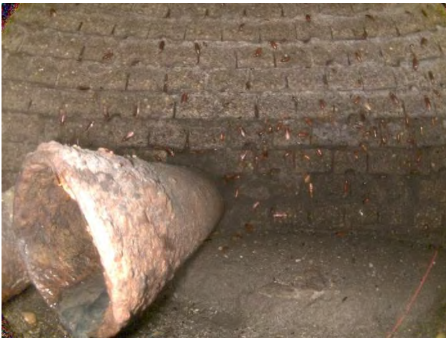
1823d_c2435bdb-6471-4a3b-8f5b-2755123d82bf_d6e66fc7-c2a3-4ae1-a821-d9494e359c22_P11.jpg, 00:00:14, 3.45 Infiltration Stain from 12 o'clock to 12 o'clock, within 8 inch
