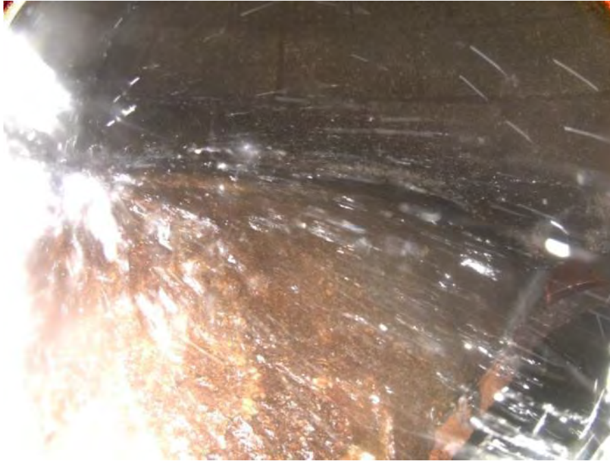
1838_4d464b94-a957-4557-a7ae-8bb14bf4d783_8215d7ef-ee63-4f71-aeed-bba2ebaa76ec_P11.jpg, 00:00:38, 8.46 Infiltration Weeper from 12 o'clock to 1 o'clock, within 8 inch
