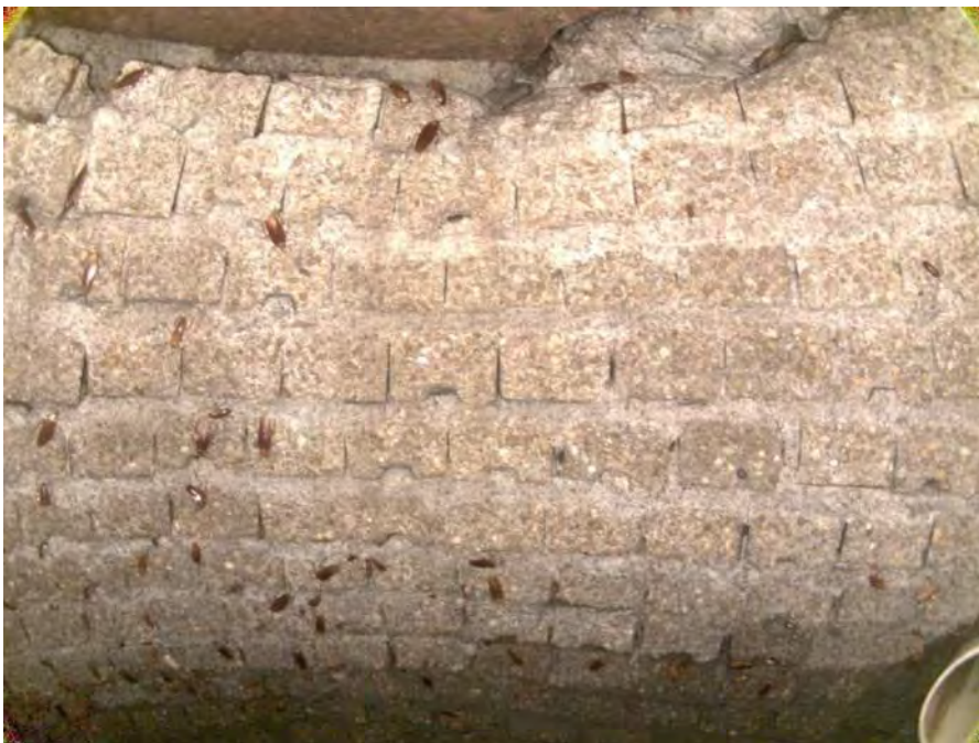
1823d_c2435bdb-6471-4a3b-8f5b-2755123d82bf_3c920d25-da83-4924-ac81-5ffd8014f1a_P11.jpg, 00:00:10, 1.87 Missing Mortar Large from 12 o'clock to 12 o'clock
