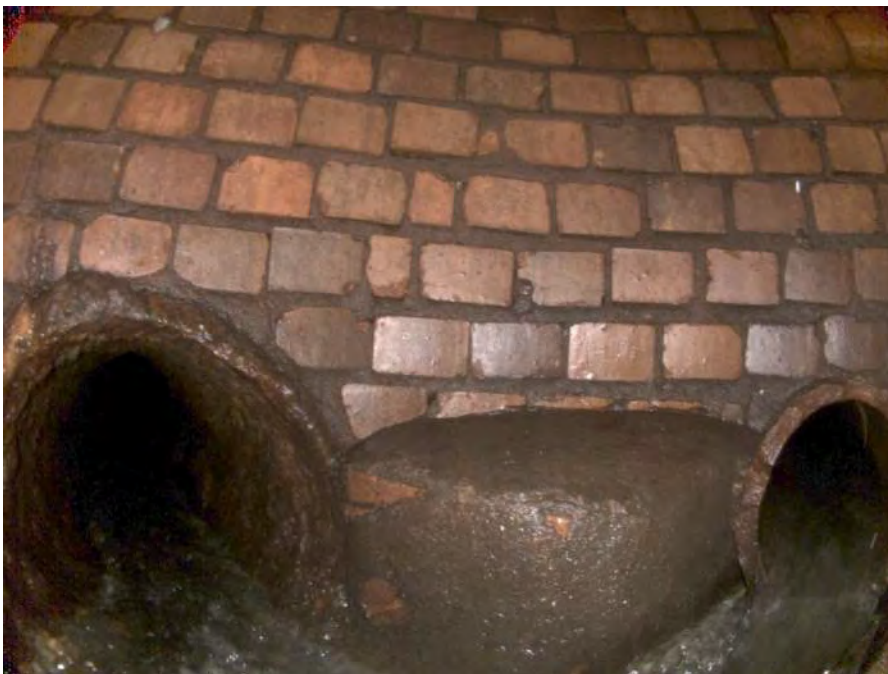
1819_3d72062a-4862-48ce-be8e-7bbe04d95bb2_00b5059a-7ab1-4e45-9d64-250f6cb011a2_P11.jpg, 00:00:36, 8.01 Infiltration Weeper from 5 o'clock to 7 o'clock, within 8 inch
