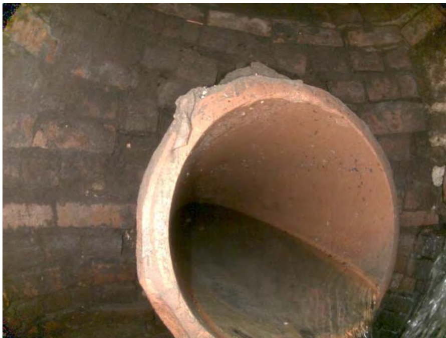
1828b_5154b3dc-7153-4625-bad4-be8d5b792f69_edb4c192-5e6a-4281-8e16-ea99f963de5c_P11.jpg, 00:00:32, 6.58 Missing Mortar Large from 12 o'clock to 12 o'clock
