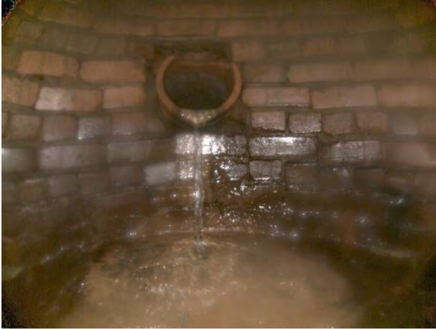
1830_f8e692ed-45a5-4111-be6d-dbb6437dd8b2_d363373a-311b-4f24-a0ef-09d577813ae1_P11.jpg, 00:00:37, 7.77 Infiltration Weeper from 12 o'clock to 12 o'clock, within 8 inch
