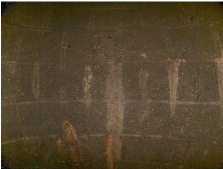
1840b_b7eec4bd-8b4a-4779-9657-5106bc04b13d_0bacfebb-7abc-441d-9d7c-0f90eb9de052_P11.jpg, 00:00:30, 7.10 Infiltration Stain from 10 o'clock to 8 o'clock, within 8 inch
