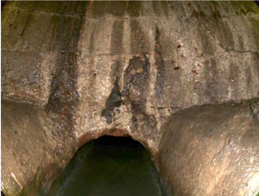
1839_f7a2e778-f07c-460d-8979-384ad1d2d1b3_f0b0d505-39c7-45cf-a092-b070cc688200_P11.jpg, 00:00:43, 9.11 Infiltration Weeper Connection from 5 o'clock to 7 o'clock, within 8 inch
