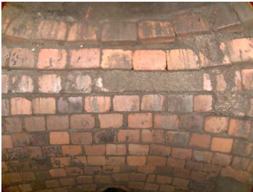
2194_1962243a-d72d-4c62-9e3a-2c87a26c1c57_f68e1b1f-3d93-4c0c-8e24-01f9fd97e403_PI1.jpg, 00:00:15, 1.99 Missing Mortar Large from 12 o'clock to 12 o'clock
