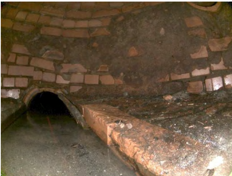
1833a_415896af-f5e7-4861-970c-902a07ead962_d9ee26c7-bdf7-4ce9-802e-334e49f7b47d_P11.jpg, 00:00:32, 7.02 Infiltration Stain from 6 o'clock to 11 o'clock, within 8 inch
