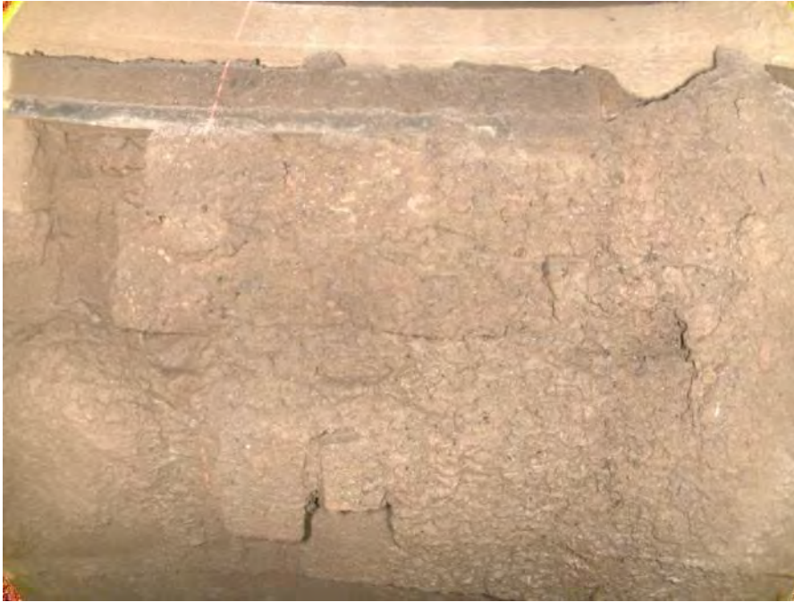
1840b_b7eec4bd-8b4a-4779-9657-5106bc04b13d_7555dfaa-36ec-44d8-94fd-88d879b45a7c_P11.jpg, 00:00:08, 1.15 Missing Mortar Medium from 12 o'clock to 12 o'clock
