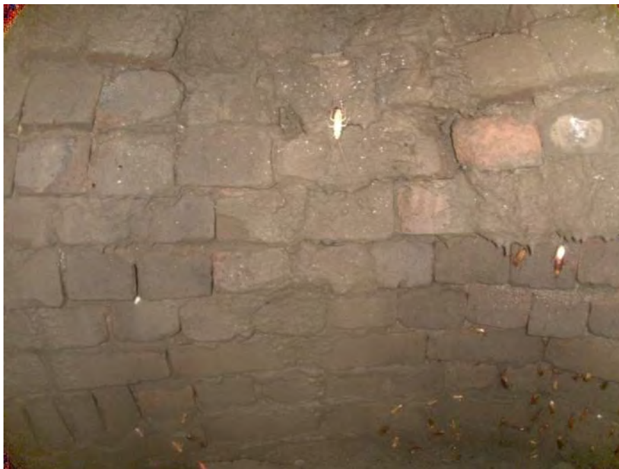
1821_b79fd861-dd10-4846-a6c3-82d3d499c9c7_b8dbdadb-54ad-48eb-bc30-e877ffbcd1a4_P11.jpg, 00:00:13, 2.00 Missing Mortar Large from 12 o'clock to 12 o'clock
