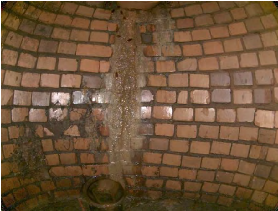
1818_a75925b2-5868-48ca-b1fe-f6e0ecc4562_dd159dc7-5399-49fc-888f-b48a01663db8_P11.jpg, 00:00:31, 7.17 Missing Mortar Large from 12 o'clock to 12 o'clock
