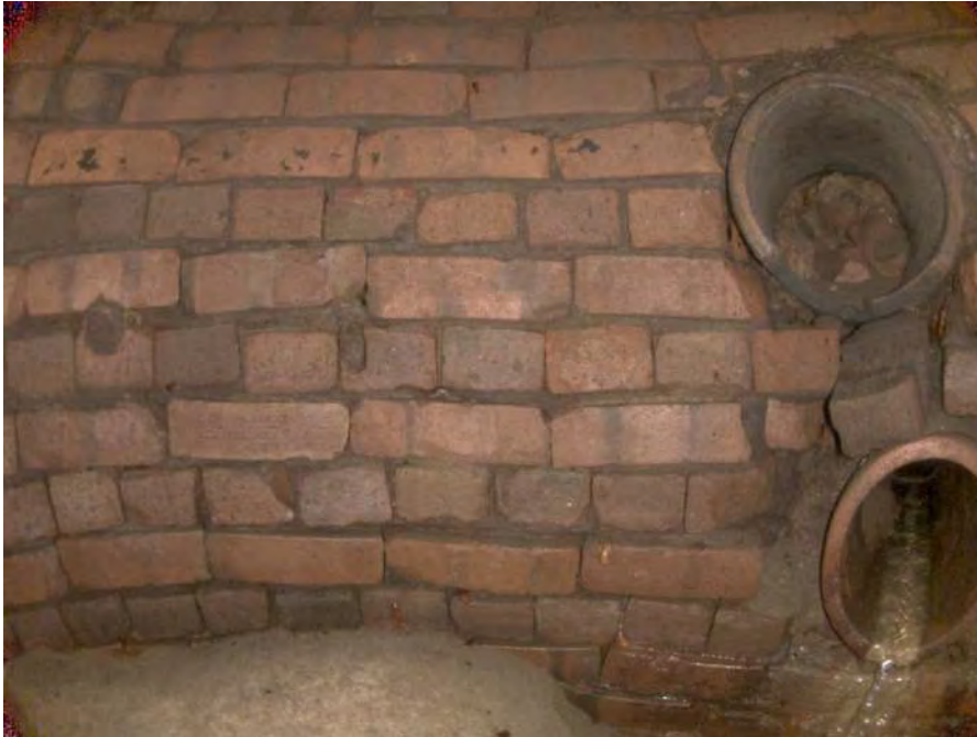
1834b_16edcb0d-7f2c-4b5a-bd27-6b0d1bf9d1bd_28df1de4-7227-40c4-98d3-59bc5e7280d2_P11.jpg, 00:00:27, 6.46 Displaced Brick from 11 o'clock to 1 o'clock
