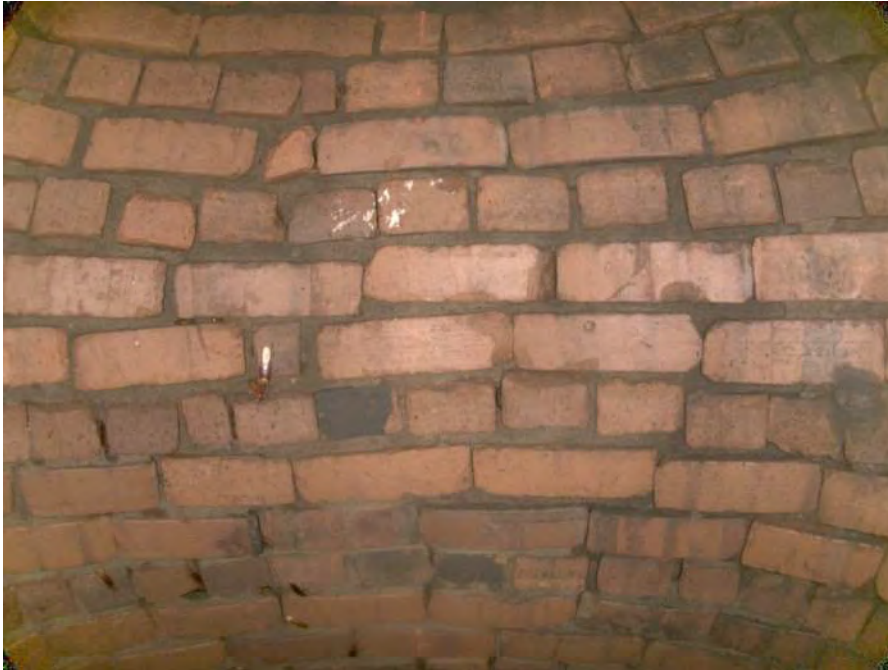
1829b_c3bb5419-4fc2-49bd-9cbb-ae8a522c6251_d20457a7-fd48-4840-a563-c6483aa35cbf_P11.jpg, 00:00:21, 4.81 Missing Mortar Large from 12 o'clock to 12 o'clock
