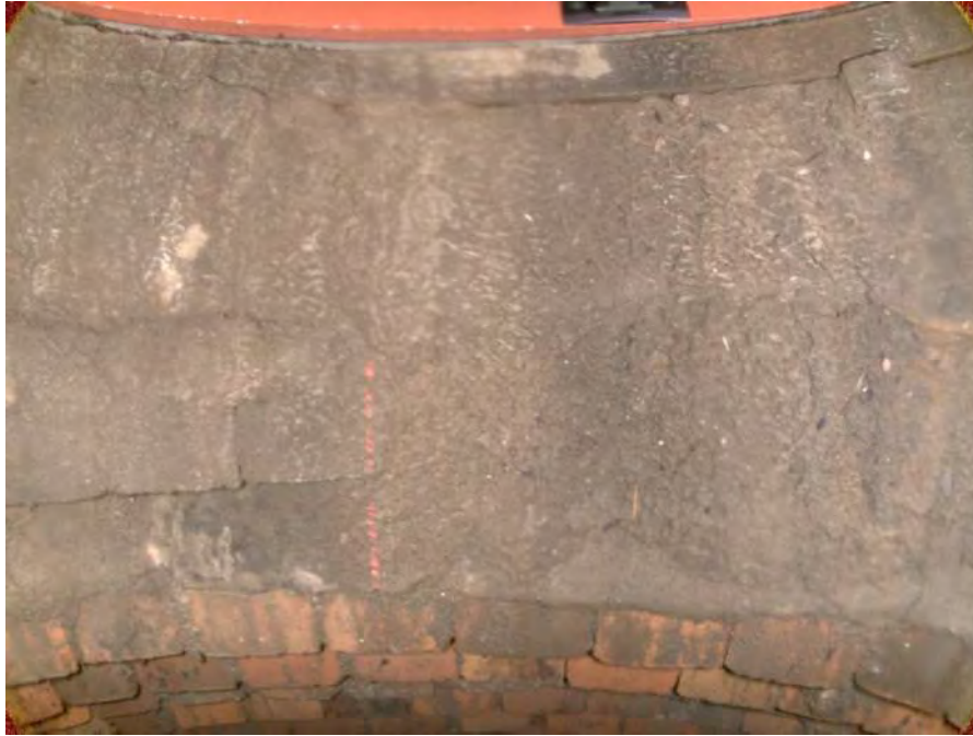
2194_1962243a-d72d-4c62-9e3a-2c87a26c1c57_aeb8bf8d-f294-49aa-a231-debc66a1da36_PI1.jpg, 0.73 Missing Mortar Medium from 12 o'clock to 12 o'clock
