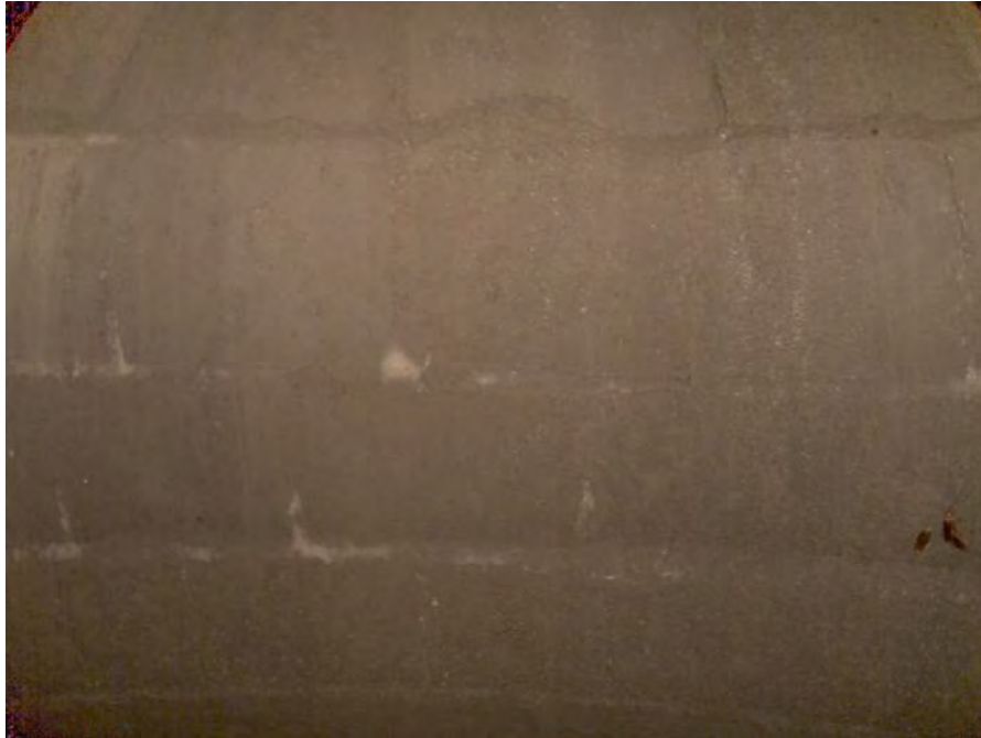
1840b_b7eec4bd-8b4a-4779-9657-5106bc04b13d_b3bd481c-4d93-4b3a-82bb-d7009eb967ba_P11.jpg, 00:00:15, 3.19 Missing Mortar Large from 12 o'clock to 12 o'clock
