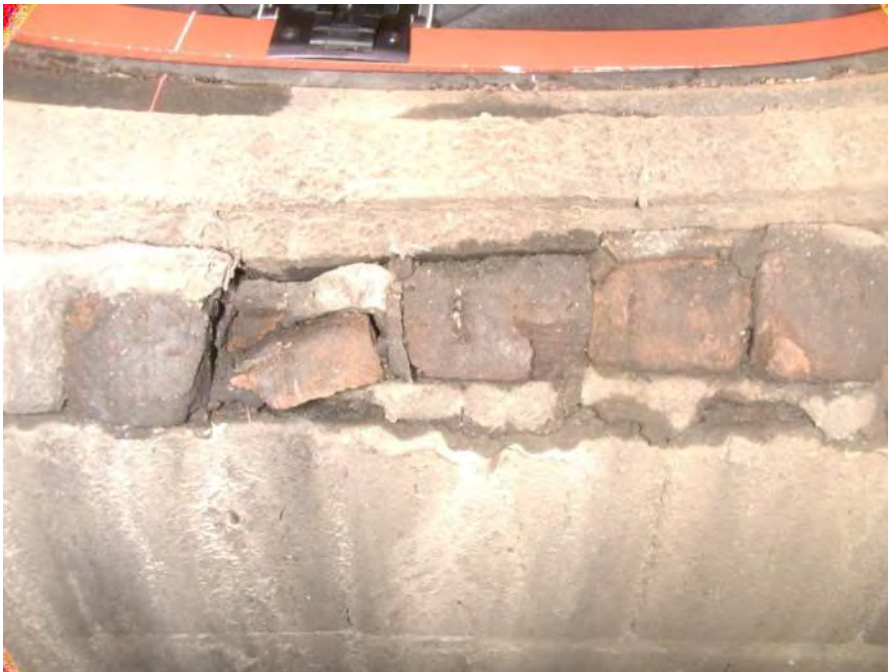
1837c_166883a2-6c9f-44dc-8d3b-993be20f6dc6_f4da2fc8-9b38-41b2-883b-1d13218a253a_P11.jpg, 00:00:00, 0.66 Displaced Brick from 6 o'clock to 8 o'clock
