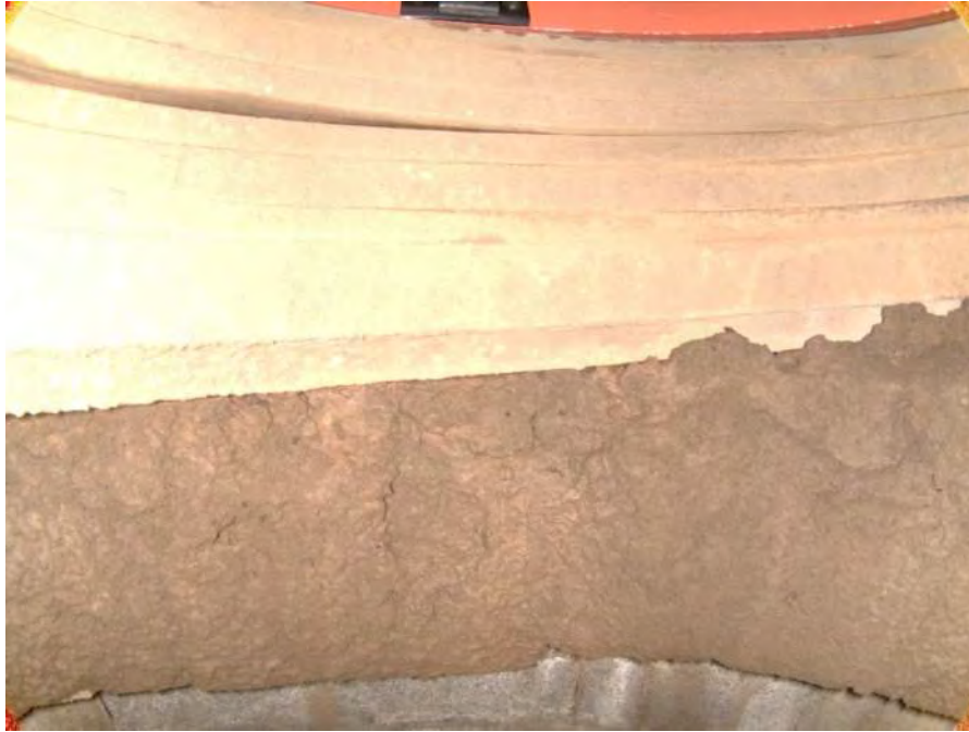
1841a_7e3e94ed-5602-4c81-88a8-bfb0bb428782_5ec9646d-4da9-4be7-a8c7-3f5e4dbdd8f5_P11.jpg, 00:00:08, 1.01 Missing Mortar Small from 1 o'clock to 6 o'clock
