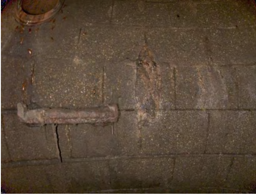
1840b_b7eec4bd-8b4a-4779-9657-5106bc04b13d_7d43213e-f383-41b4-bd9d-7330807a6025_P11.jpg, 00:00:36, 8.56 Infiltration Weeper from 11 o'clock to 12 o'clock, within 8 inch
