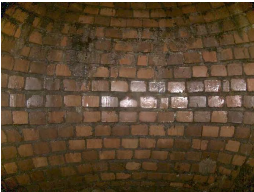
1819_3d72062a-4862-48ce-be8e-7bbe04d95bb2_49e29911-486c-4574-8c37-30f56f9aaa5d_P11.jpg, 00:00:30, 6.41 Infiltration Weeper from 11 o'clock to 3 o'clock, within 8 inch
