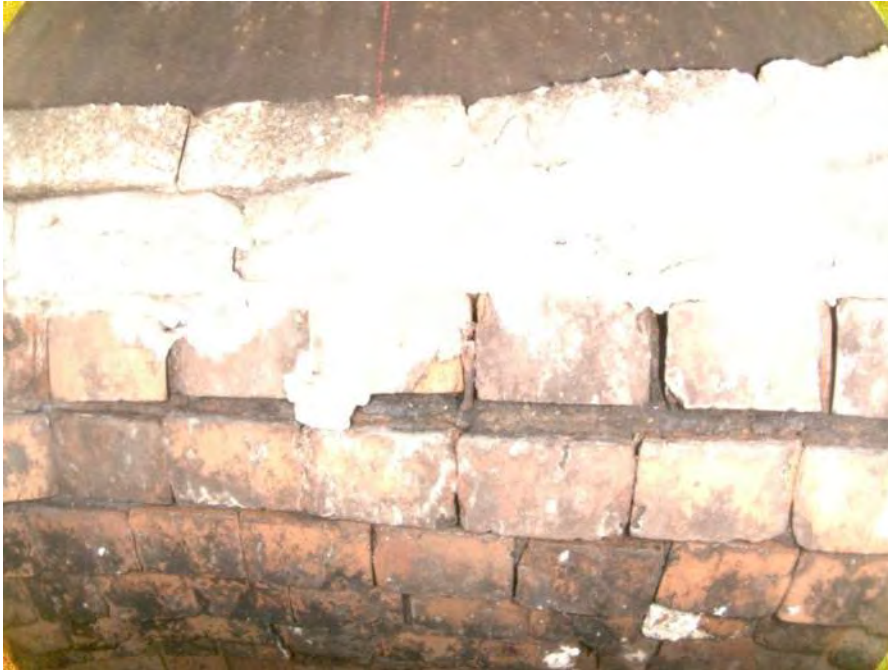
2193c_2b27c63e-1844-43c6-8c49-44849fa40c9a_27231513-463e-40f2-a886-37276c3d5b57_P11.jpg, 1.12 Missing Mortar Large from 12 o'clock to 12 o'clock
