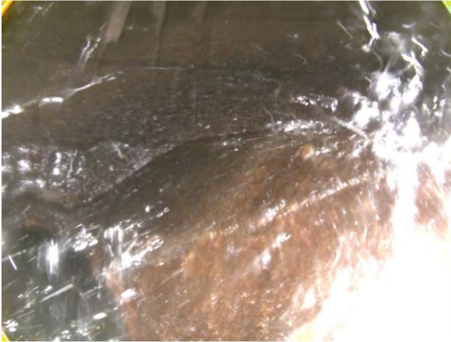
1838_4d464b94-a957-4557-a7ae-8bb14bf4d783_04cfbab0-958e-48d8-82d2-5ef393c965f4_P11.jpg, 00:00:38, 8.37 Crack Longitudinal at 7 o'clock, within 8 inch
