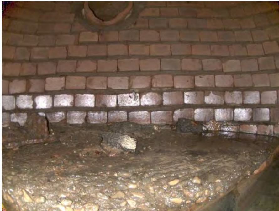
1831_511dce6f-34cf-4134-8589-97e8cd9b2803_ad7a6b38-3803-4d93-8950-c59468f78ae6_P11.jpg, 00:00:32, 6.81 Infiltration Stain from 7 o'clock to 12 o'clock, within 8 inch
