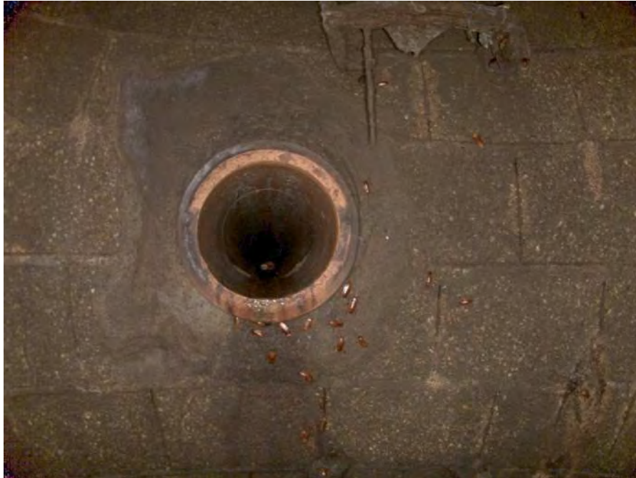
1840b_b7eec4bd-8b4a-4779-9657-5106bc04b13d_35529e95-0a62-48f8-98e8-335a84118c73_P11.jpg, 00:00:31, 7.26 Deposits Attached Ragging, 5% of cross sectional area from 9 o'clock to 12 o'clock, within 8 inch
