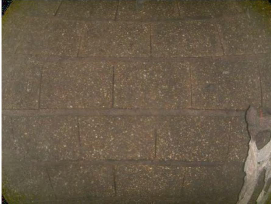
1838_4d464b94-a957-4557-a7ae-8bb14bf4d783_b3954de8-385d-4369-9bee-3867a1223ba2_P11.jpg, 00:00:28, 6.10 Surface Damage Aggregate Visible from 12 o'clock to 12 o'clock, within 8 inch
