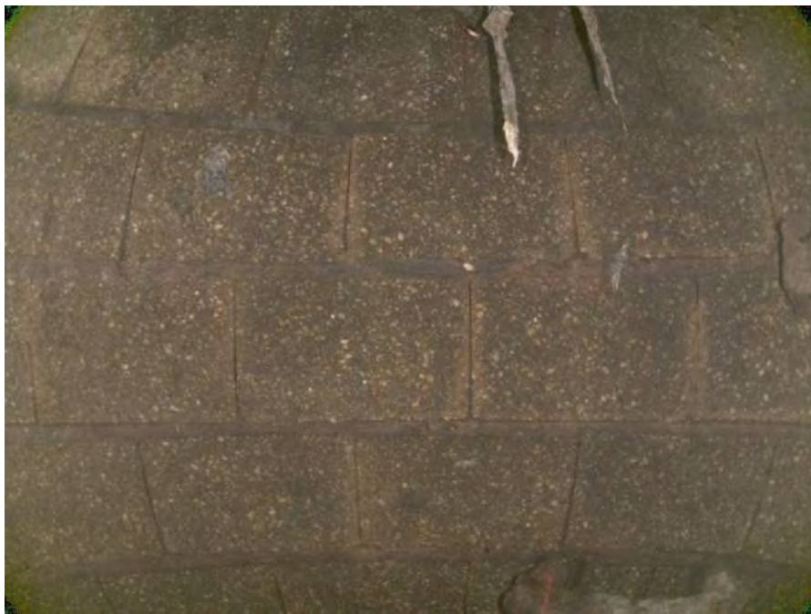
1838_4d464b94-a957-4557-a7ae-8bb14bf4d783_2af9f40c-8e6b-4a28-8936-9ca041e50edf_PI1.jpg, 00:00:23, 4.86 Deposits Attached Ragging, 5% of cross sectional area from 6 o'clock to 8 o'clock, within 8 inch
