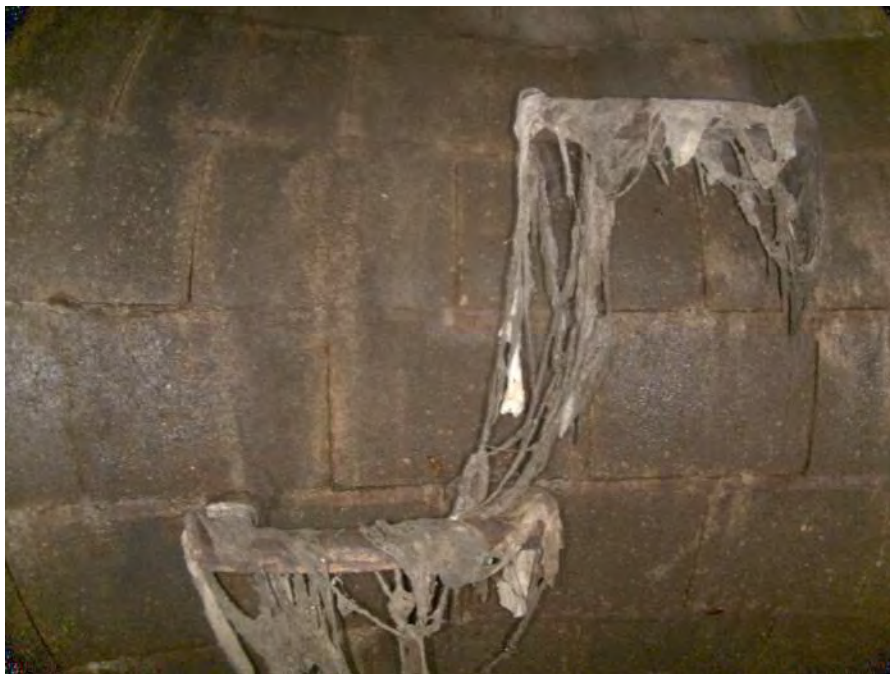
1842_98b1de5e-0e50-41ed-b476-ff581fdb636e_59d47be1-5aec-4a1d-aa9f-42075eb1f695_PI1.jpg, , 5.45 Deposits Attached Ragging, 5% of cross sectional area from 11 o'clock to 2 o'clock, within 8 inch
