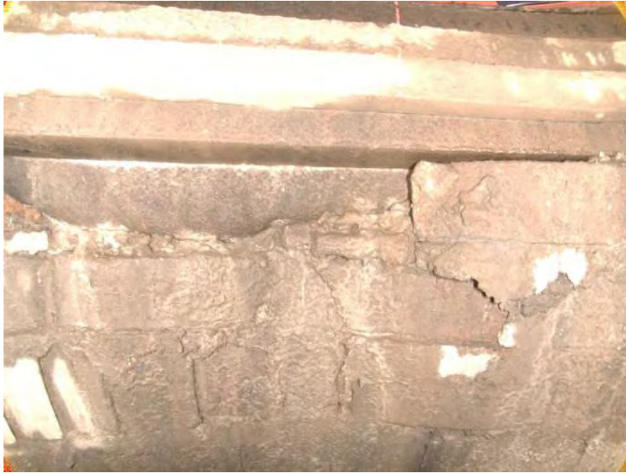
1839_f7a2e778-f07c-460d-8979-384ad1d2d1b3_31e68735-8741-46f8-a0f5-72a580d3aa28_P11.jpg, 00:00:09, 0.84 Missing Brick from 3 o'clock to 6 o'clock
