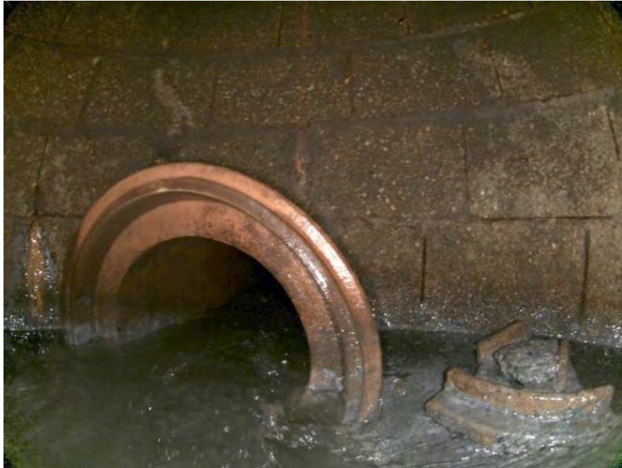
1842_98b1de5e-0e50-41ed-b476-ff581fdb636e_da26af56-9524-4d1f-8dc6-a1a065c0e713_PI1.jpg, 00:00:43, 9.47 Obstruction Construction Debris, 5% of cross sectional area from 7 o'clock to 9 o'clock
