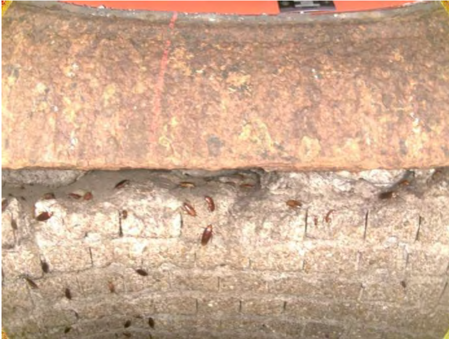
1823d_c2435bdb-6471-4a3b-8f5b-2755123d82bf_2abfd172-3343-4967-8249-fb00c0f1d705_P11.jpg, 0.89 Missing Mortar Medium from 12 o'clock to 12 o'clock
