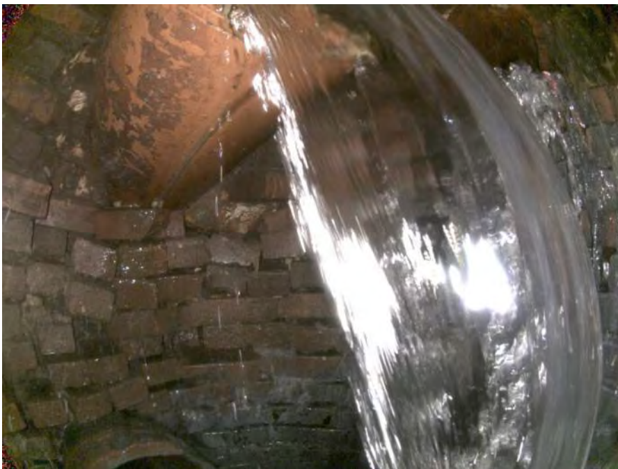
1828b_5154b3dc-7153-4625-bad4-be8d5b792f69_a9eef5b8-2357-475d-a879-3b8cd9676573_P11.jpg, 00:00:39, 8.18 Displaced Brick from 8 o'clock to 11 o'clock
