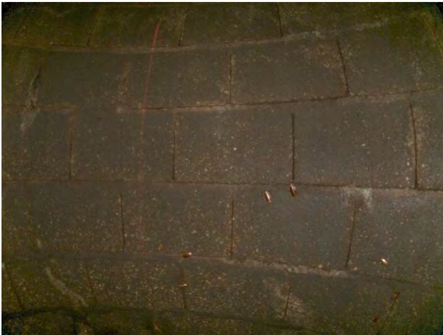
1842_98b1de5e-0e50-41ed-b476-ff581fdb636e_dcbefd8a-b7e6-401c-9a30-5acdf49e2291_P11.jpg, 00:00:33, 6.73 Missing Mortar Large from 12 o'clock to 12 o'clock
