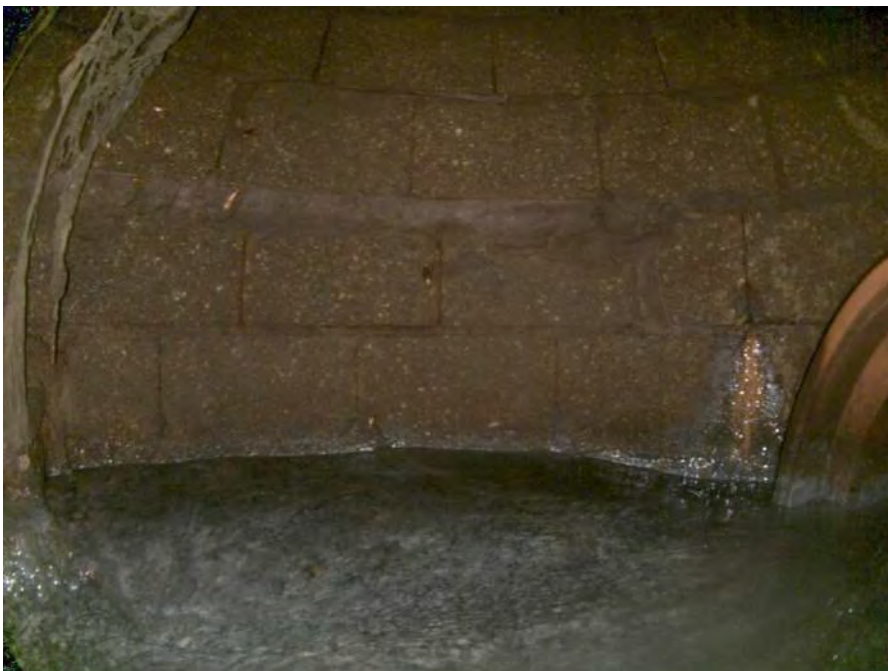
1842_98b1de5e-0e50-41ed-b476-ff581fdb636e_20bb308d-109f-4d91-8794-926c0ba74d99_PI1.jpg, 00:00:42, 8.87 Infiltration Weeper from 4 o'clock to 6 o'clock, within 8 inch
