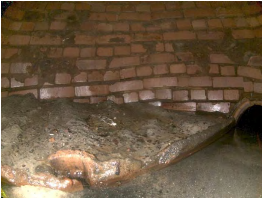
1833a_415896af-f5e7-4861-970c-902a07ead962_67f78bf4-e94b-4f03-8b46-ec002a1f34f9_P11.jpg, 00:00:32, 7.50 Deposits Settled Fine, 45% of cross sectional area from 12 o'clock to 12 o'clock, within 8 inch
