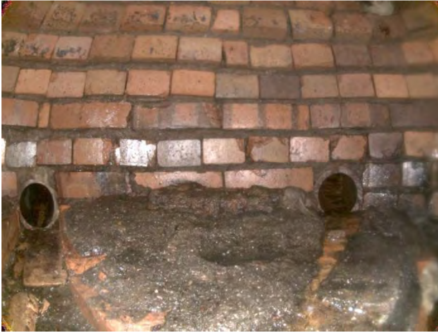
2193c_2b27c63e-1844-43c6-8c49-44849fa40c9a_6167233f-25d9-4a6c-8135-a91386f86965_P11.jpg, 00:00:17, 3.80 Deposits Attached Grease, 5% of cross sectional area from 5 o'clock to 7 o'clock, within 8 inch
