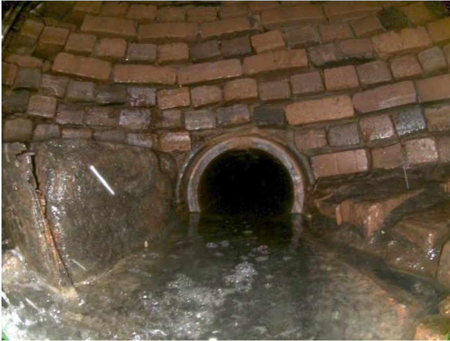
1829b_c3bb5419-4fc2-49bd-9cbb-ae8a522c6251_f3ab9e9f-2c73-4d4d-b4f0-7177eac04aa9_P11.jpg, 00:00:43, 10.68 Missing Mortar Large from 12 o'clock to 12 o'clock
