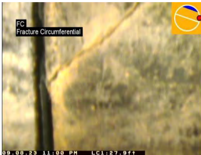
Distance: 27.8 ft. Grade: 2 Condition: Fracture Circumferential Remarks: FRACTURED AT JOINT
