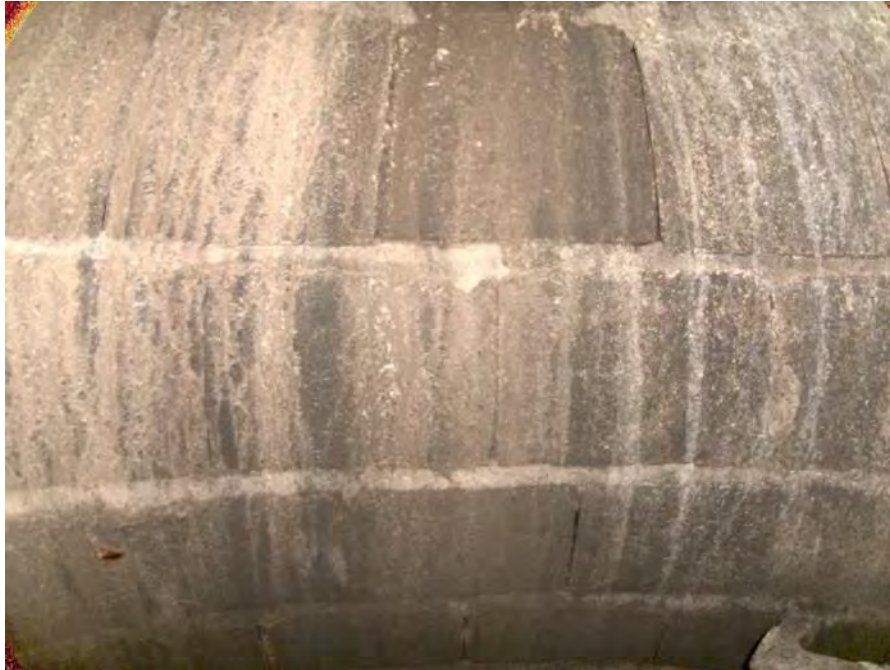
1839_f7a2e778-f07c-460d-8979-384ad1d2d1b3_ee7ac1aa-28e5-461c-bbd2-05e6ce6ef2a0_P11.jpg, 00:00:15, 2.33 Infiltration Stain from 12 o'clock to 12 o'clock, within 8 inch
