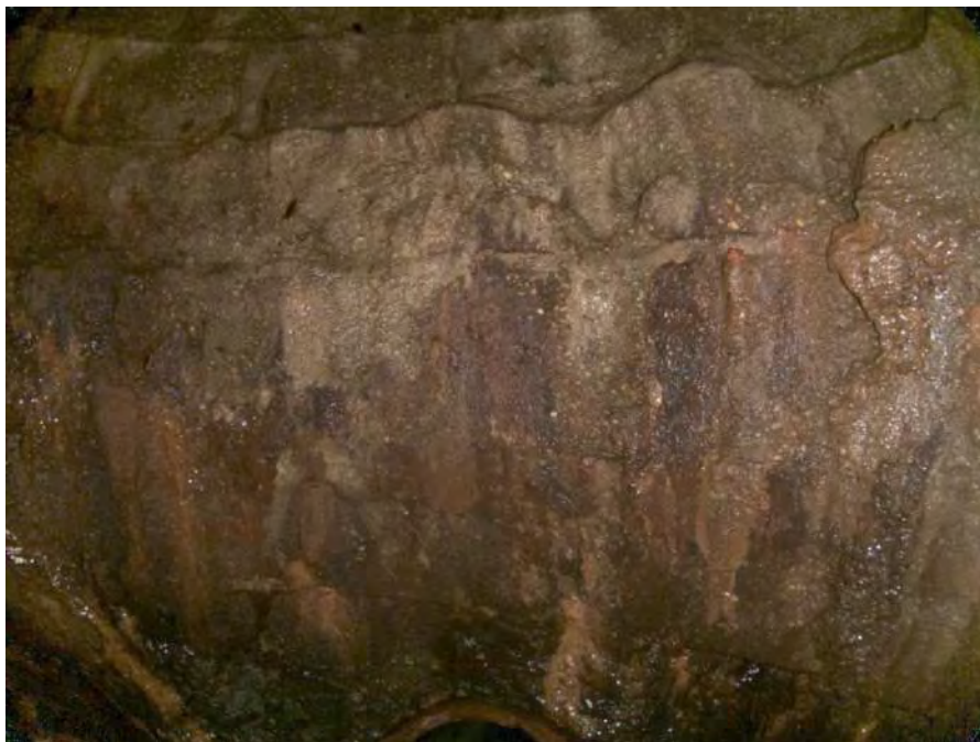
1835c_f2d6f72e-14ab-43ef-906b-8e360bc88926_b3a93ac4-f918-4e68-95ed-4a09c6c64798_P11.jpg, 00:00:29, 6.57 Infiltration Weeper from 12 o'clock to 12 o'clock, within 8 inch
