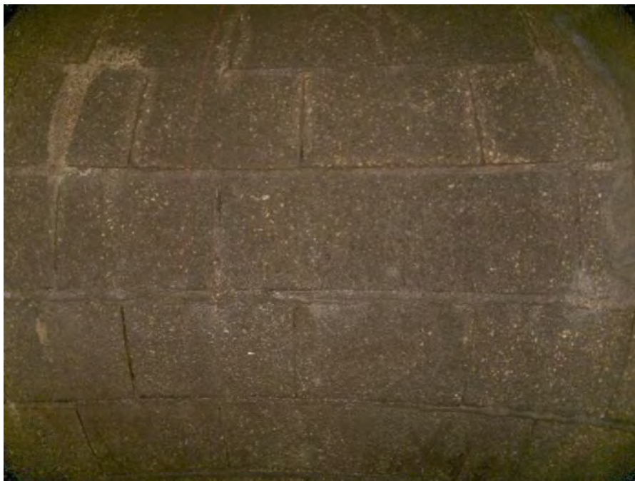
1840b_b7eec4bd-8b4a-4779-9657-5106bc04b13d_66d9a5cb-d985-4416-addd-6f90bc001a71_P11.jpg, 00:00:33, 7.78 Missing Mortar Large from 12 o'clock to 12 o'clock
