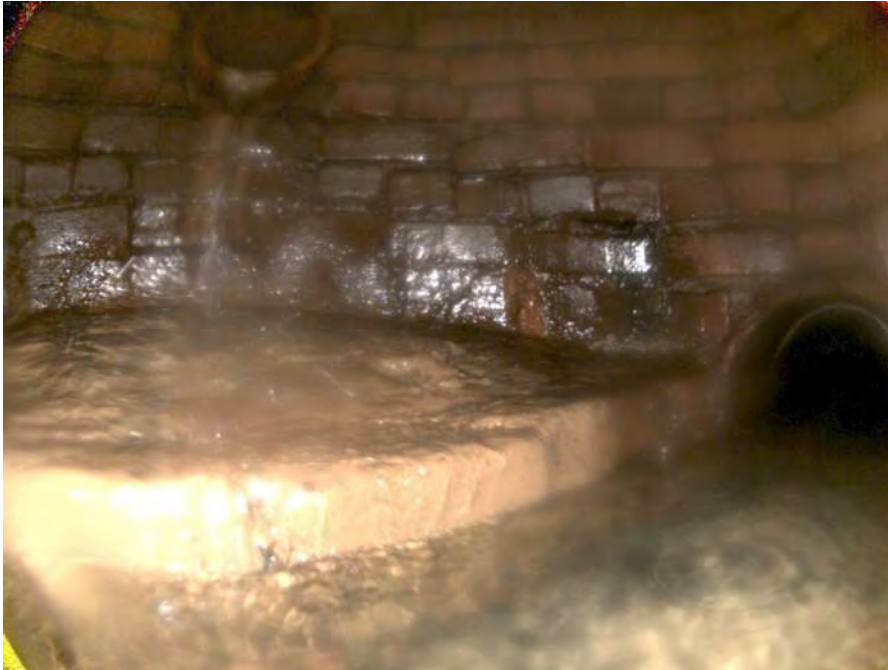
1830_f8e692ed-45a5-4111-be6d-dbb6437dd8b2_0017aeda-f63f-406e-b9a0-11021f9f5edf_PI1.jpg, 00:00:40, 8.26 Missing Mortar Large from 12 o'clock to 12 o'clock
