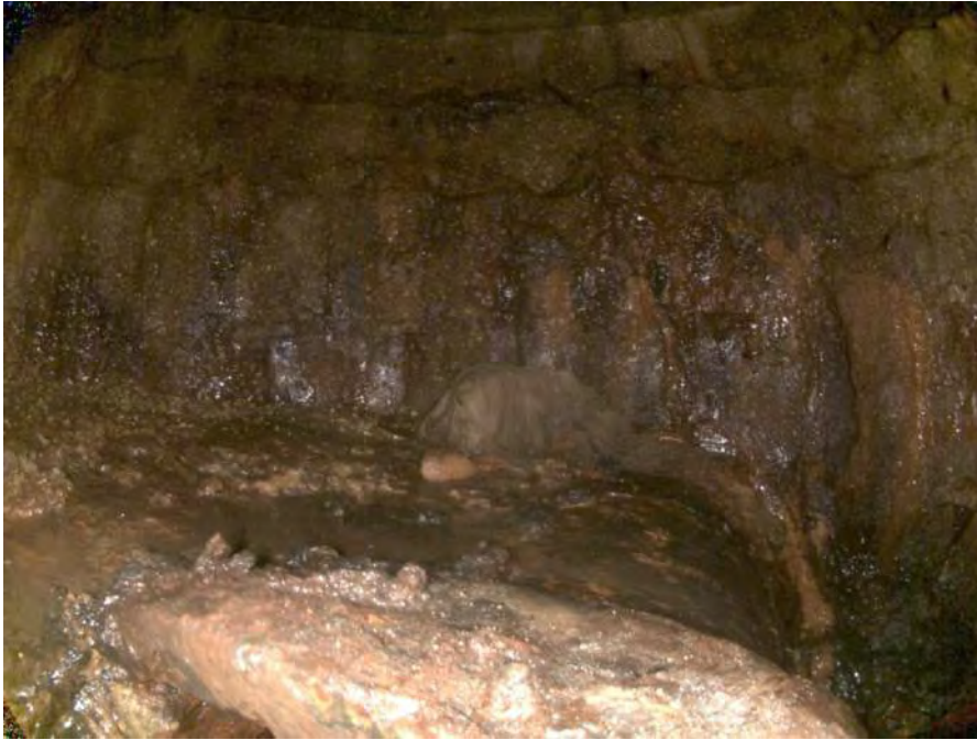
1835c_f2d6f72e-14ab-43ef-906b-8e360bc88926_591172c5-468d-4e0c-a783-9c27bbd0c414_P11.jpg, 00:00:31, 7.01 Deposits Attached Ragging, 5% of cross sectional area from 2 o'clock to 6 o'clock, within 8 inch
