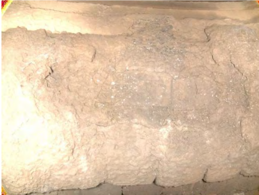
1821_b79fd861-dd10-4846-a6c3-82d3d499c9c7_15c60b1e-ee94-4fb7-ac51-8482027d4423_P11.jpg, , 0.80 Missing Mortar Large from 1 o'clock to 3 o'clock
