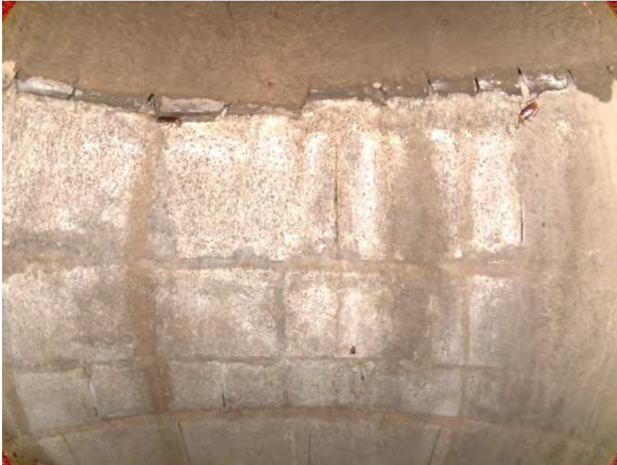
1841a_7e3e94ed-5602-4c81-88a8-bfb0bb428782_641b5ecd-14ad-4f0e-ad71-51baa60bf26d_P11.jpg, , 2.40 Infiltration Stain from 12 o'clock to 10 o'clock, within 8 inch
