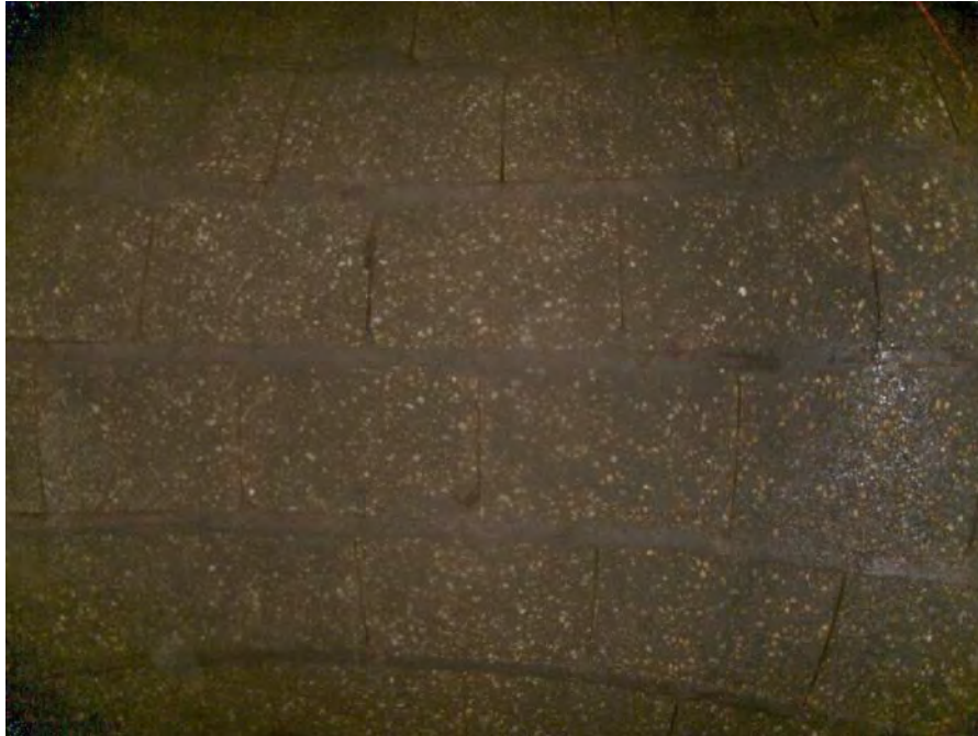
1837c_166883a2-6c9f-44dc-8d3b-993be20f6dc6_6c594d86-7c73-4195-9bc9-07d1a28f67d3_P11.jpg, 00:00:29, 6.32 Infiltration Weeper from 5 o'clock to 6 o'clock, within 8 inch
