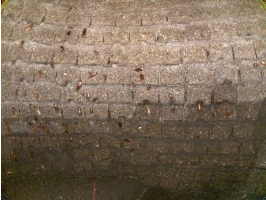
1823d_c2435bdb-6471-4a3b-8f5b-2755123d82bf_03683b8d-11dc-48d5-bed8-cf54731349bd_P11.jpg, 00:00:12, 3.34 Surface Damage Aggregate Visible from 12 o'clock to 12 o'clock, within 8 inch
