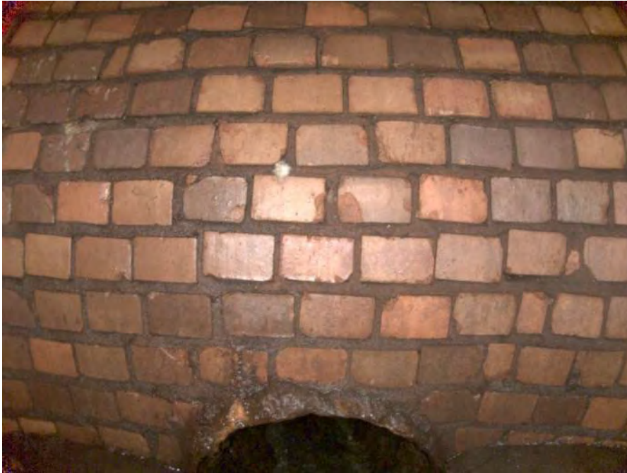
1819_3d72062a-4862-48ce-be8e-7bbe04d95bb2_9da08c23-6361-4752-b91f-34d64f0347f5_P11.jpg, 00:00:32, 7.00 Missing Mortar Large from 12 o'clock to 12 o'clock
