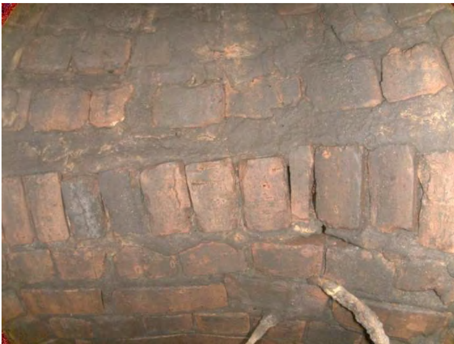
1832_5c717e28-5342-43ea-a091-aed22e190ee5_2baee998-b878-45fc-a1c0-24d43f548fb2_P11.jpg, 00:00:00, 2.84 Infiltration Stain from 11 o'clock to 5 o'clock, within 8 inch
