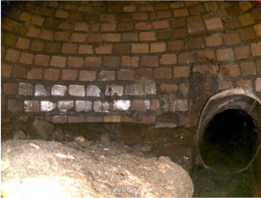
1819_3d72062a-4862-48ce-be8e-7bbe04d95bb2_bdad6f71-750a-47c5-9c9e-cf68ca13fd8e_PI1.jpg, 00:00:36, 8.57 Deposits Settled Other, 35% of cross sectional area from 9 o'clock to 3 o'clock, within 8 inch
