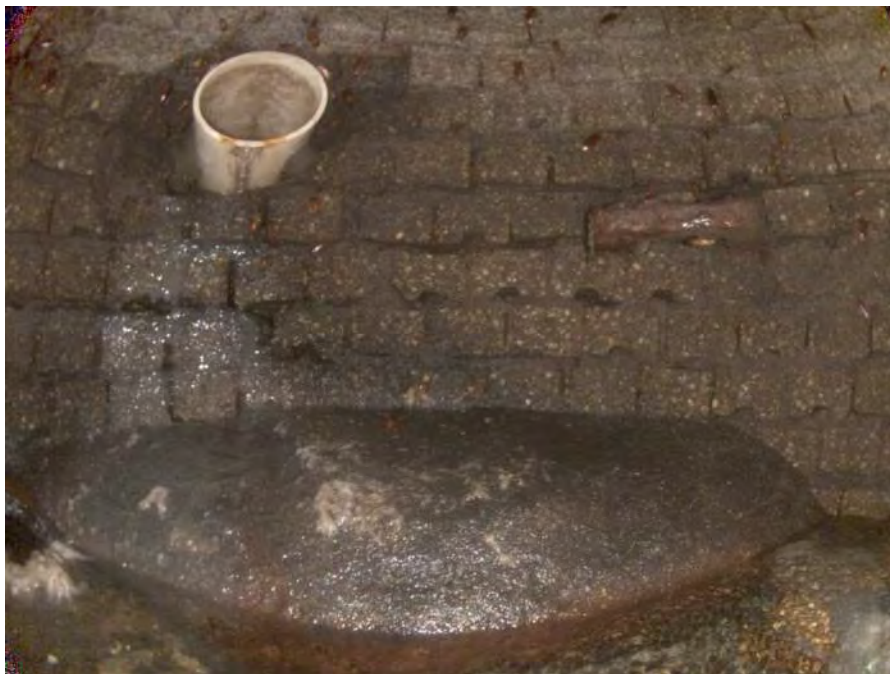
1823d_c2435bdb-6471-4a3b-8f5b-2755123d82bf_7b3163da-1179-4d08-8a3e-afb833ffb71f_P11.jpg, 00:00:15, 4.37 Deposits Settled Gravel, 15% of cross sectional area from 8 o'clock to 12 o'clock, within 8 inch
