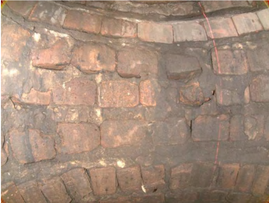
1832_5c717e28-5342-43ea-a091-aed22e190ee5_3cf15600-ec26-4327-815b-692ad98783b9_P11.jpg, 00:00:00, 1.82 Missing Mortar Large from 12 o'clock to 12 o'clock
