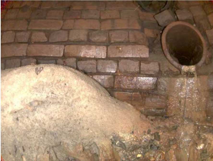
1834b_16edcb0d-7f2c-4b5a-bd27-6b0d1bf9d1bd_988d04c8-f11c-4480-860f-6154cb292fd8_P11.jpg, 00:00:32, 7.63 Infiltration Weeper from 9 o'clock to 5 o'clock, within 8 inch
