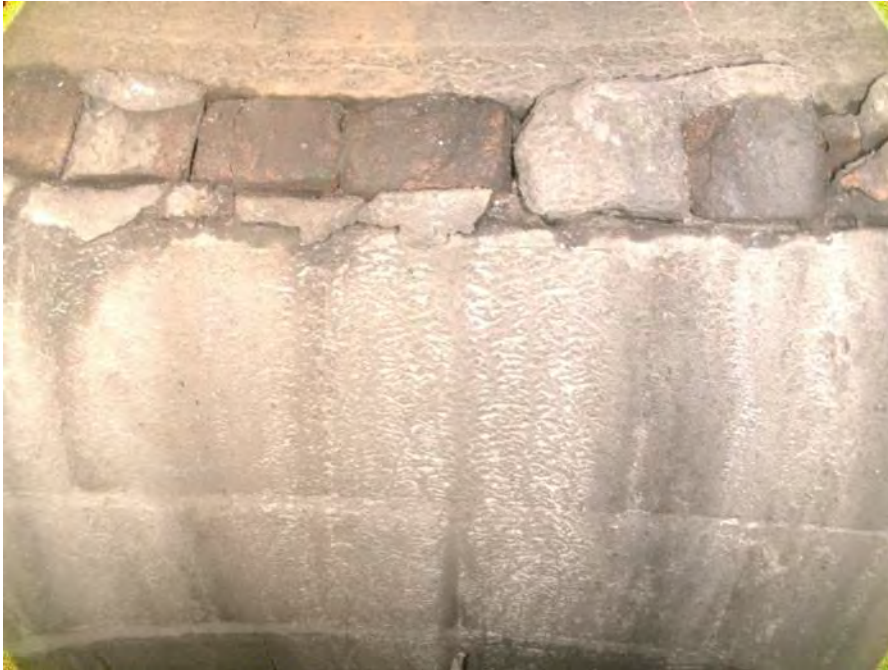
1837c_166883a2-6c9f-44dc-8d3b-993be20f6dc6_657e633f-e4e6-4faa-a090-0da65f01be06_PI1.jpg, 00:00:09, 1.12 Infiltration Stain from 12 o'clock to 12 o'clock, within 8 inch
