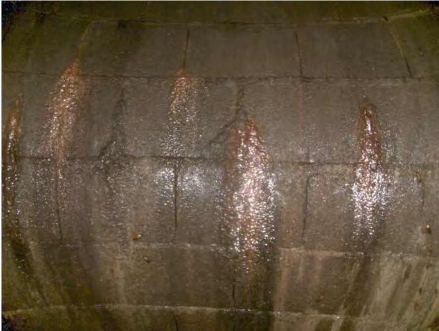
1839_f7a2e778-f07c-460d-8979-384ad1d2d1b3_ebbdf695-60e2-4b49-8316-3a0d50958fff_PI1.jpg, 00:00:31, 6.30 Infiltration Weeper from 1 o'clock to 8 o'clock, within 8 inch
