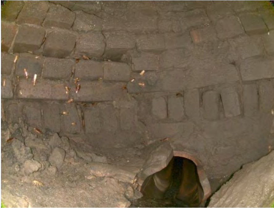
1821_b79fd861-dd10-4846-a6c3-82d3d499c9c7_b7cfa781-f78c-4dad-bb28-9ce6c40f33d1_PI1.jpg, 00:00:16, 3.04 Missing Mortar Large from 12 o'clock to 12 o'clock
