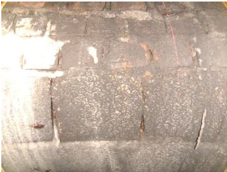
1838_4d464b94-a957-4557-a7ae-8bb14bf4d783_e2af839c-408d-41e6-99c2-131845b5d5b6_P11.jpg, , 1.51 Infiltration Stain from 12 o'clock to 12 o'clock, within 8 inch
