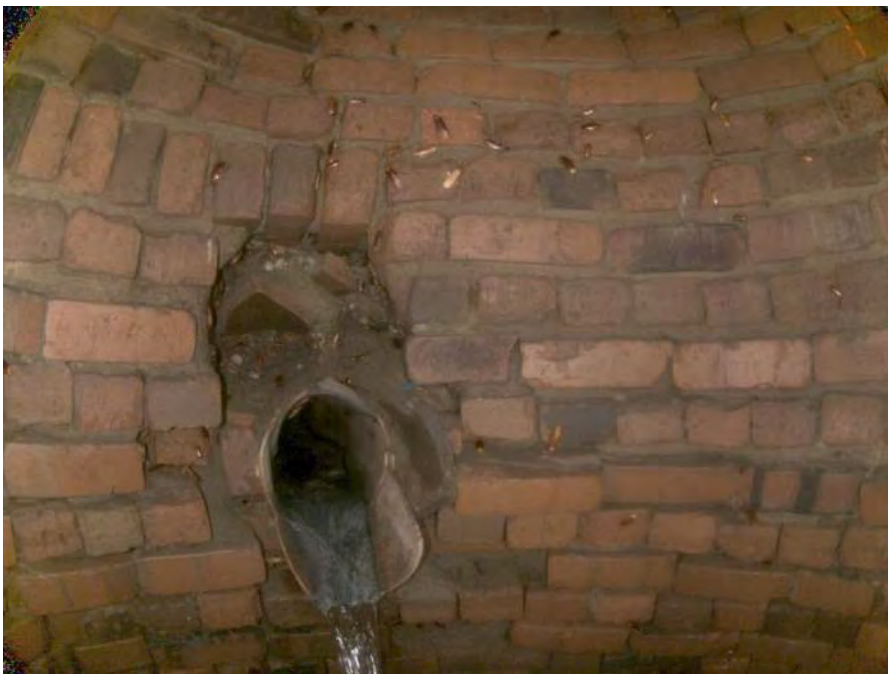
1829b_c3bb5419-4fc2-49bd-9cbb-ae8a522c6251_529420aa-6db1-47bc-8ee3-9da21fb0b2d7_P11.jpg, 00:00:32, 7.57 Hole Void Visible from 2 o'clock to 4 o'clock, within 8 inch
