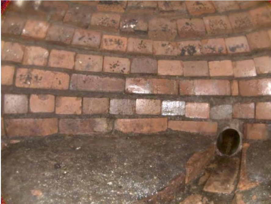
2193c_2b27c63e-1844-43c6-8c49-44849fa40c9a_f01e8115-6d9e-48aa-8948-beff3c204241_P11.jpg, 00:00:17, 3.06 Infiltration Weeper from 11 o'clock to 3 o'clock, within 8 inch
