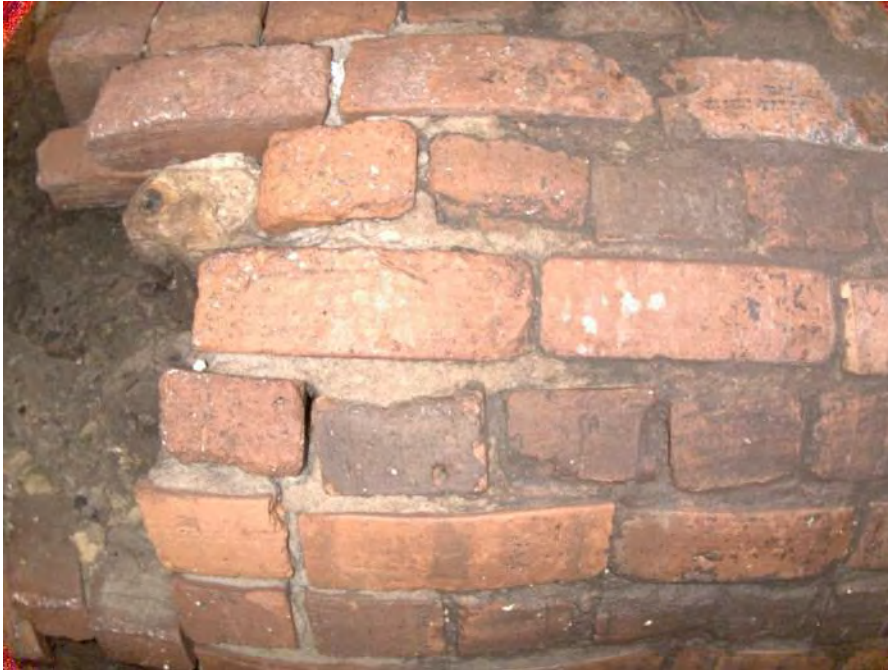
1828b_5154b3dc-7153-4625-bad4-be8d5b792f69_3173cf7b-f6db-4944-a0d7-c17632622fc9_P11.jpg, 00:00:33, 6.91 Broken Soil Visible, 18inch defective, 18inch intrusion at 1 o'clock, within 8 inch, Start
