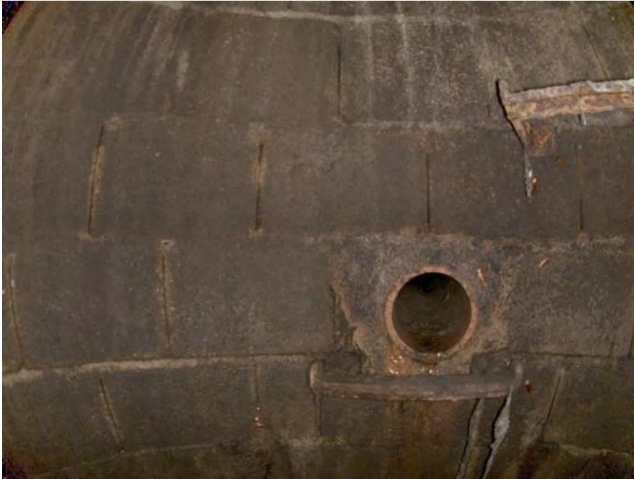
1839_f7a2e778-f07c-460d-8979-384ad1d2d1b3_26e11d77-b5b6-47cb-ba13-ce6b8078be20_P11.jpg, 00:00:22, 4.10 Deposits Attached Ragging, 5% of cross sectional area from 8 o'clock to 12 o'clock, within 8 inch
