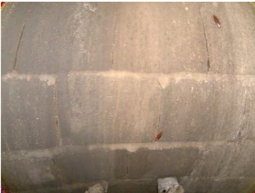
1842_98b1de5e-0e50-41ed-b476-ff581fdb636e_aa2a85a8-e416-49a8-9ee1-a1520a8a9a6f_PI1.jpg, 00:00:17, 2.39 Infiltration Stain from 8 o'clock to 5 o'clock, within 8 inch
