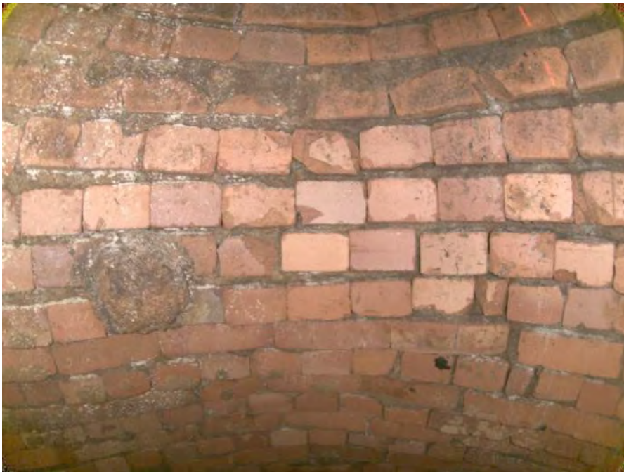
1833a_415896af-f5e7-4861-970c-902a07ead962_4fdf478f-d238-4325-aa4c-e1c799d57fa0_P11.jpg, 00:00:19, 3.55 Missing Mortar Large from 12 o'clock to 12 o'clock
