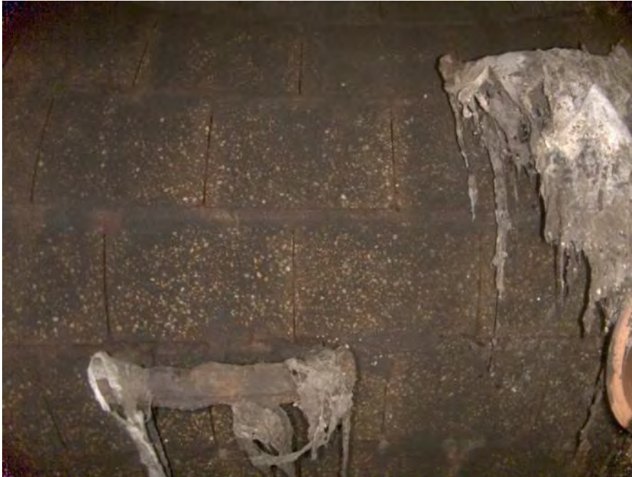
1837c_166883a2-6c9f-44dc-8d3b-993be20f6dc6_9705dbdb-6ee7-4b05-98c9-4de012303572_P11.jpg, 00:00:23, 5.04 Deposits Attached Ragging, 5% of cross sectional area from 7 o'clock to 10 o'clock, within 8 inch
