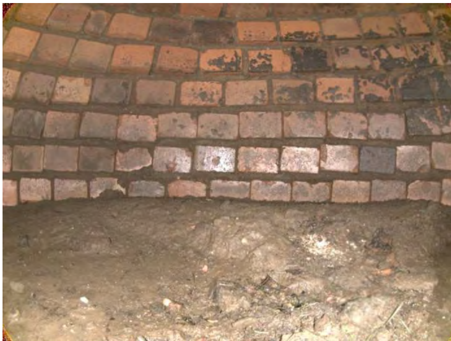
2194_1962243a-d72d-4c62-9e3a-2c87a26c1c57_80c86366-c9e9-43ae-8397-d26630ffeced_P11.jpg, 00:00:20, 3.69 Deposits Settled Gravel, 30% of cross sectional area from 9 o'clock to 2 o'clock, within 8 inch
