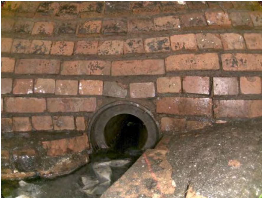
2193c_2b27c63e-1844-43c6-8c49-44849fa40c9a_64fc95ca-fdb3-46c0-8178-6593d18247cb_P11.jpg, 00:00:17, 3.83 Missing Mortar Medium from 12 o'clock to 12 o'clock
