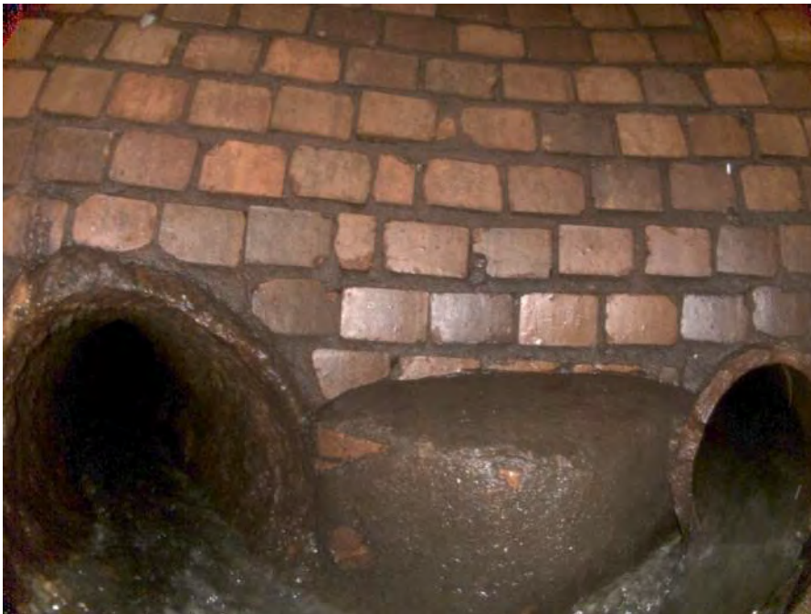
1819_3d72062a-4862-48ce-be8e-7bbe04d95bb2_f70a0414-0ff6-4f34-b025-c17650aa6690_PI1.jpg, 00:00:36, 8.64 Missing Mortar Small from 3 o'clock to 9 o'clock
