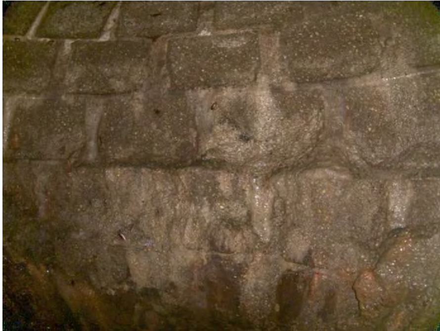
1835c_f2d6f72e-14ab-43ef-906b-8e360bc88926_f8f971ba-6780-4a33-823f-3022d1b31921_P11.jpg, 00:00:25, 5.46 Missing Mortar Large from 12 o'clock to 12 o'clock
