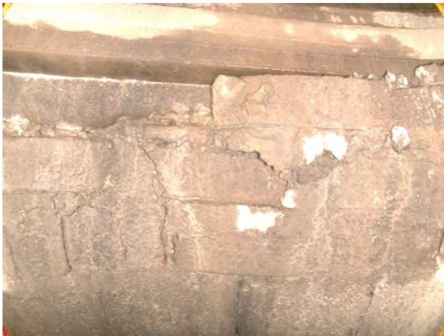
1839_f7a2e778-f07c-460d-8979-384ad1d2d1b3_f10eed2a-ba9a-477d-b689-5f09c7740fe1_P11.jpg, , 0.99 Missing Mortar Large from 12 o'clock to 12 o'clock
