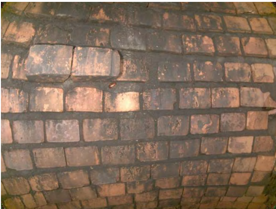
1818_a75925b2-5868-48ca-b1fe-f6e00ecc4562_f686146f-7c19-45e6-84c8-ca697ba48ffe_P11.jpg, 00:00:19, 4.21 Missing Mortar Large from 12 o'clock to 12 o'clock
