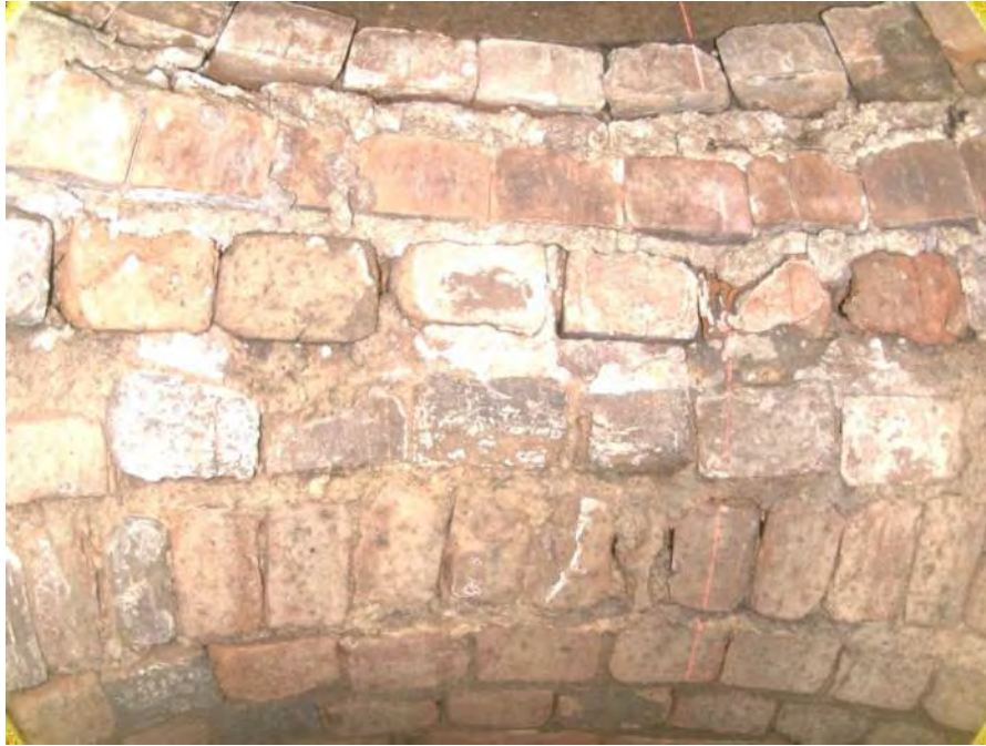
1834b_16edcb0d-7f2c-4b5a-bd27-6b0d1bf9d1bd_3d5f165f-06b8-4857-8369-535a926f5c84_P11.jpg, , 1.48 Missing Mortar Large from 12 o'clock to 12 o'clock
