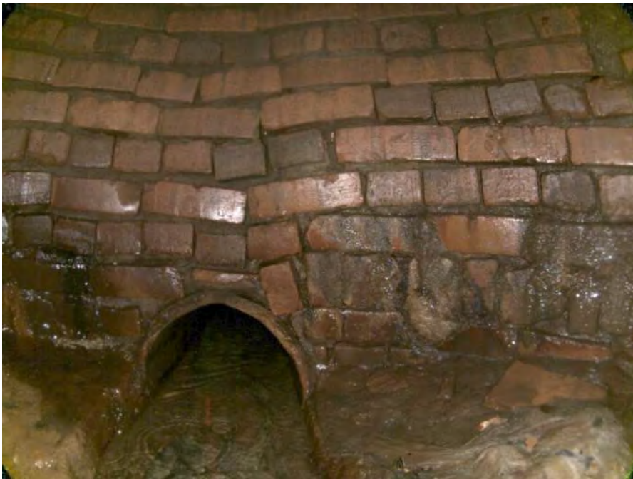
1830_f8e692ed-45a5-4111-be6d-dbb6437dd8b2_e7ceb1d1-5301-4ee2-b6a3-deb392ea1197_P11.jpg, 00:00:38, 7.93 Displaced Brick from 5 o'clock to 7 o'clock
