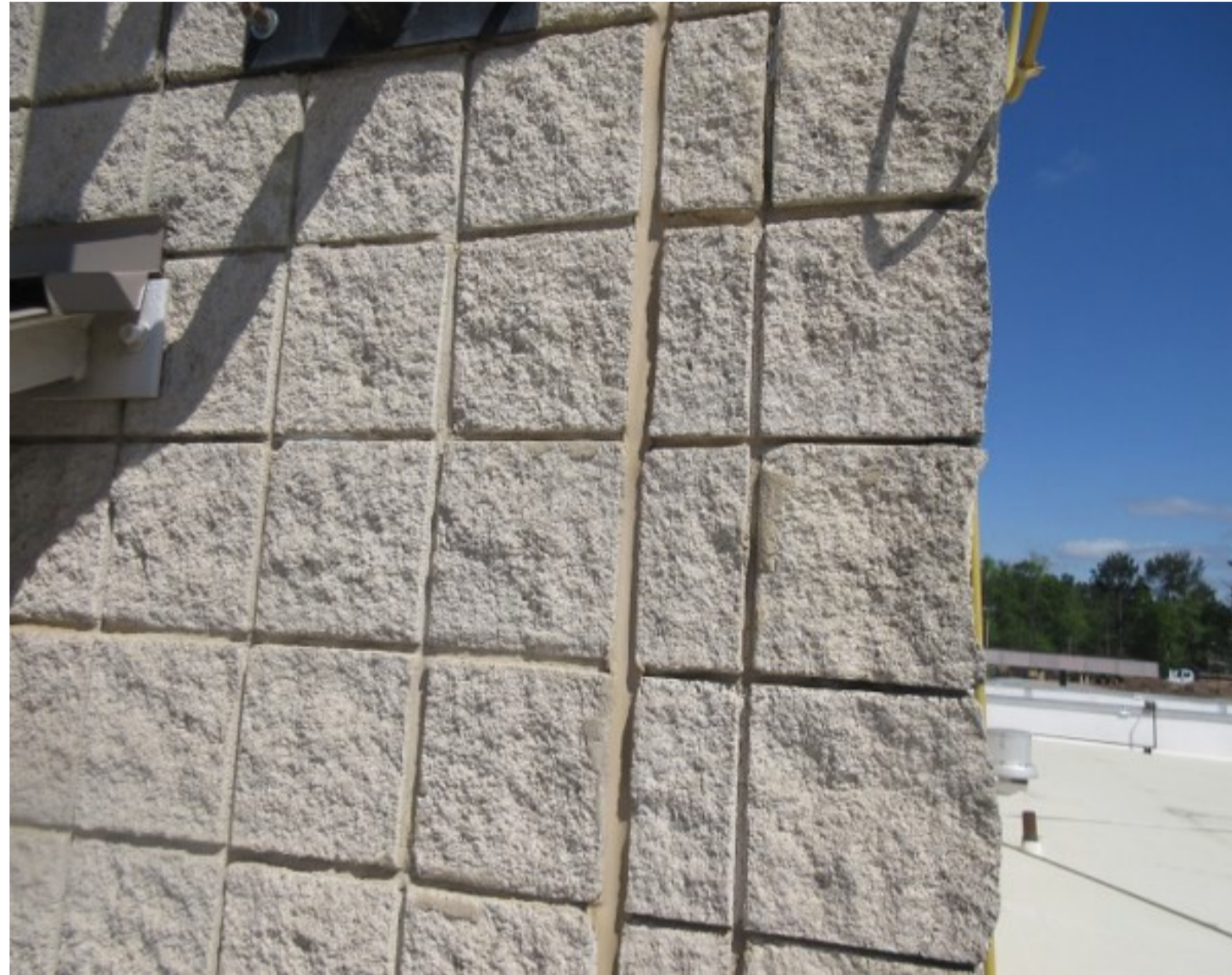
Expansion joints and control joints are to be replaced with new high performance sealant joints before the elastomeric coating is applied.
