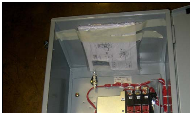
Figure 21. Wire Securely Installed in the Terminal Block.
