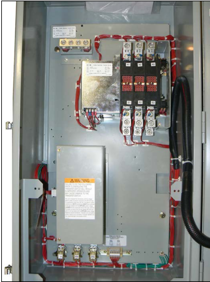
Figure 8. Typical Power Panel for 40-400A Open Transition ATS.
