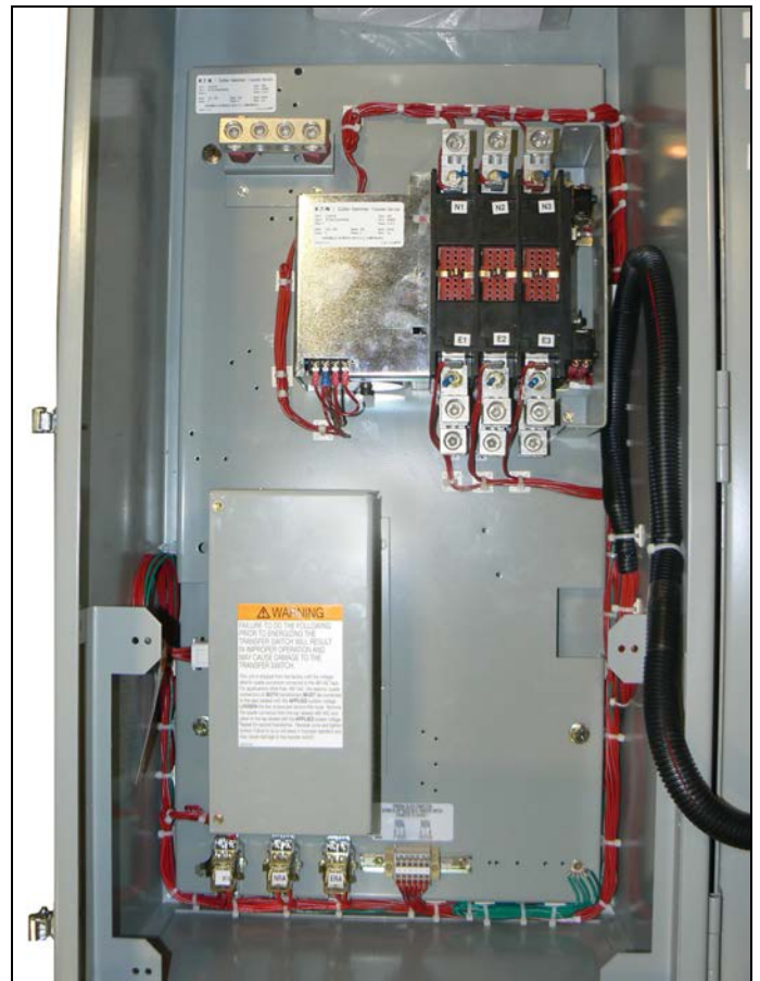
Figure 3. Typical Power Panel for a 100A Open Transition ATS.
