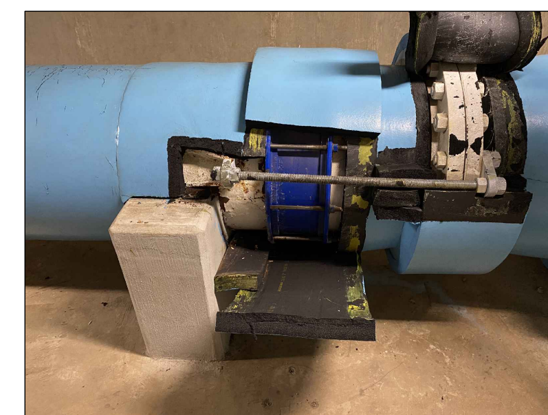
PHOTO OF EXISTING FINISHED WATER HEADER IN PUMP GALLERY
