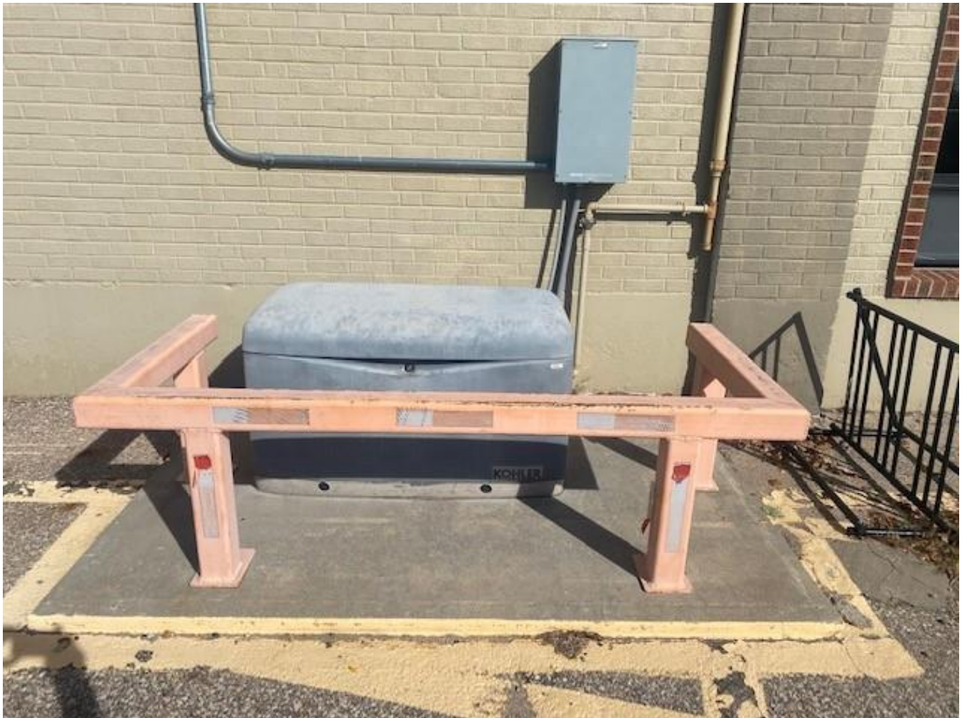
Existing Kohler Generator
