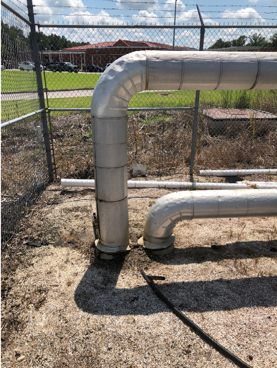
Condenser Water Piping from Mechanical Room
