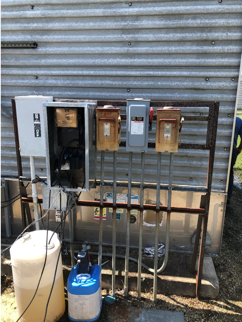
Makeup water for tower and electrical power source
