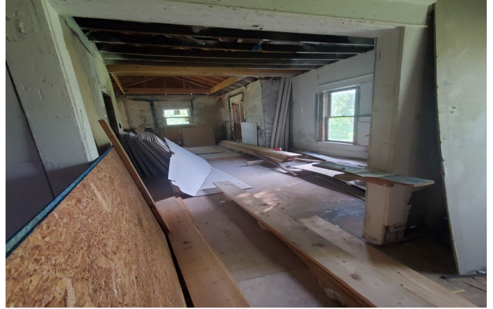
Photo 8 – Stacks of unfinished drywall located sporadically throughout.
