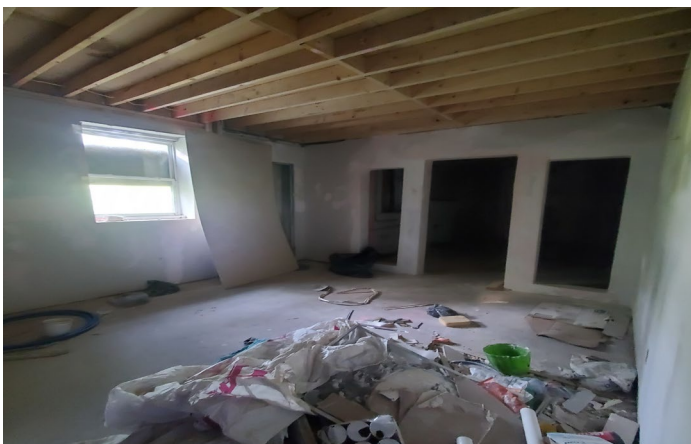
Photo 5 – New drywall added to basement since initial assessment. View of sampling area.
