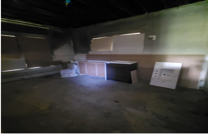
Photo 7 – Newly added wood flooring. Building material stored on main level of residence.
