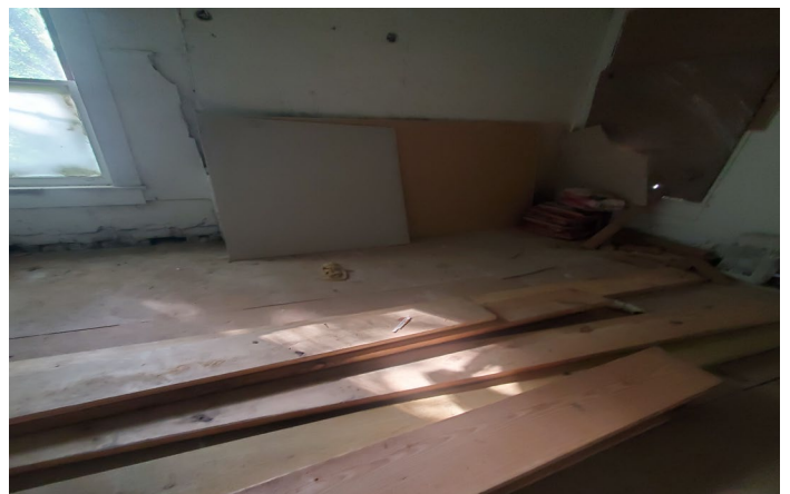
Photo 6 – Typical view of wood flooring stored throughout main level. New subflooring has been added.
