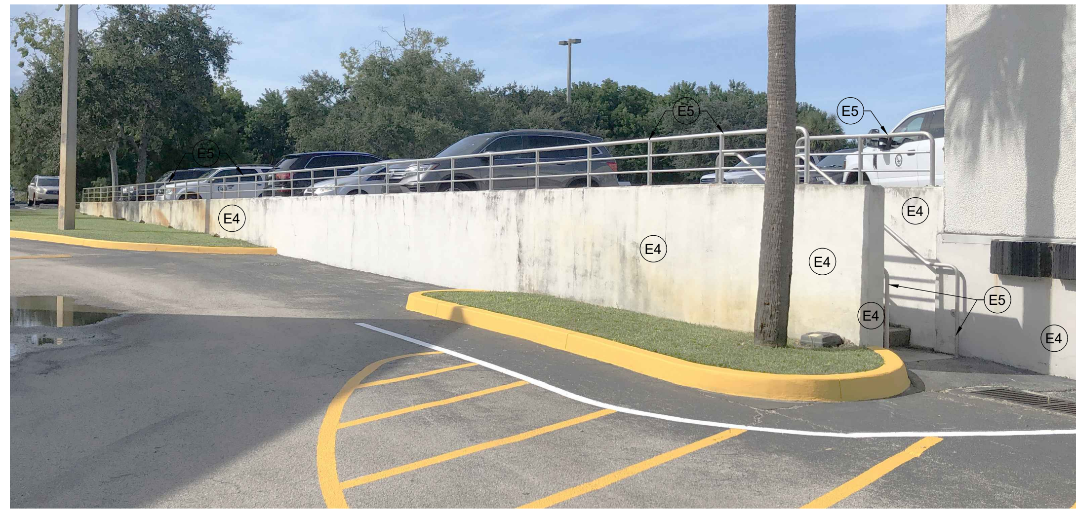
06 RETAINING WALL B TYPICAL FOR ALL EXPOSED SIDES OF RETAINING WALL SCALE: NTS
