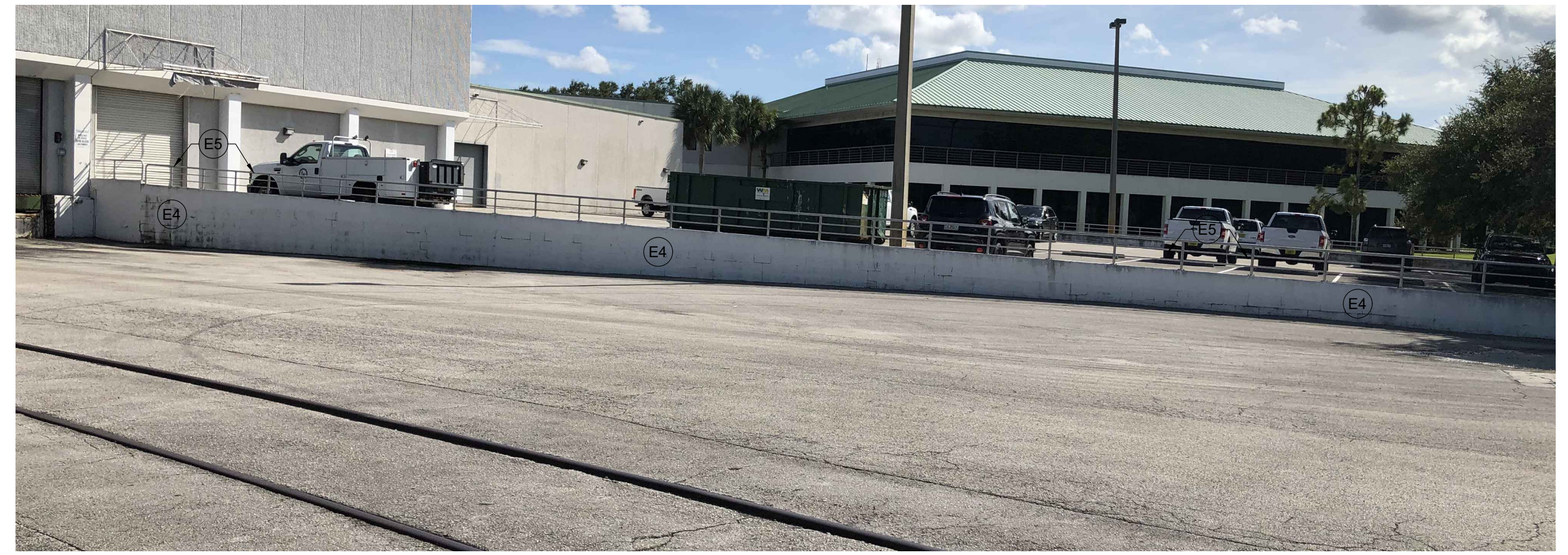
05 RETAINING WALL A TYPICAL FOR ALL EXPOSED SIDES OF RETAINING WALL SCALE: NTS
