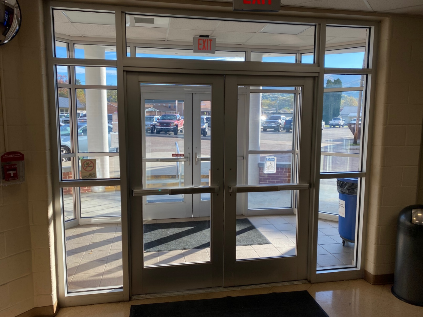
(Item 1) Interior view of the current doors (both sets) is shown below.
