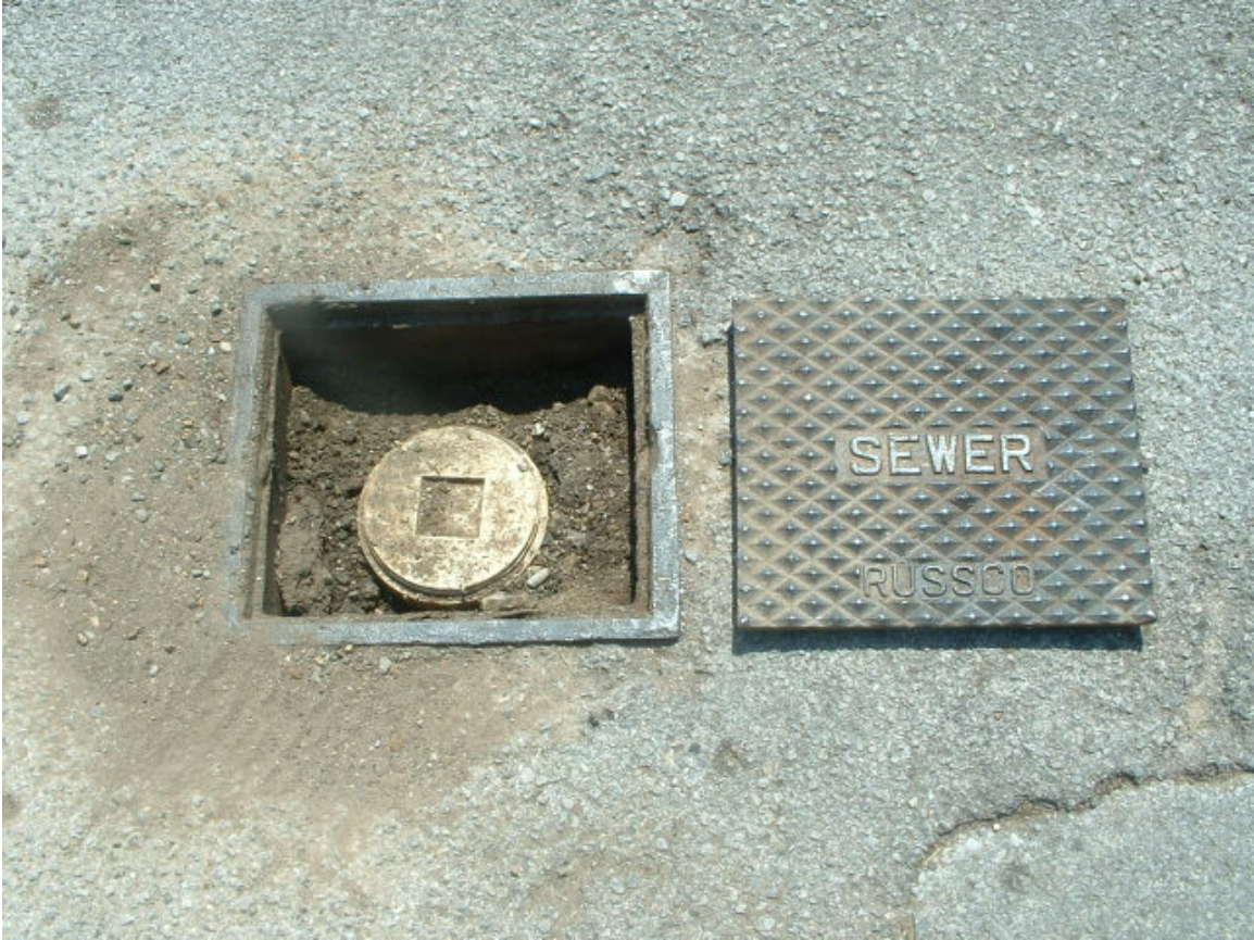
TYPICAL EXAMPLE PHOTOGRAPH OF A CAST IRON SEWER CLEAN-OUT BOX
