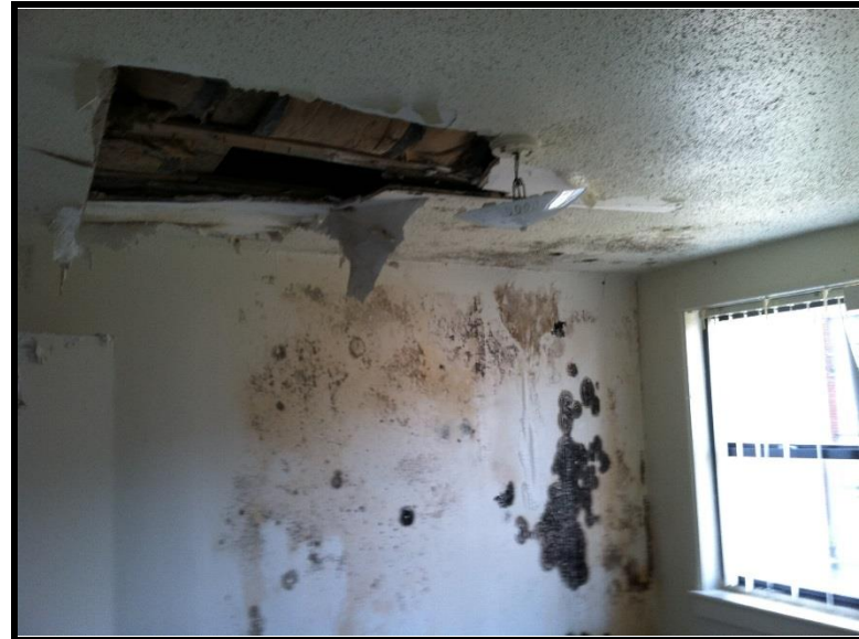
10 General view of unit 343 damaged 2 nd floor ceiling
