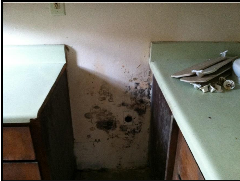
9 Mold located on unit 343 – drywall wall Sample S1
