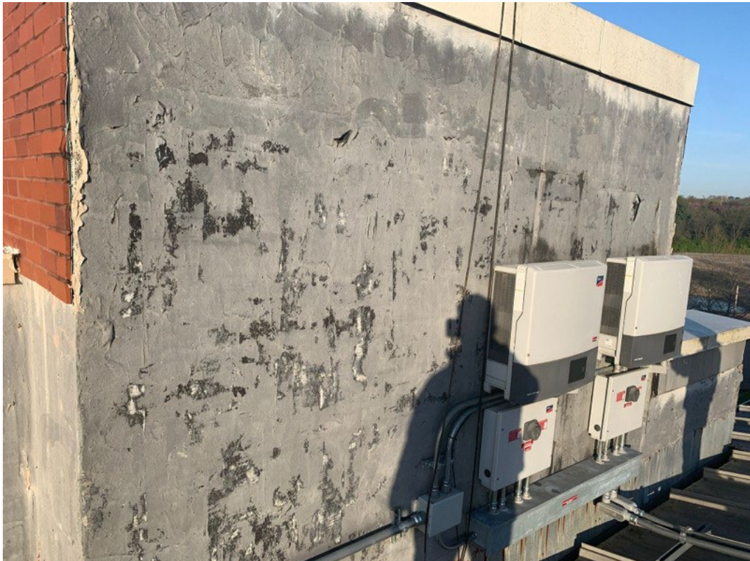
Solar Panel Control Boxes
