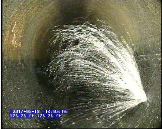
G270 G272_d3e0174d-46f3-4bf9-8d25-161e05baba4b.bmp, 00:03:55, 176.80 Infiltration Gusher, at 4 o'clock
