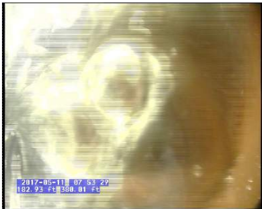
G160 G161_3c4c3644-cfe2-4fd1-ad6b-c565f6a13c6c.bmp, 00:06:31, 182.97 Tap Break-In, at 9 o'clock, 4 inch dim
