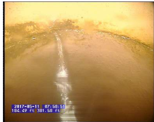
G160 G161_01c89cc4-169b-4891-8b8c-66de64491820.bmp, 00:08:17, 184.55 Infiltration Runner, at 12 o'clock
