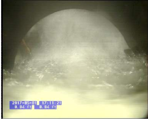
P36 P74_fdd61753-f9be-410f-844d-23e9d200c77e.bmp, NaN:NaN:, 1.02 Survey Abandoned, offset joint
