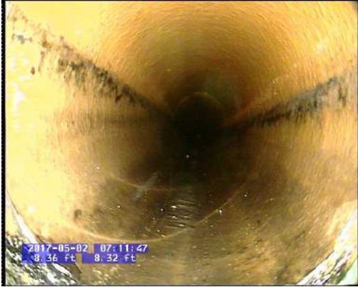
P37 P36_2b950ddc-6a67-4b33-93b8-4f85cf56f1a3.bmp, 00:00:17, 8.37 Material Change, Vitrified clay pipe
