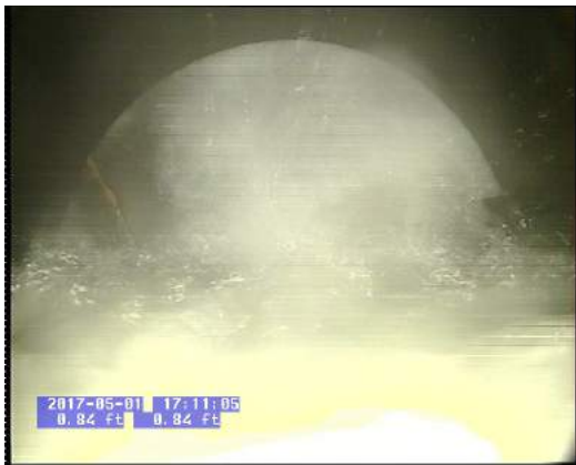
P36 P74_db4e454f-3ba2-473e-9445-4154ee93850e.bmp, NaN:NaN:, 1.02 Survey Abandoned, offset joint
