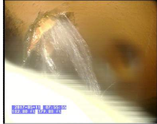
G160 G161_c0caf2a2-9e76-4e62-adbb-02af314ea669.bmp, 00:07:39, 182.84 Infiltration Gusher, at 9 o'clock
