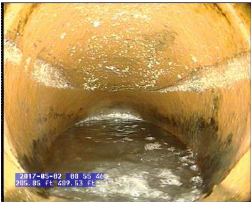
P86 P36_ca8557df-ae5b-47e3-97c0-49cc43cfcda.bmp, 00:05:47, 285.93 Survey Abandoned
