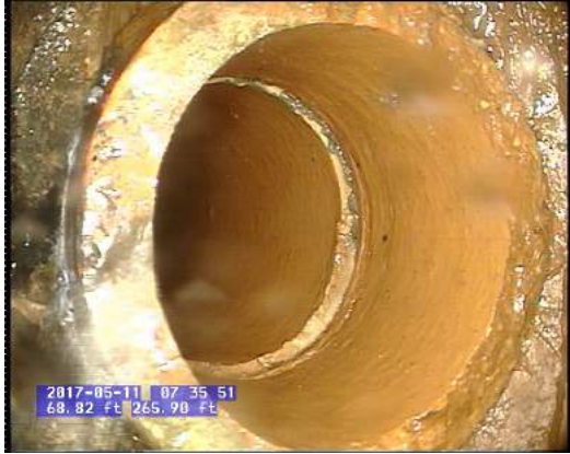
G160 G161_48d84a4b-2377-4ee4-9a3f-ed6f8c312317.bmp, 00:02:08, 68.83 Tap Break-In, at 9 o'clock, 4 inch dim
