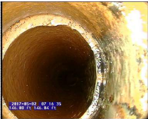
P37 P36_739d1293-6cb2-4798-b2ef-a10506e25cc0.bmp, 00:04:31, 146.13 Tap Factory Made Active, at 3 o'clock, 4 inch dim
