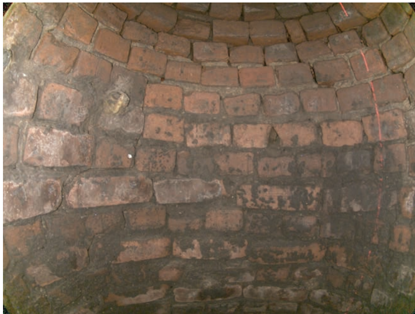
1828b_5154b3dc-7153-4625-bad4-be8d5b792f69_af14e9ce-43e7-4d78-b89c-bf5f5b97d8ee_P11.jpg, , 3.02 Missing Mortar Large from 12 o'clock to 12 o'clock
