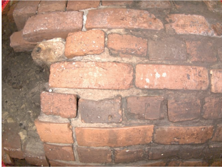
1828b_5154b3dc-7153-4625-bad4-be8d5b792f69_3173cf7b-f6db-4944-a0d7-c17632622fc9_P11.jpg, 00:00:33, 6.91 Broken Soil Visible, 18inch defective, 18inch intrusion at 1 o'clock, within 8 inch, Start
