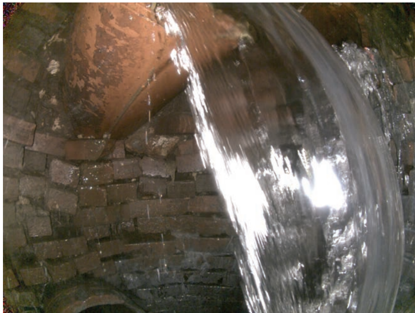
1828b_5154b3dc-7153-4625-bad4-be8d5b792f69_a9eef5b8-2357-475d-a879-3b8cd9676573_P11.jpg, 00:00:39, 8.18 Displaced Brick from 8 o'clock to 11 o'clock
