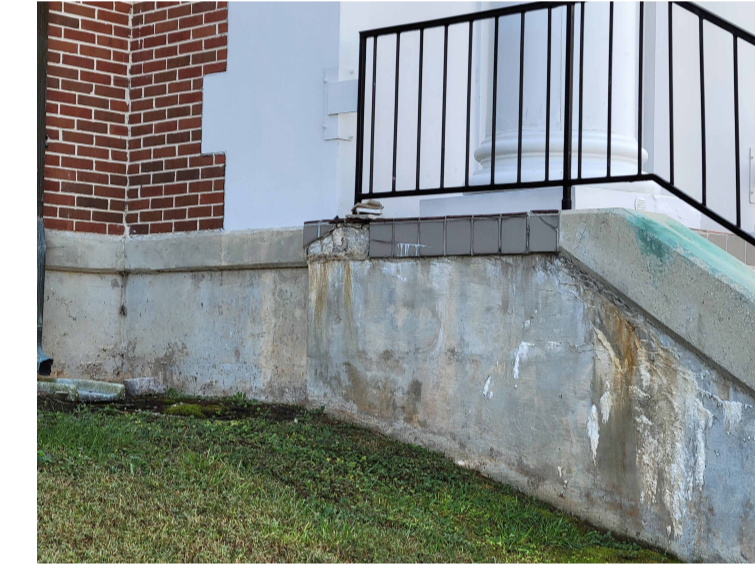
CONDITION 10: TILE AT STAIRS DAMAGED AND STAINED
