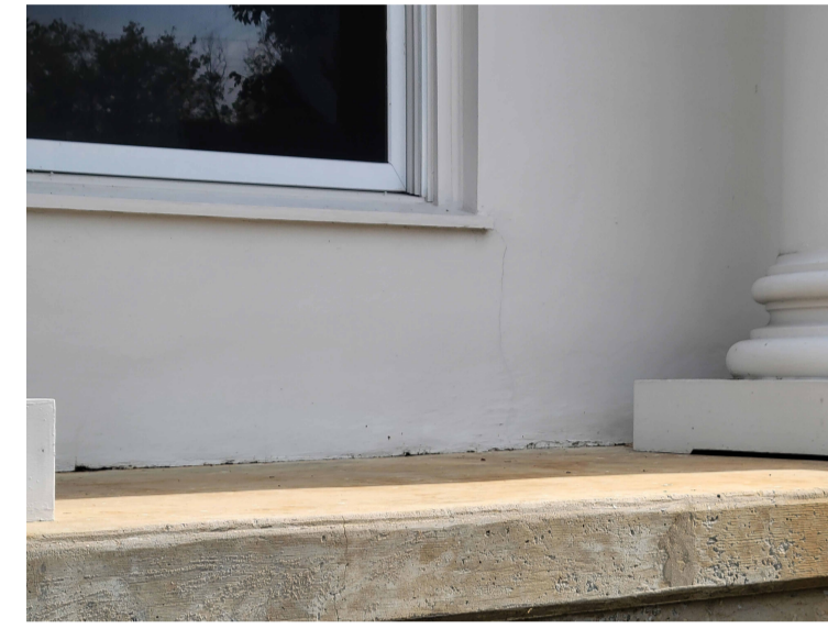
CONDITION 07: WALL BASE CRACKED WITH GAPS
