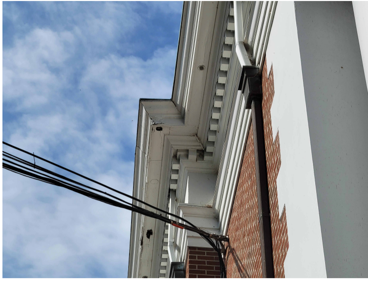
CONDITION 01: SPLIT AND DAMAGED SOFFITS AND CORNICE
