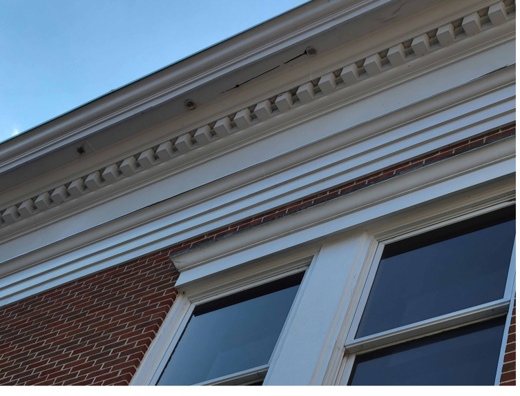
CONDITION 01: SPLIT AND DAMAGED SOFFITS AND CORNICE
