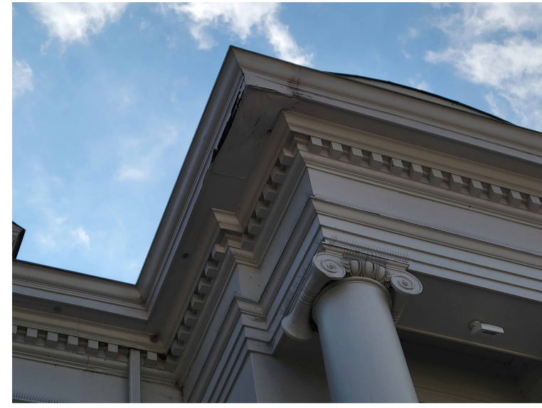
CONDITION 01: SPLIT AND DAMAGED SOFFITS AND CORNICE
