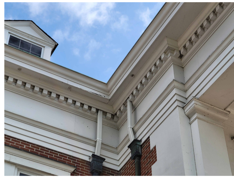
CONDITION 01: SPLIT AND DAMAGED SOFFITS AND CORNICE
