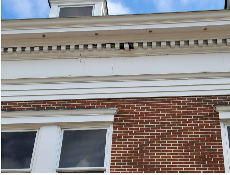
CONDITION 01: SPLIT AND DAMAGED SOFFITS AND CORNICE
