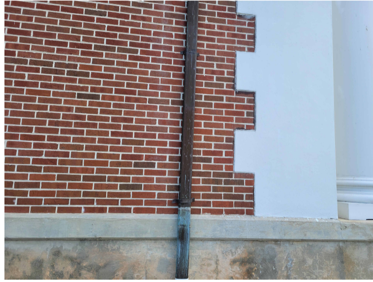
CONDITION 04: DECORATIVE PLASTER TO BRICK STAINED
