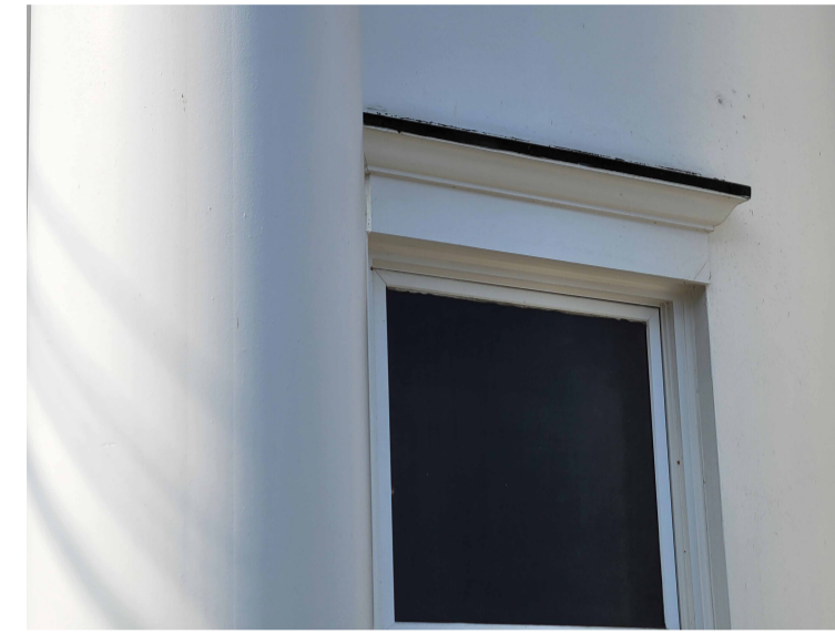
CONDITION 05: WINDOW HEAD CRACKED
