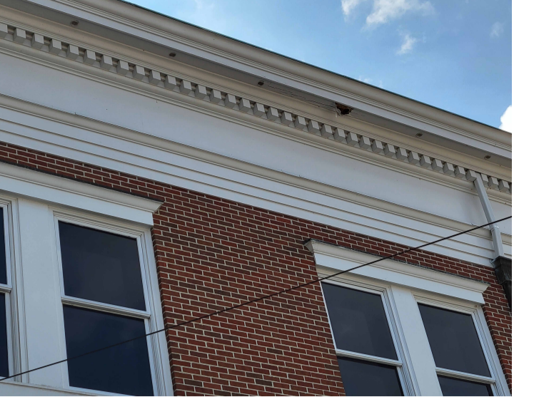
CONDITION 01: SPLIT AND DAMAGED SOFFITS AND CORNICE
