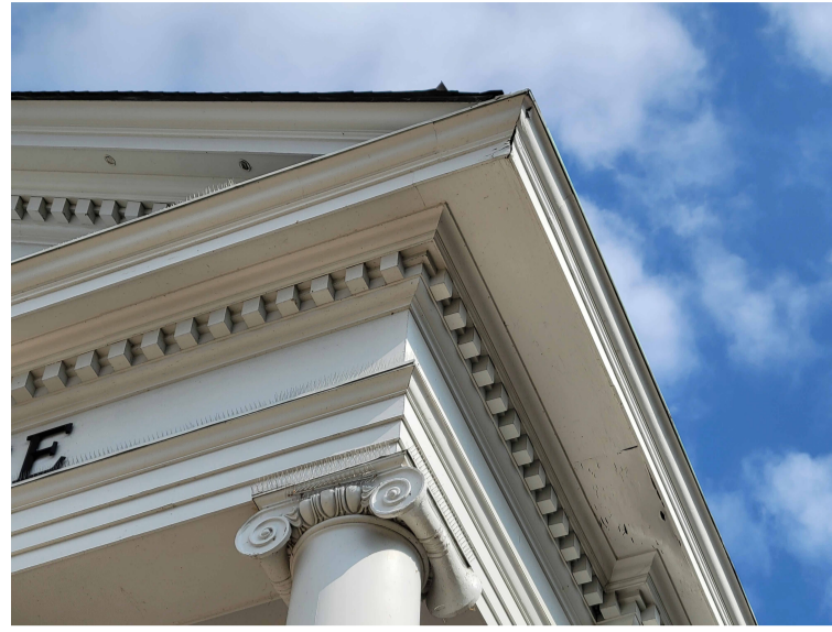
CONDITION 01: SPLIT AND DAMAGED SOFFITS AND CORNICE
