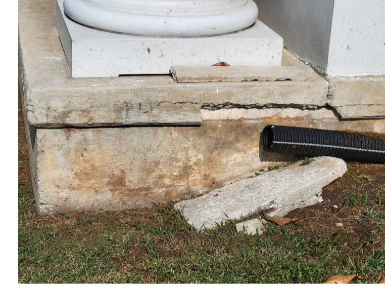
CONDITION 09: CONCRETE EDGES CRACKED AND STAINED
