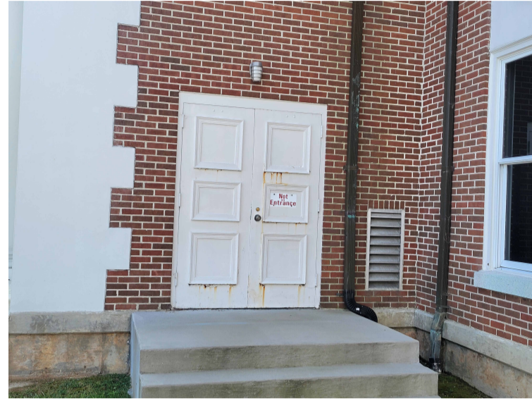
CONDITION 03: STAINED EXTERIOR DOORS
