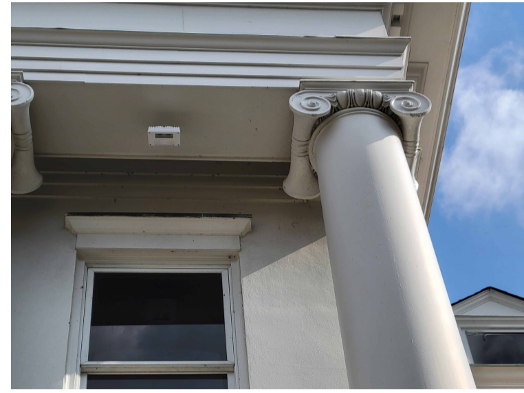
CONDITION 02: COLUMN CAPITAL NEEDS REPAINT
