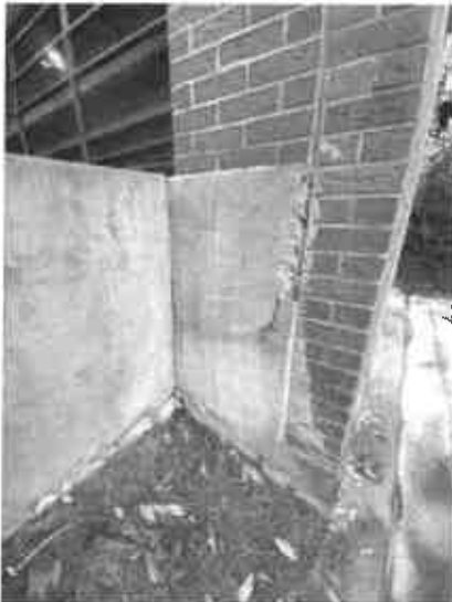
PHOTO 55: CRACK THROUGH EXTERIOR BRICK VENEER
