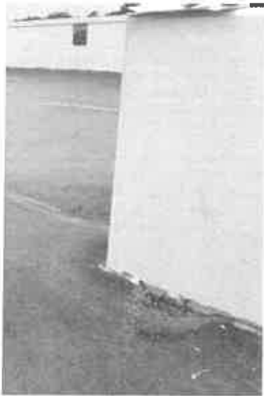
PHOTO 9: CONCRETE TOPPING DAMAGE AT UPPER LEVEL
