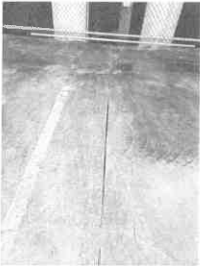
PHOTO 7: TOPPING SLAB JOINT AT UPPER LEVEL DECK
