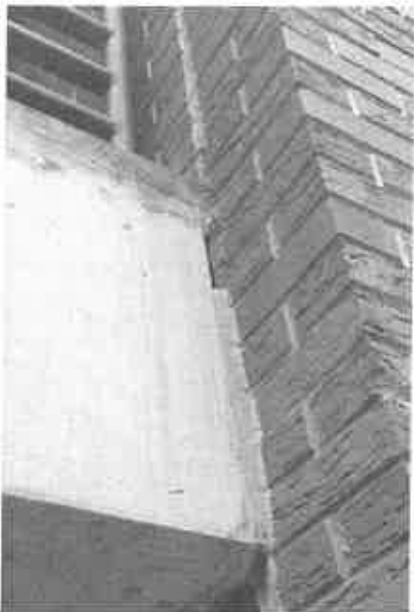
PHOTO 27: MISSING CAULK AT THE WALL PANEL AND BEAM JOINT
