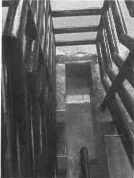
PHOTO 22: RAINWATER RUNOFF BETWEEN STAIR FLIGHTS
