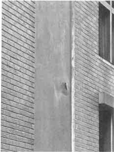
PHOTO 20: ISOLATED SPALLING ON EAST WALL
