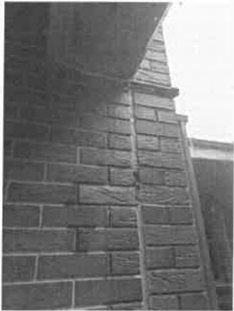
PHOTO 26: DETERIORATED CAULK IN WALL PANEL JOINTS
