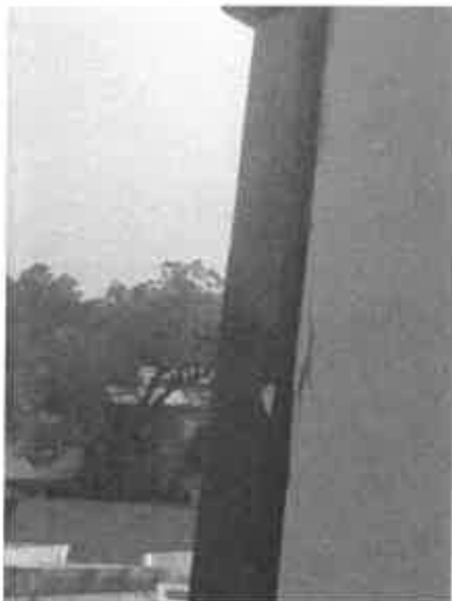
PHOTO 40: SPALLED CONCRETE COVER OVER PANEL JOINT
