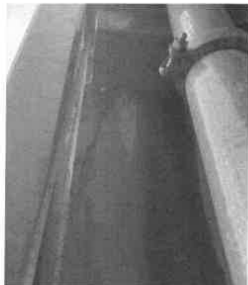
PHOTO 41: SPALLED CONCRETE COVER OVER PANEL JOINT BELOW UPPER LANDING
