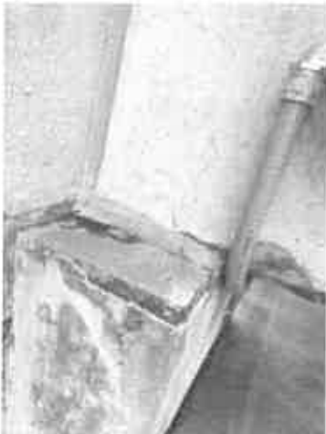
PHOTO 19: CORRODED BEAM BEARING PLATE
