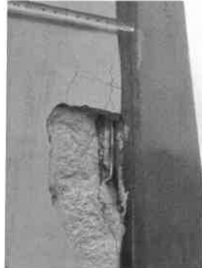
PHOTO 39: CLOSE UP OF SPALLED CONCRETE AND CORRODED REINFORCING
