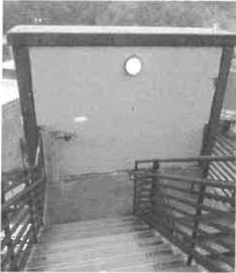
PHOTO 38: SPALLED CONCRETE COVER OVER PANEL JOINT
