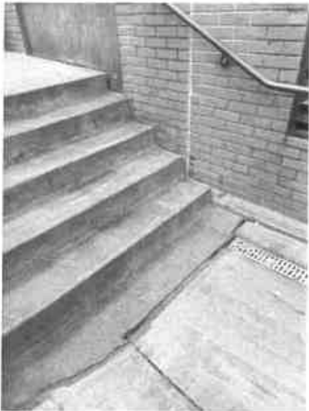
PHOTO 28: DAMAGED BRICK VENEER
