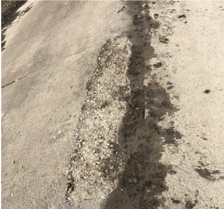
Figure 11 – Signs of Spalling
