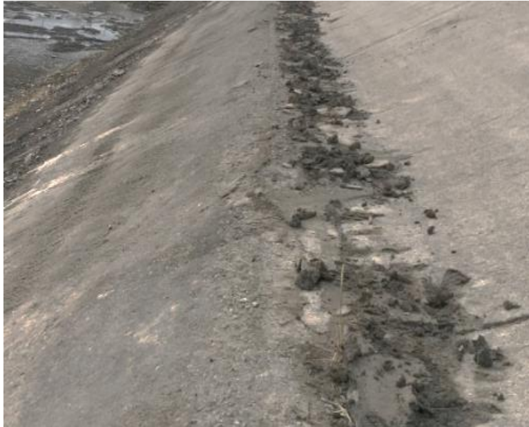
Figure 7 – Signs of Spalling
