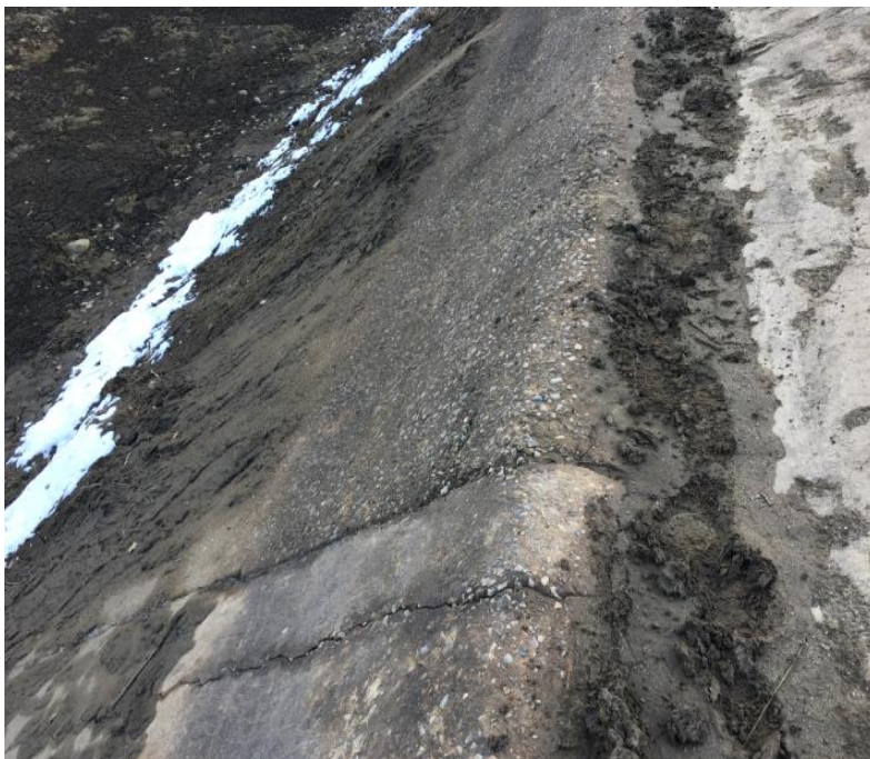
Figure 12 – Signs of Spalling and Longitudinal Crack
