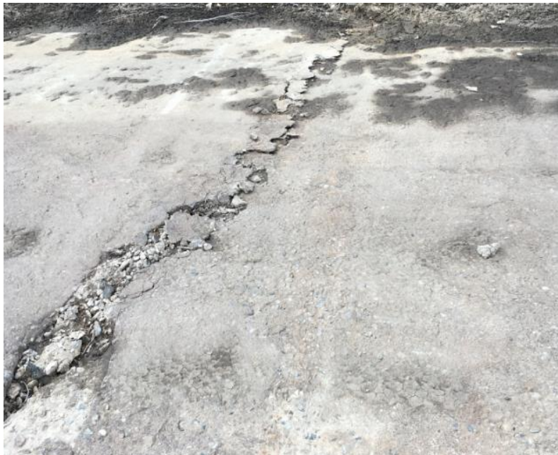
Figure 10 – Longitudinal Crack with Delamination
