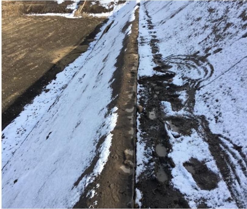
Figure 15 – Lower Lining Bulging Out (Sideview)
