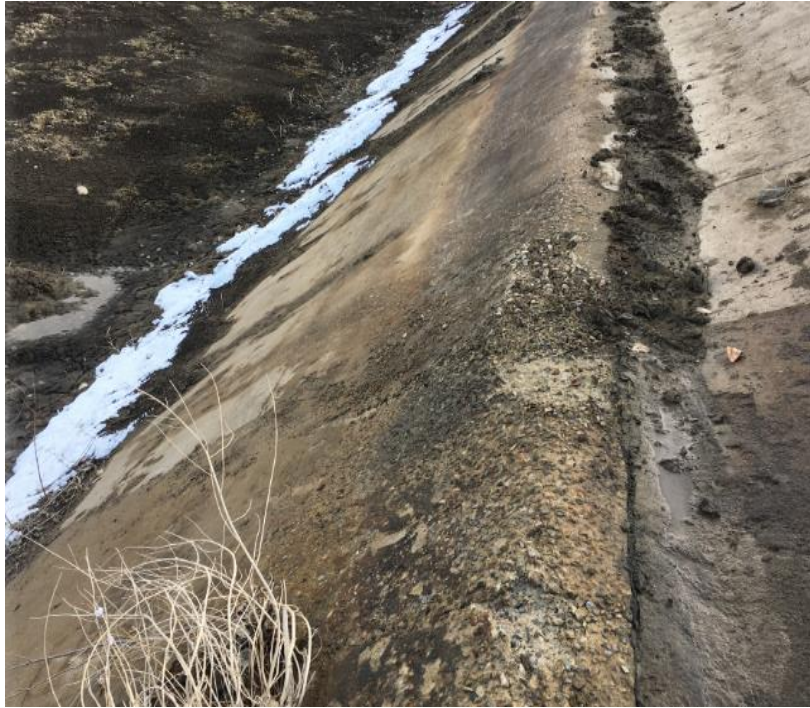
Figure 13 - Signs of Spalling with Longitudinal Crack
