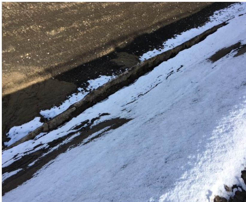
Figure 16 – Lower Lining Bulging Out
