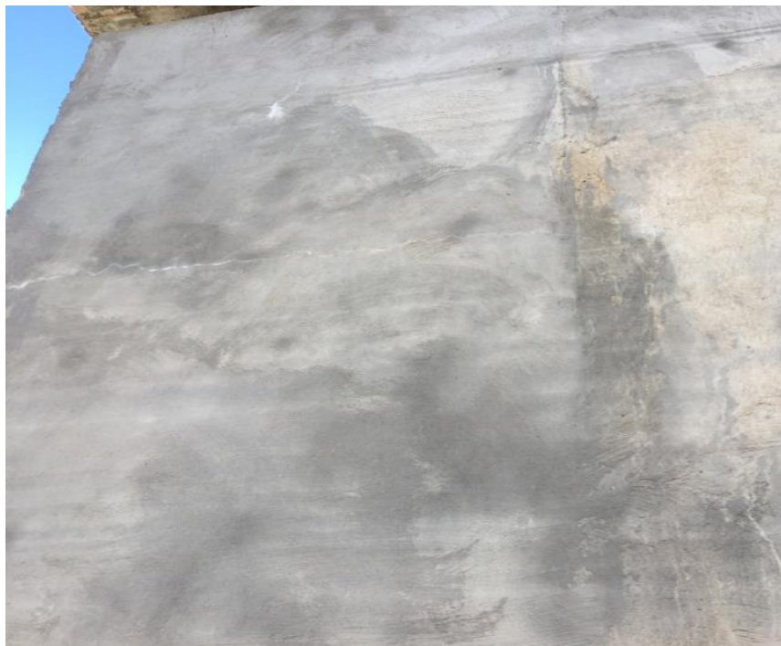
Figure 20 – Leaching in the Middle Cap of the Outlet Tower
