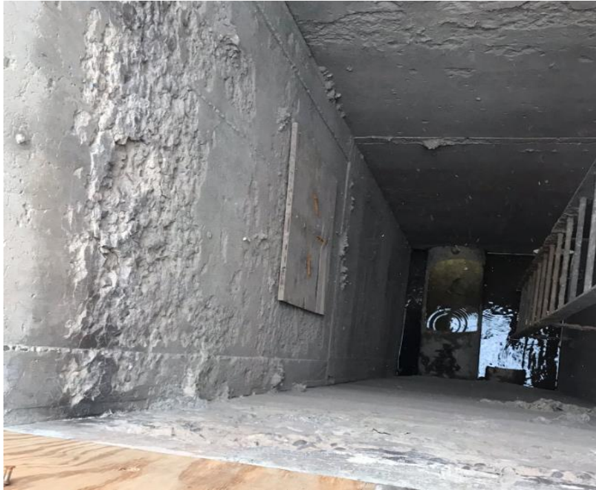
Figure 23 – Signs of Spalling
