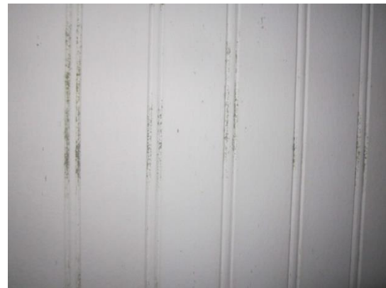
Photo #12 Example of possible mold growth.
