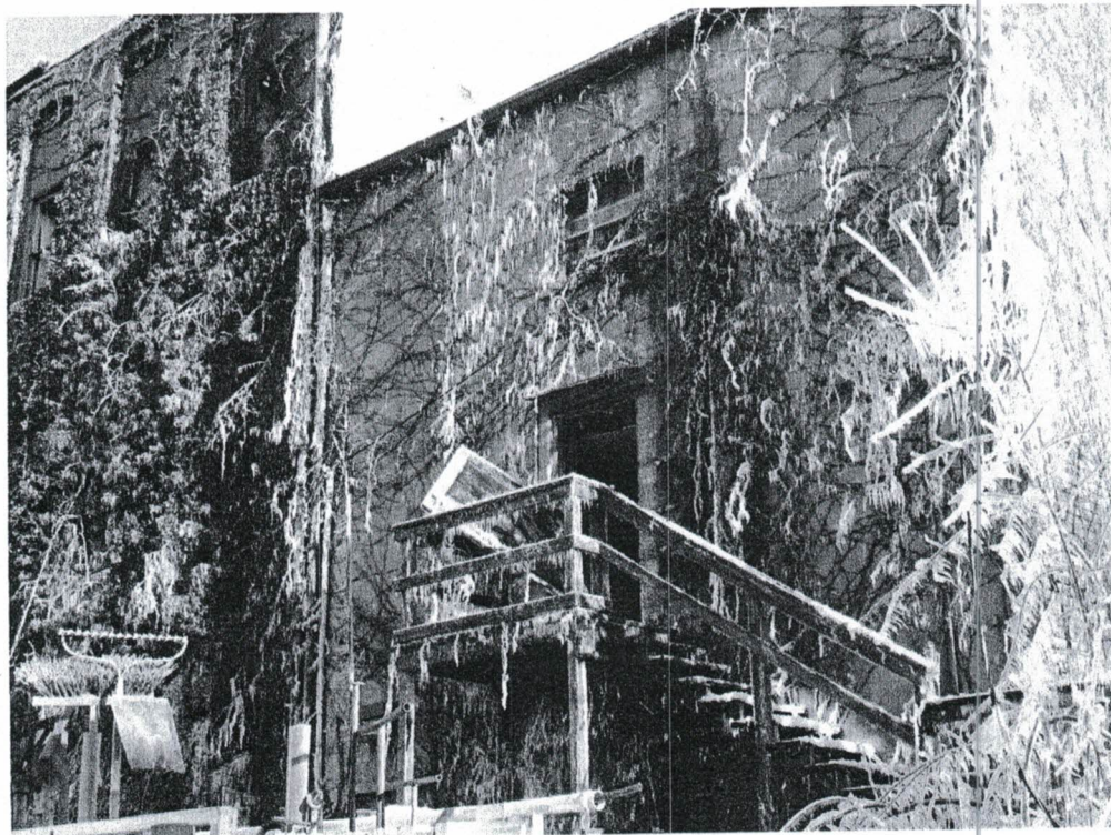
Photograph 26: The end building was not entered for this study. The door is displaced from the frame and is expected to be in a similar poor condition to the remainder of the connected buildings.
