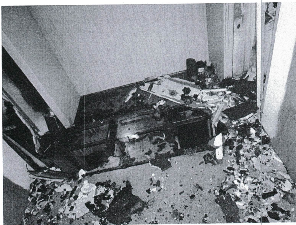
Photograph 22: The framing around the elevator is charred or completely burned away.
