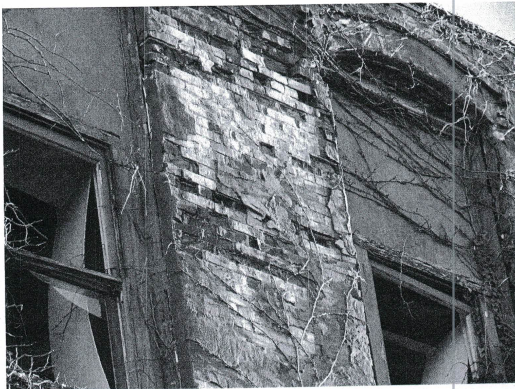
Photograph 6: The brick on the rear of the building has spalled.
