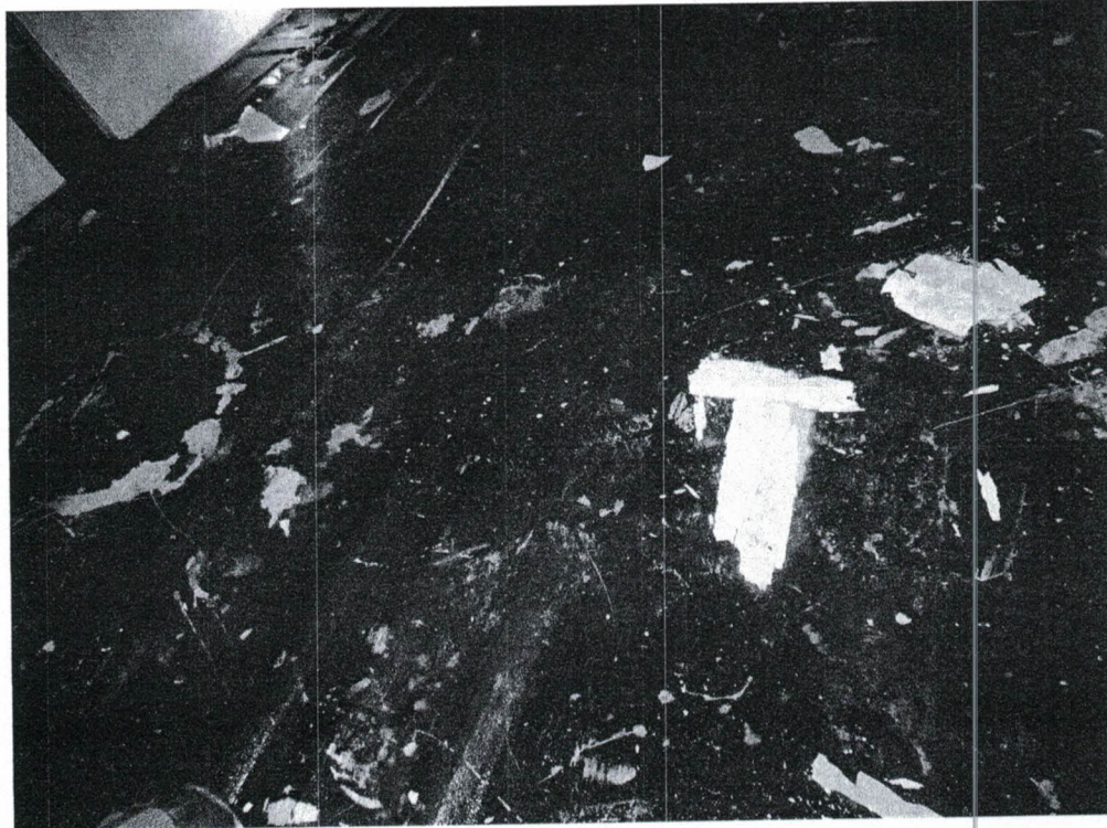
Photograph 18: Water/ice on the warped and deteriorated wood floors.
