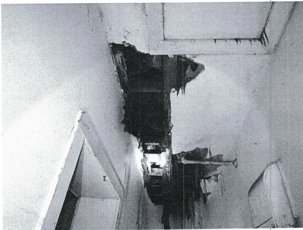
Photograph 21: Damaged drywall along the rear exit from the second floor. Icicles are present coming down from the attic and around the attic access hatch.
