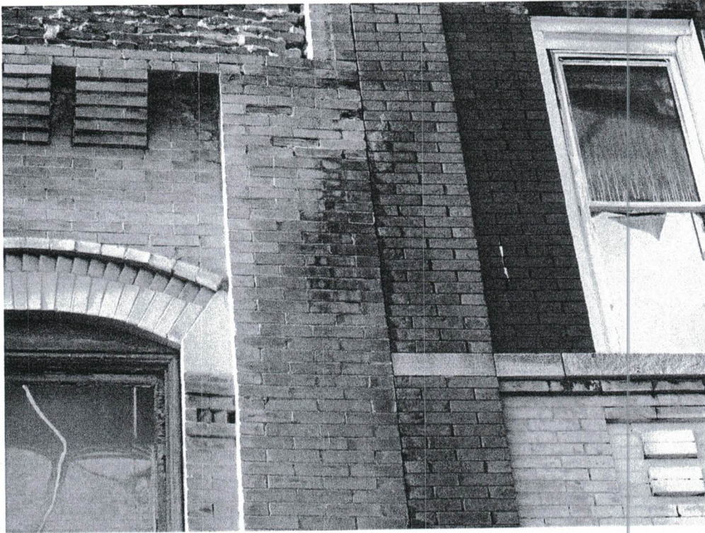
Photograph 11: Close-up of soot on the brick.
