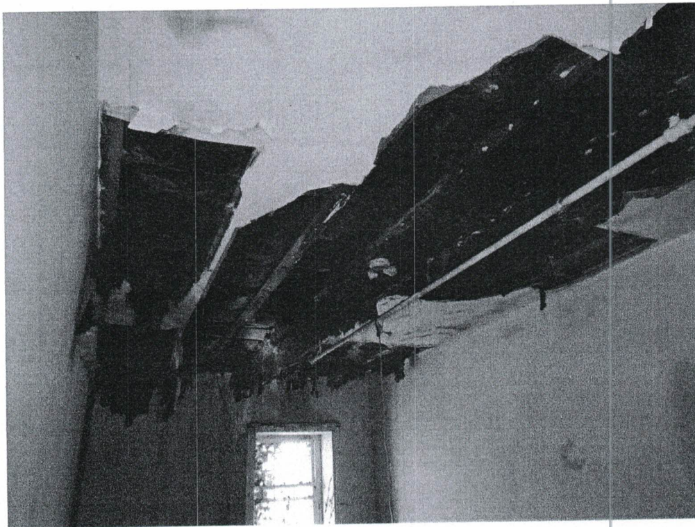
Photograph 20: The ceiling above the damaged floor is missing drywall, and the insulation is wet and frozen.
