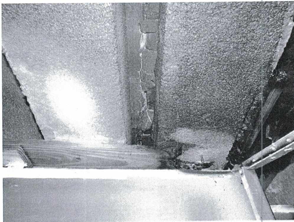
Photograph 23: The wood framing above the elevator access doorway is burned.
