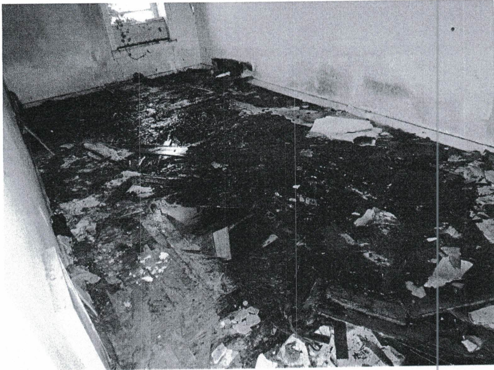
Photograph 19: Saturated and frozen floor with a large hole in it.
