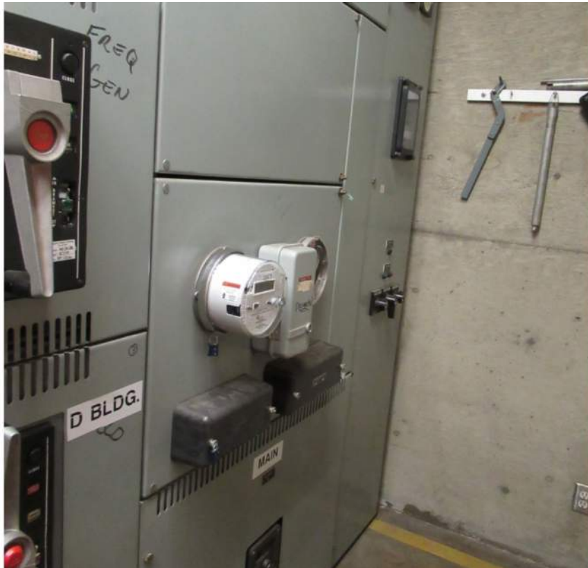
Addendum 01 – Attachment - Photos of (E) MSB in Bldg C
