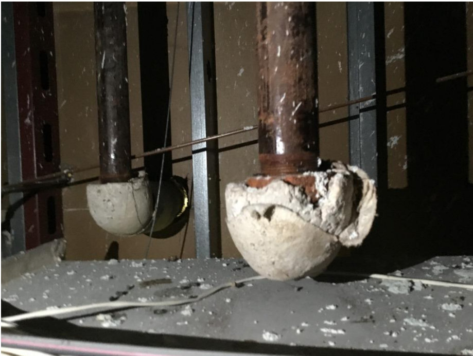
Photograph 6: View depicting the asbestos containing TSI hard pack located in the storage room located on the second floor.
