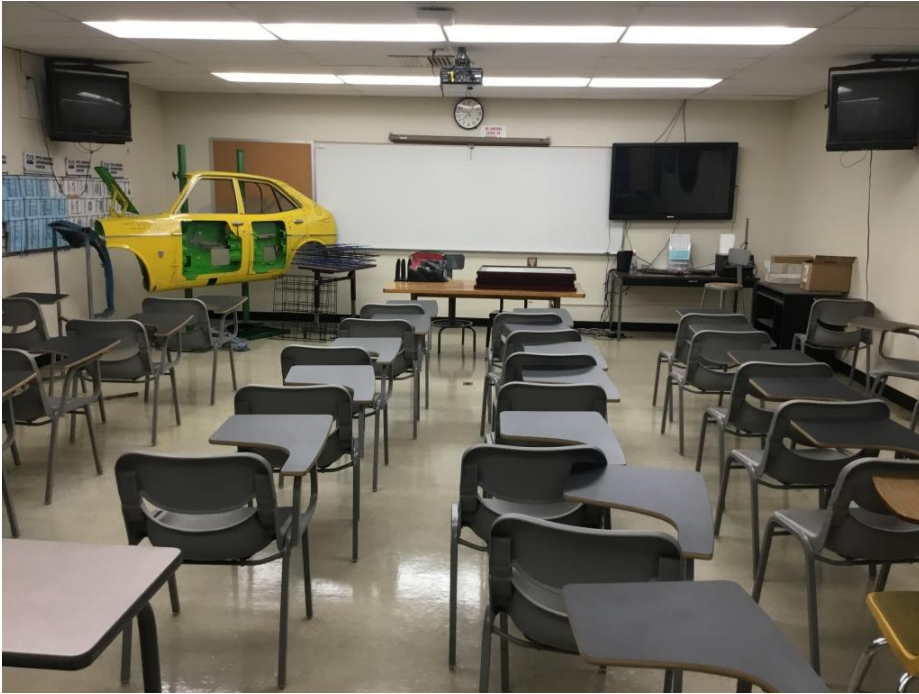
Photograph 7: View depicting the typical second-floor classroom interior. Asbestos-containing joint compound applied to the gypsum board.
