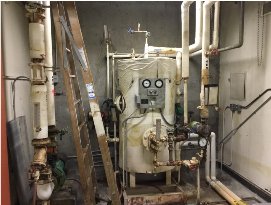
Photograph 4: View depicting the typical boiler room located on the second floor. Asbestos-containing gaskets on the piping system located on the left side of the picture.
