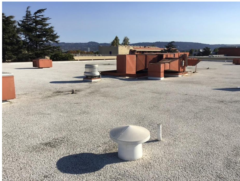
Photograph 10: View depicting the typical roof and associated HVAC system. Asbestos-containing brown insulation beneath the white gravel cap.
