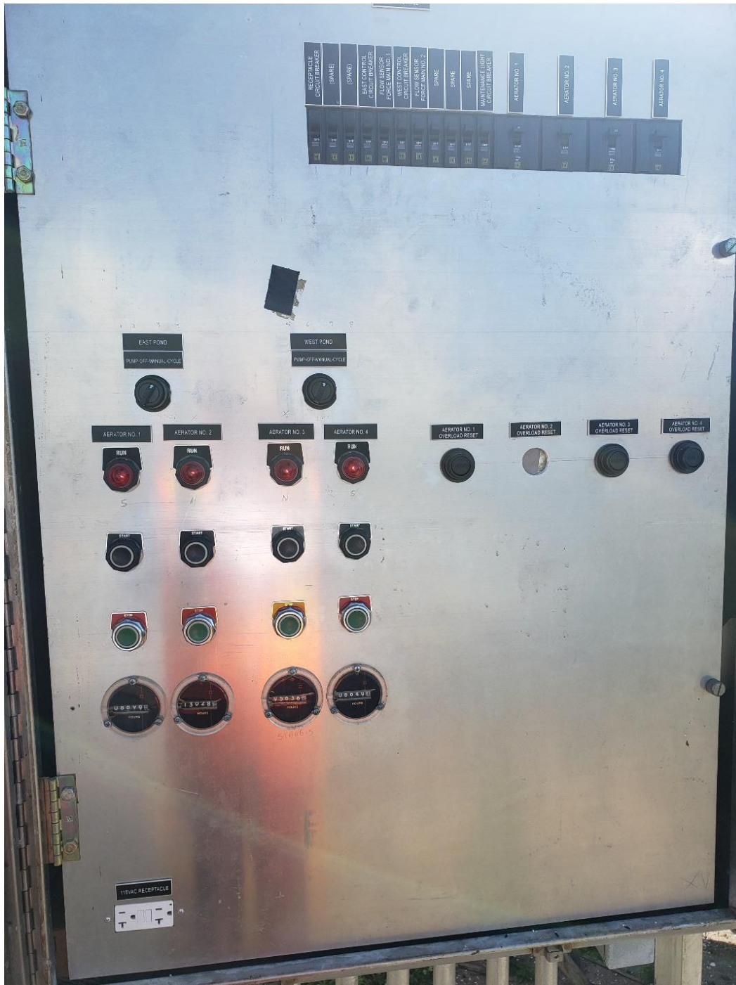
Figure 1-42 Aerator Control Access for Leachate Impoundment Basins
