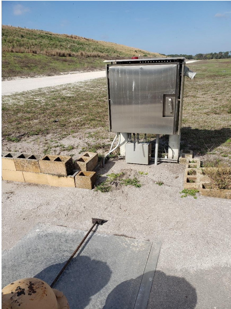
Figure 1-23 Dosing Pump Station
