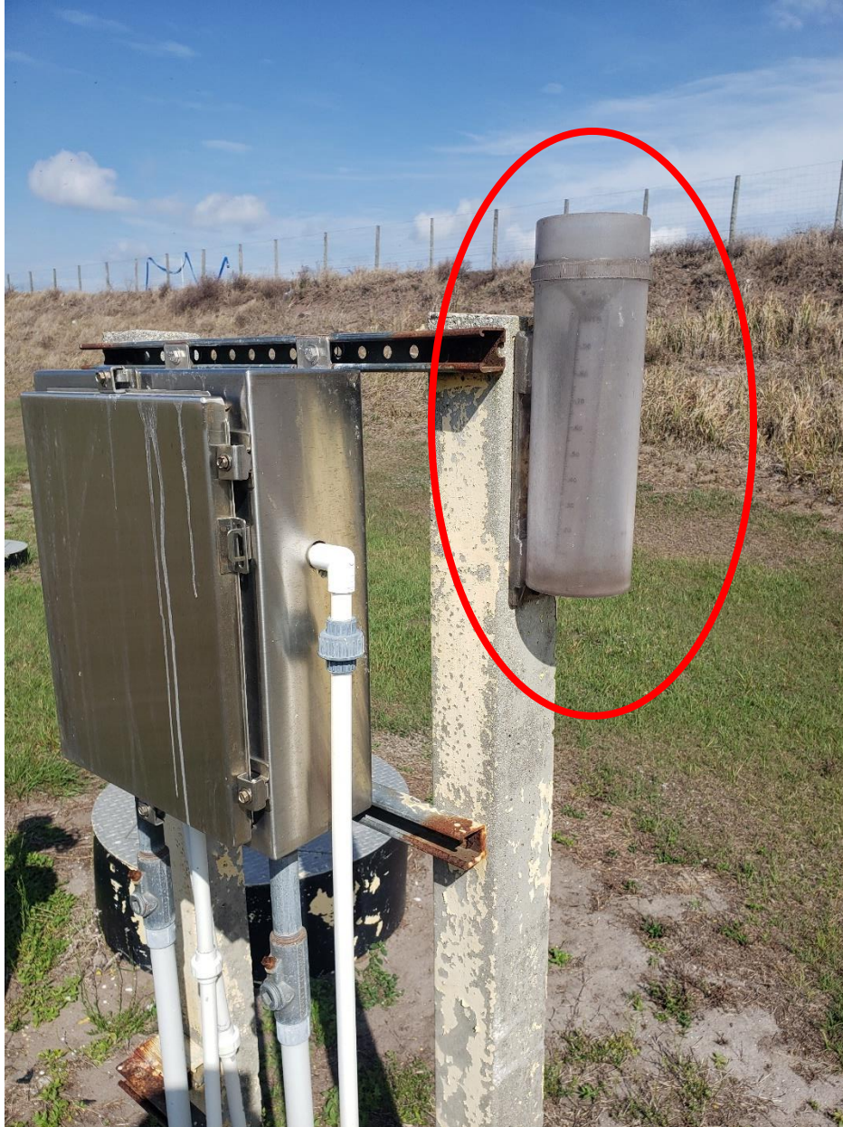
Figure 1-28 WWTP Rain Data Gauge
