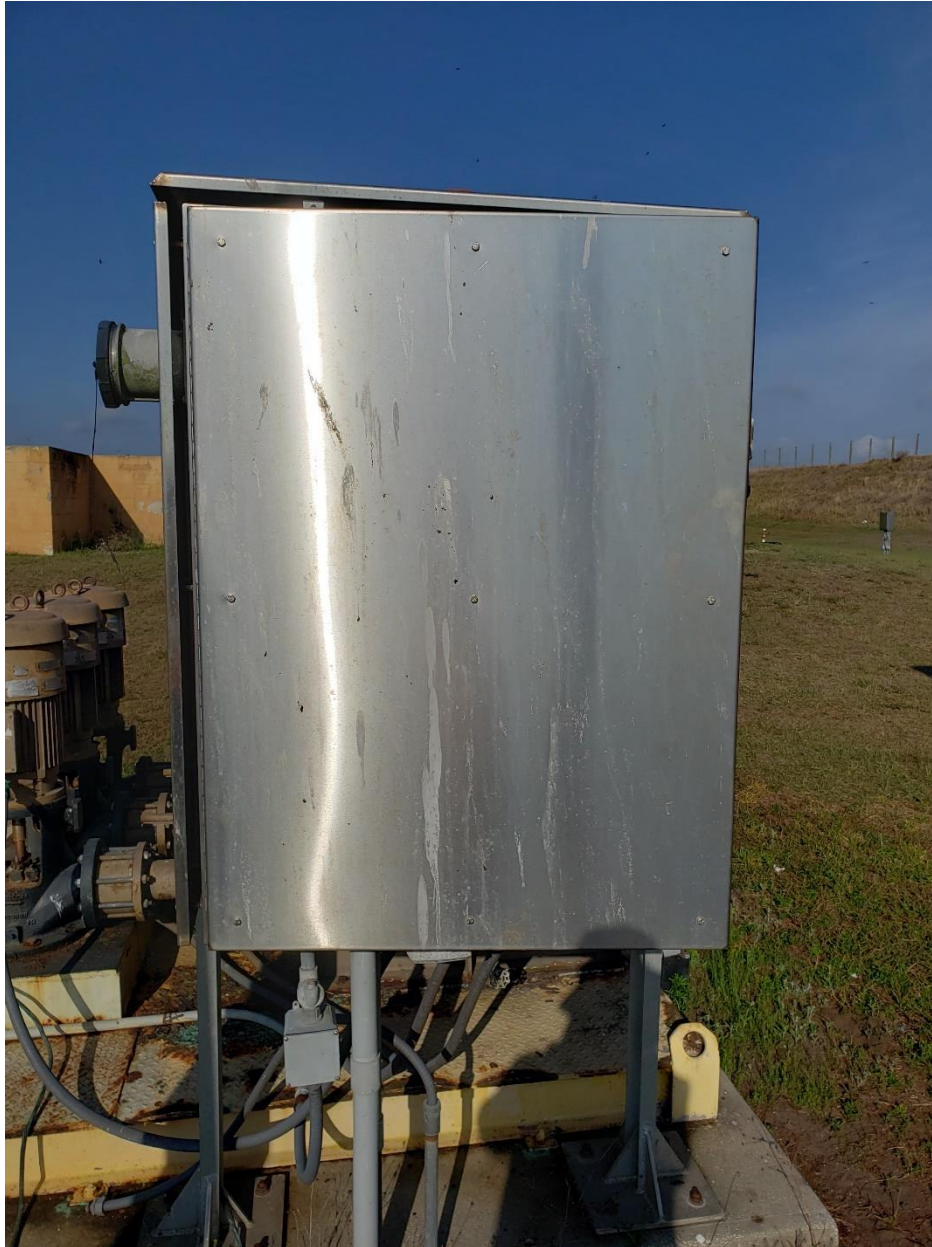
Figure 1-25 Pump Controls Access for Triplex Pump Station
