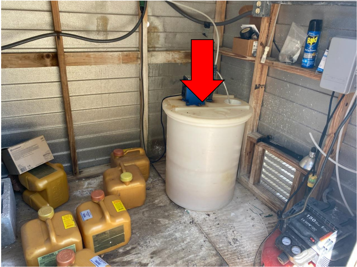
Figure 3-2 Inside the Chlorine Shed with Chlorine Barrel Shown
