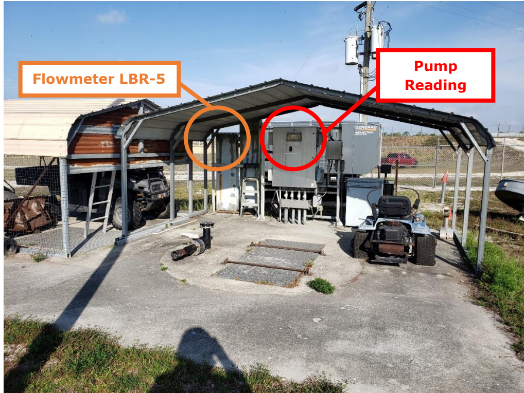
Figure 1-19 Master Lift Station
