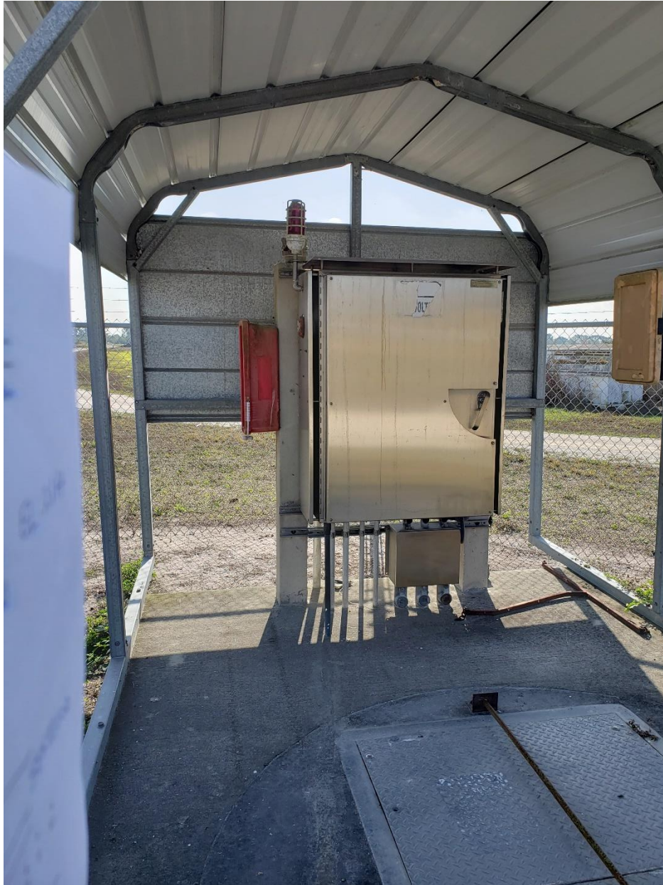
Figure 1-31 Cell 1A Lift Station Pump Controls Access
