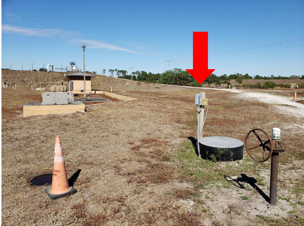
Figure 1-22 Treatment Plant Flowmeter TP-7
