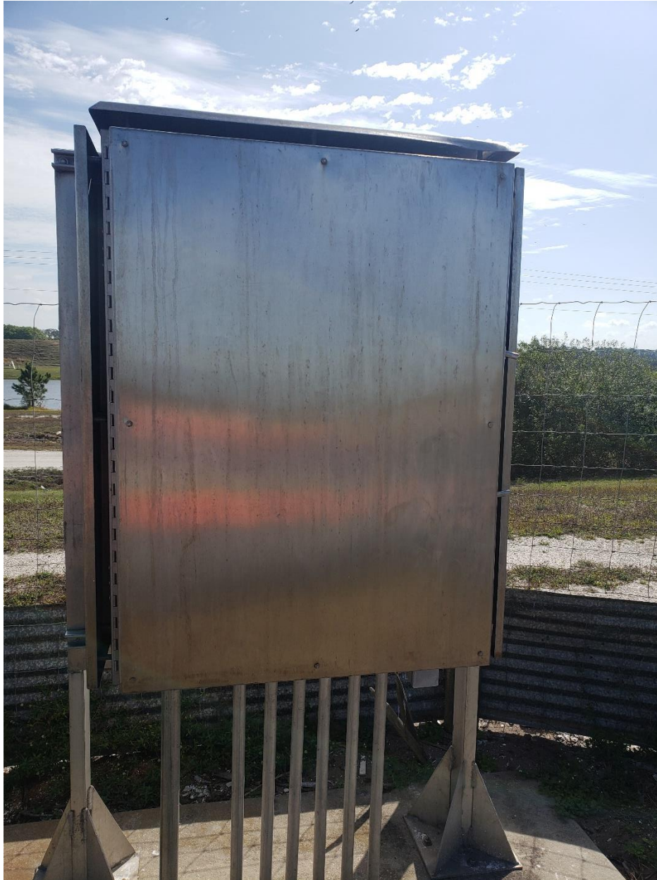
Figure 1-41 Aeration Control Access for Leachate Impoundment Basins
