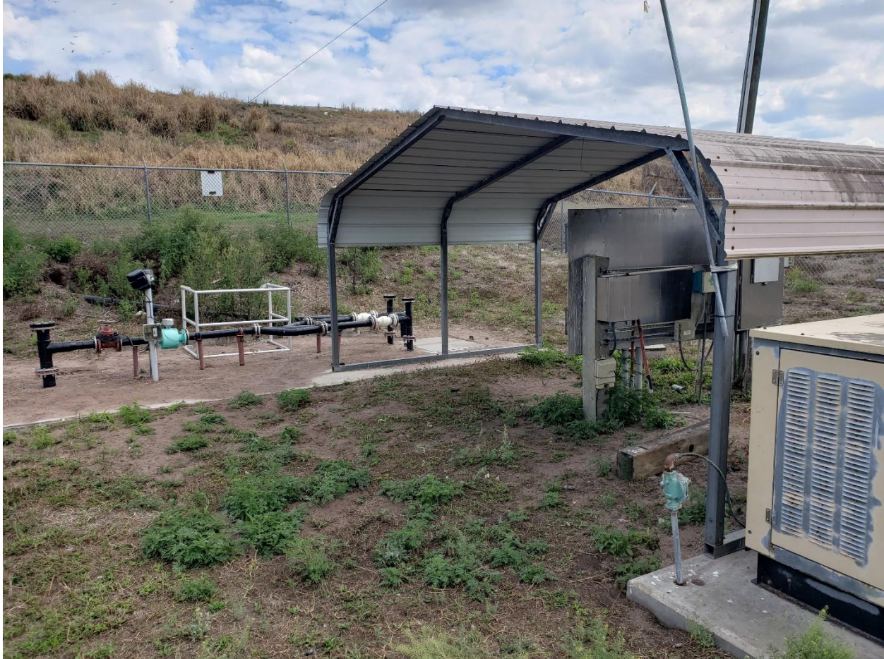
Figure 1-34 Cell 1B/3 Pump Station
