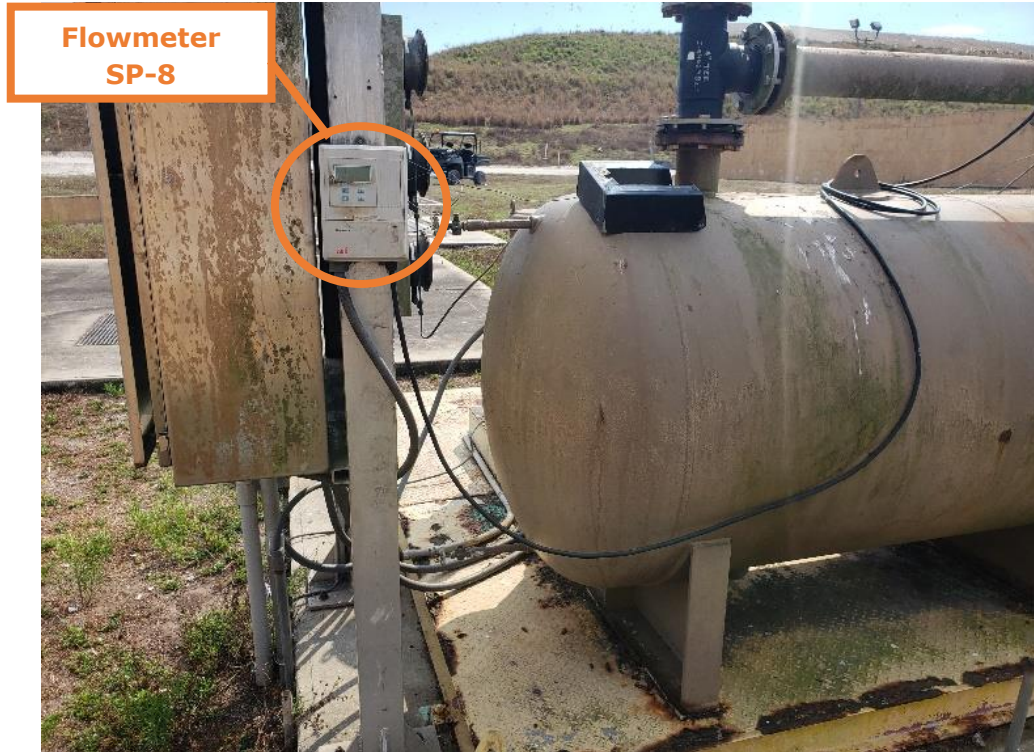
Figure 1-27 Treatment Plant Flowmeter SP-8
