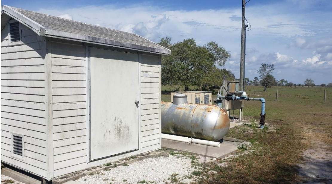
Figure 1-46 Well/Pump Irrigation (Supply Well Water) Station
