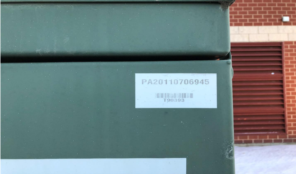
Courthouse Transformer Label
