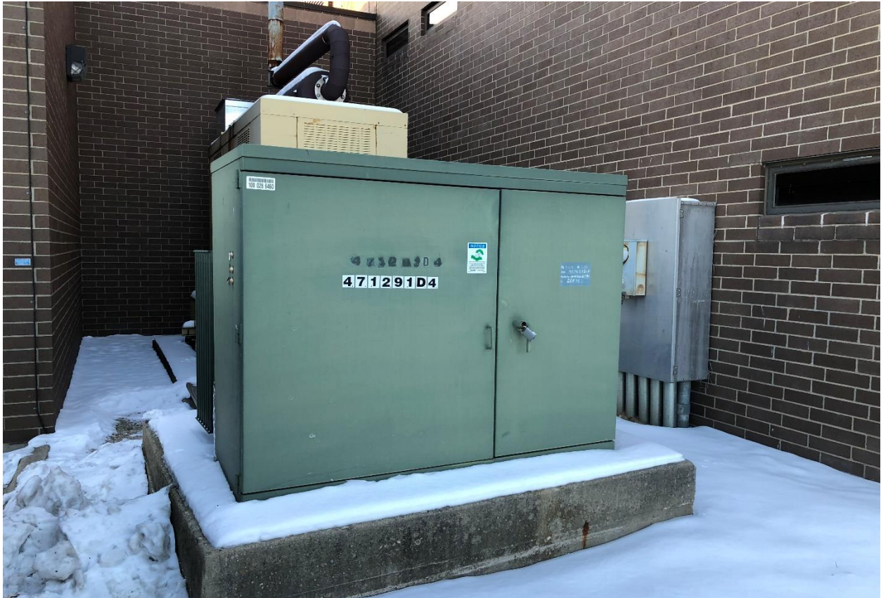
Public Safety Center Transformer
