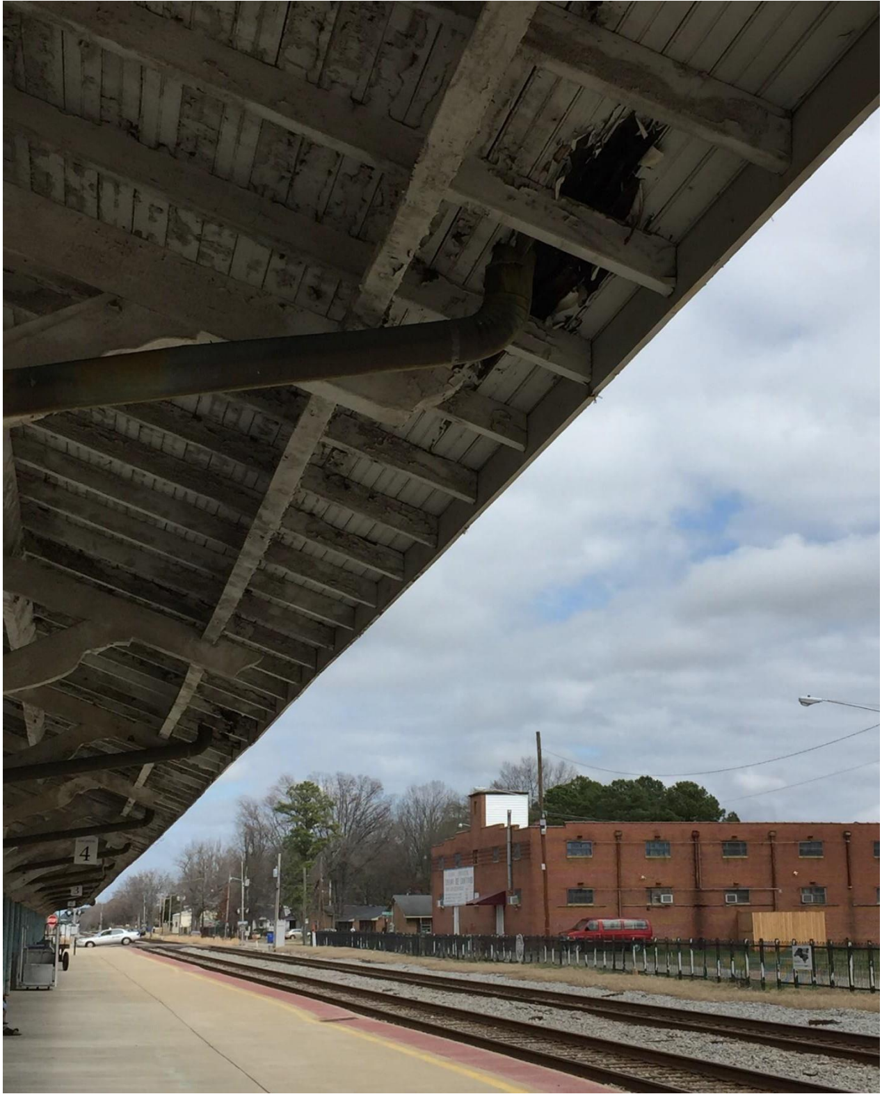
Water Damage At Roof Drain
