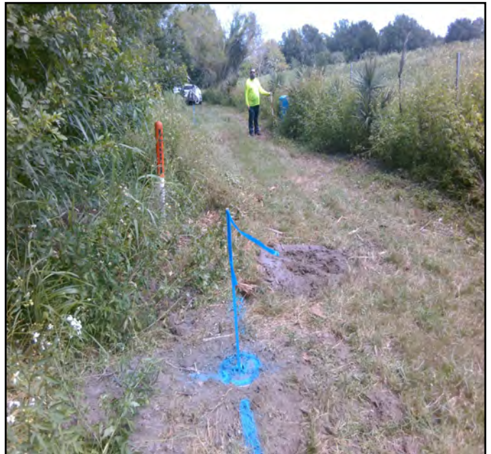
Tie 02 (From Test Hole): VALVE, WATER
