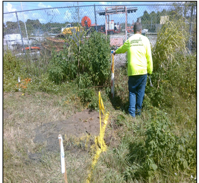
Tie 02 (From Test Hole): GAS MARKER
