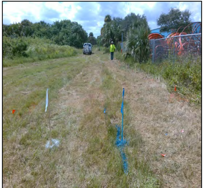
Tie 02 (From Test Hole): COMM HH
