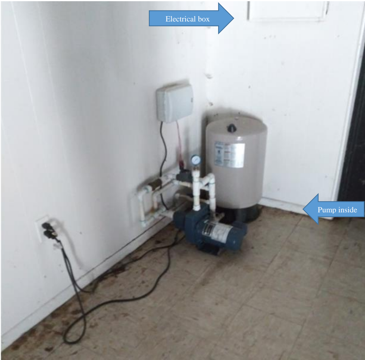
Water pump located inside of building in the northwest corner
