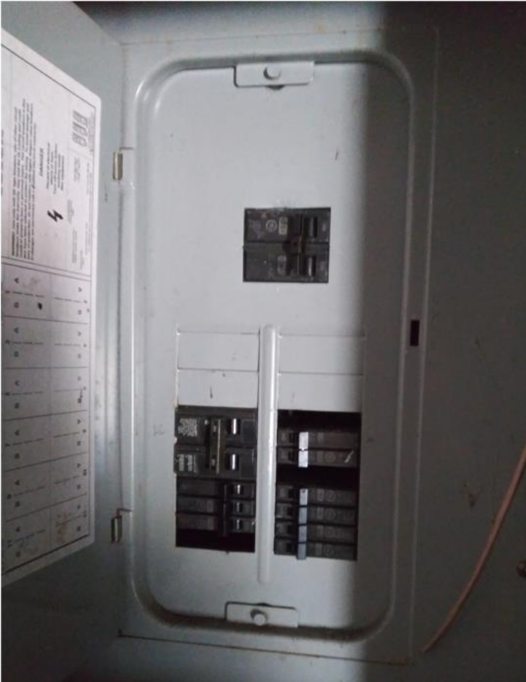
View of electrical box located above the water pump on the north interior wall
