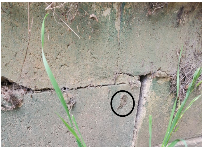
Photo 5 – Caulk located sporadically on foundation CMU blocks.
