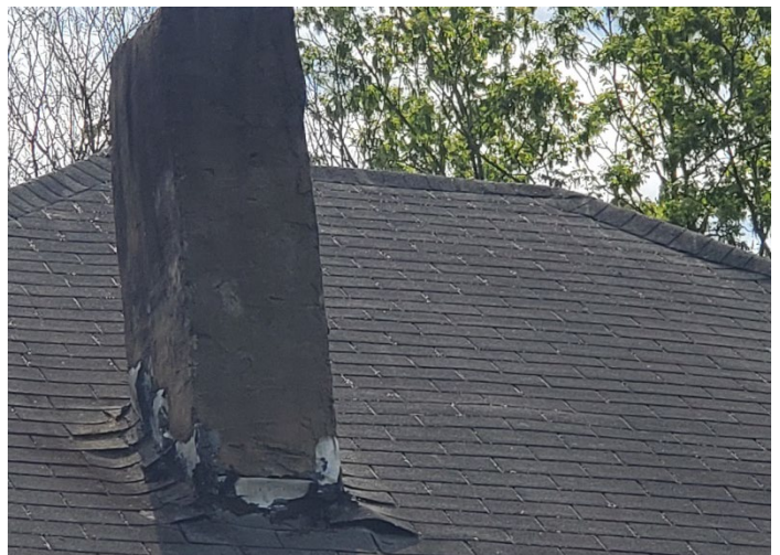
Photo 10 – Chimney tar is assumed asbestos containing material.
