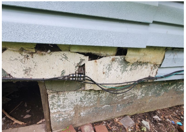
Photo 4 – Top layer of vinyl siding over transite siding. Transite is over wood siding. Transite is ACM.
