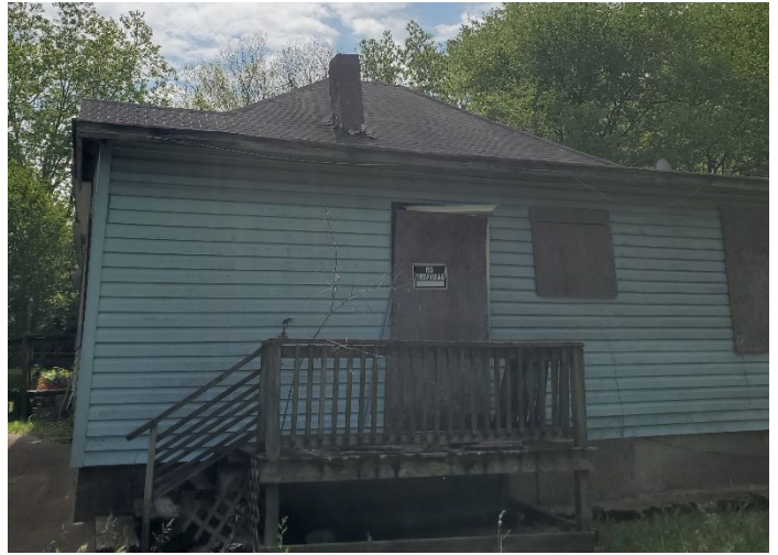
Photo 2 – Side view of 1010 Carson Avenue. Porch has missing floor boards and steps unstable.
