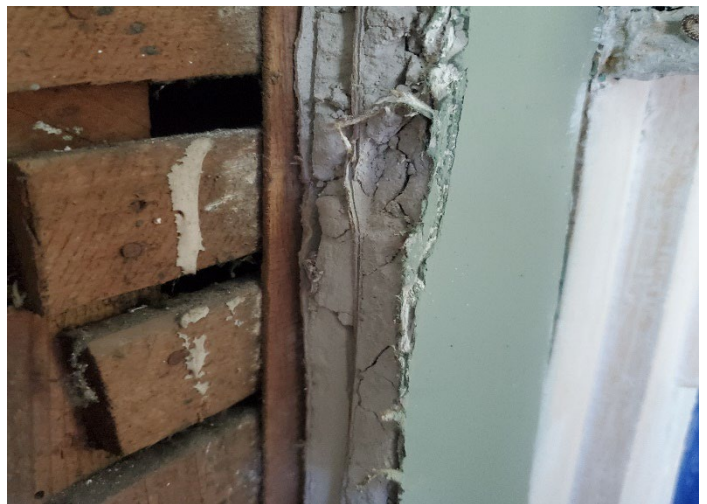
Photo 8 – Double layers of drywall located sporadically throughout the walls.
