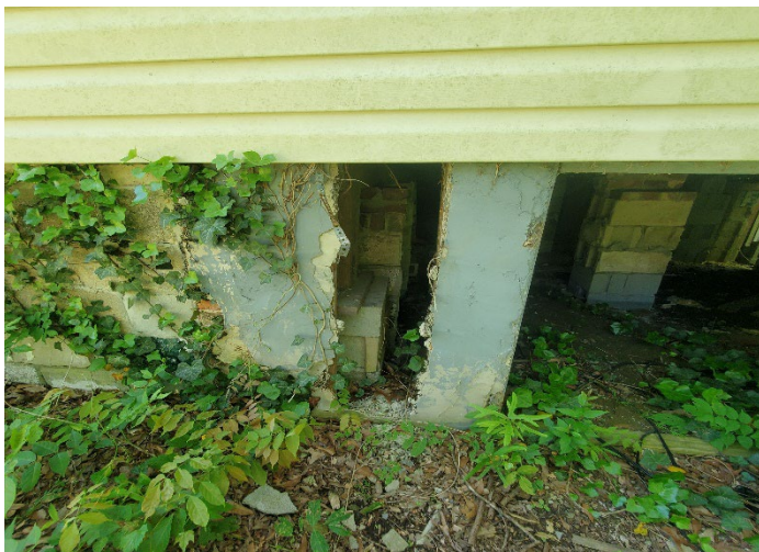
Photo 9 – Plaster and skim coat located on exterior foundation.
