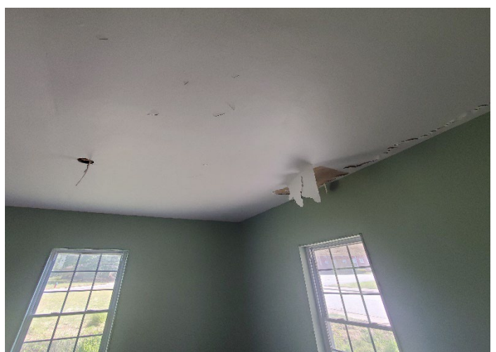
Photo 4 – Ceiling with flat skim coat over plywood located in back right room, front right and left rooms.
