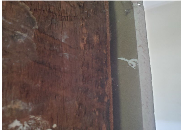
Photo 6 – White caulk found sporadically throughout interior door ways
