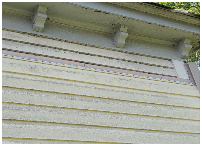
Photo 10 – Transite and two layers of felt located under vinyl siding. Gray transite is ACM.
