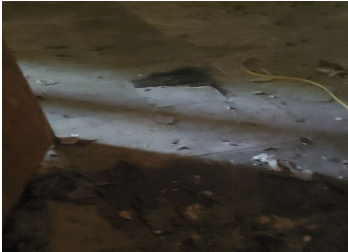
Photo 5 – Roll vinyl with glue located within kitchen area.
