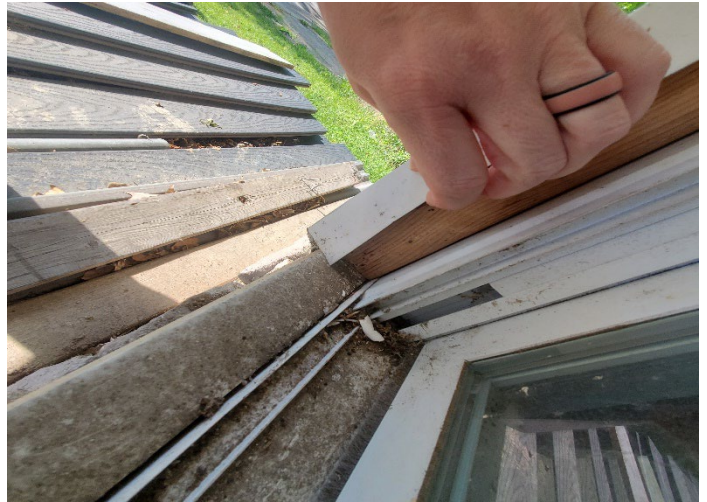
Photo 2 – Exterior vinyl windows with metal wrap and no caulk
