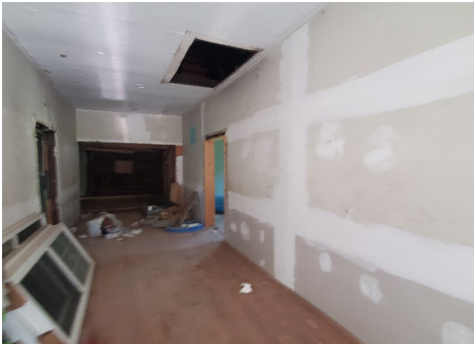
Photo 3 – Drywall and joint compound throughout walls.
