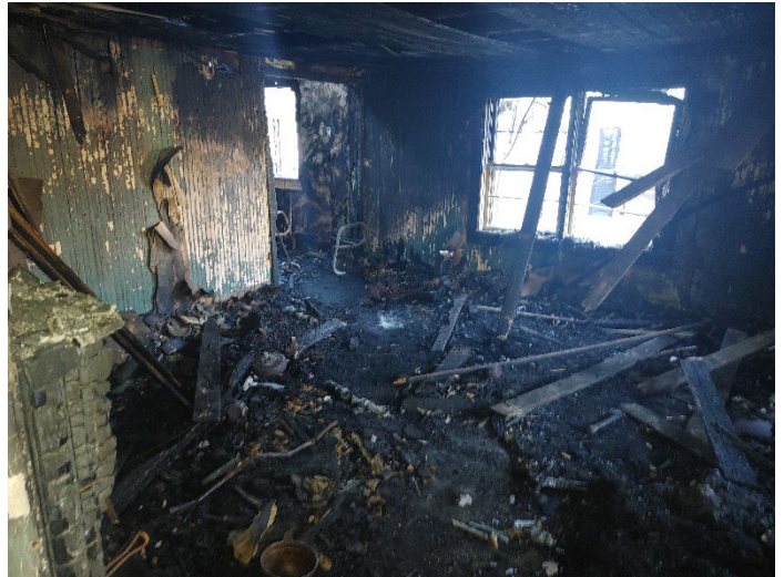
Photo 8 – Typical view of fire damage
