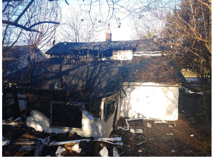
Photo 2 – Rear of property showing fire damage.
