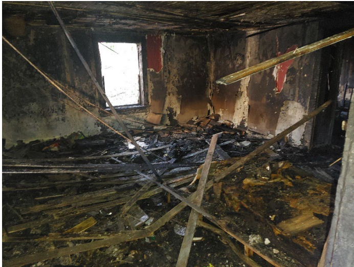
Photo 7 – Typical view of fire damage
