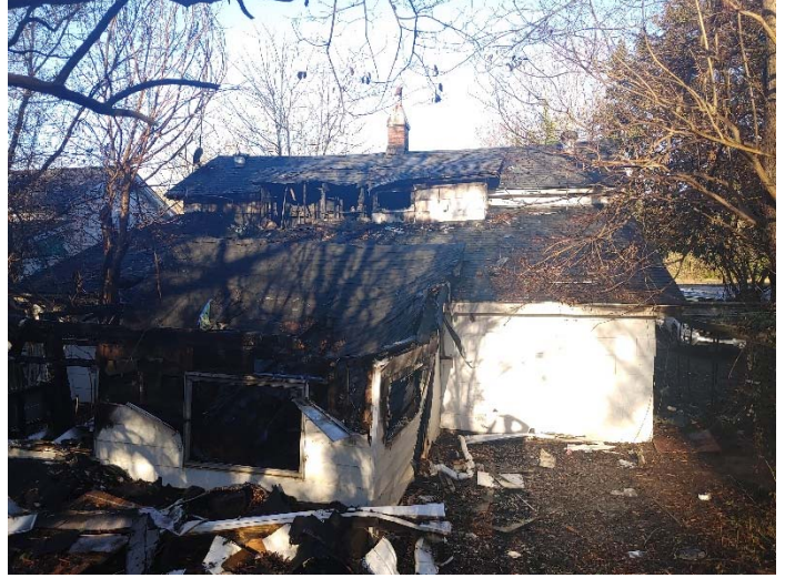
Photo 6 – Typical view of fire damage
