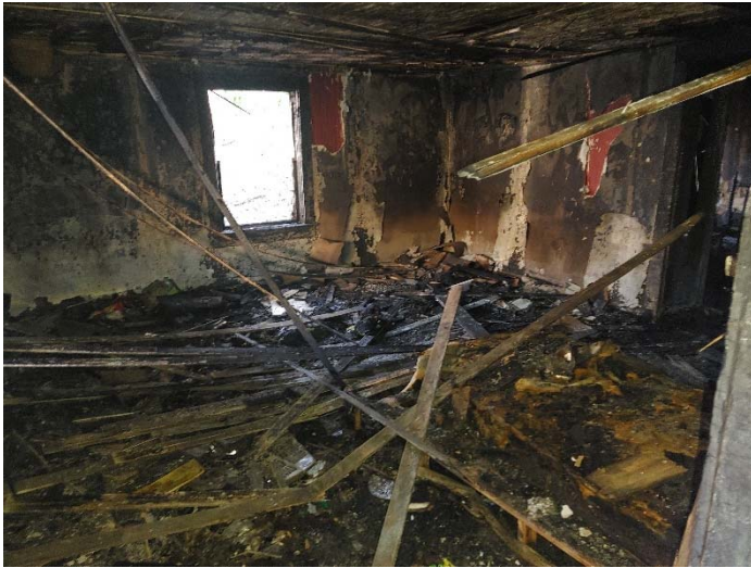
Photo 7 – Typical view of fire damage
