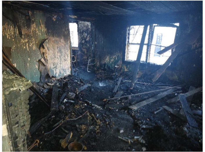
Photo 8 – Typical view of fire damage
