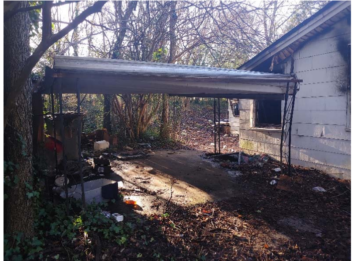
Photo 2 – Exterior carport/canopy with hard white caulk on the front side of the roof
