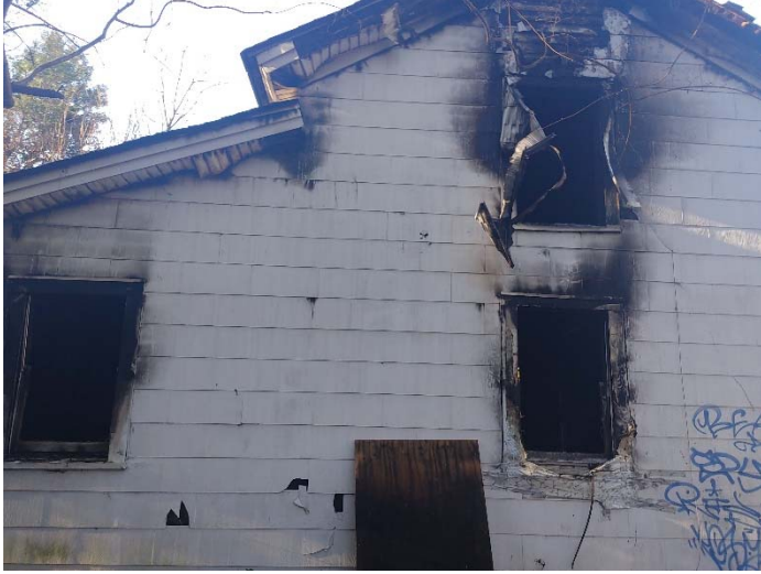
Photo 5 – Typical view of fire damage
