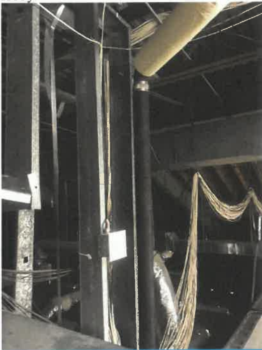
HVAC system above ceiling tiles in public lobby
