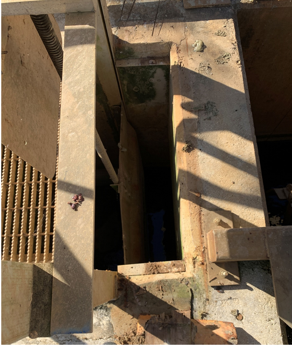
VIEW BEHIND SLIDE GATE #4 (FLOW IS TOWARD THE LEFT OF THE PAGE)
