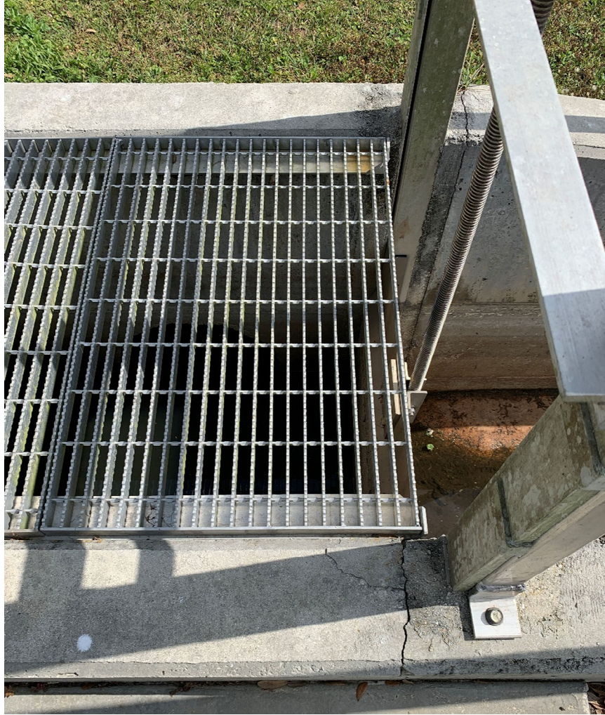
SLIDE GATE #5 (LOOKING EAST). NEW GATE GOES TO THE LEFT OF THE EXISTING GATE LOCATION.
