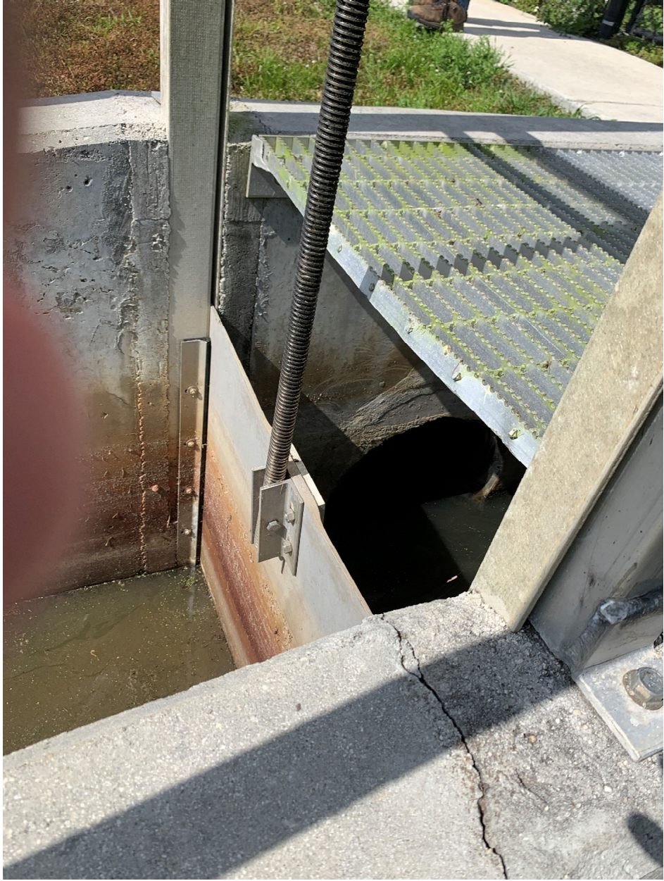
SLIDE GATE #6 (LOOKING WEST). NEW GATE GOES TO THE RIGHT OF THE EXISTING GATE LOCATION.
