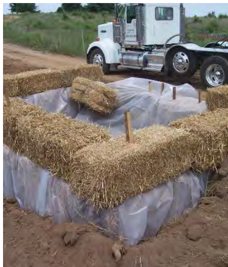
Example washout structures. Note that each example is fully lined and the washout is contained.
