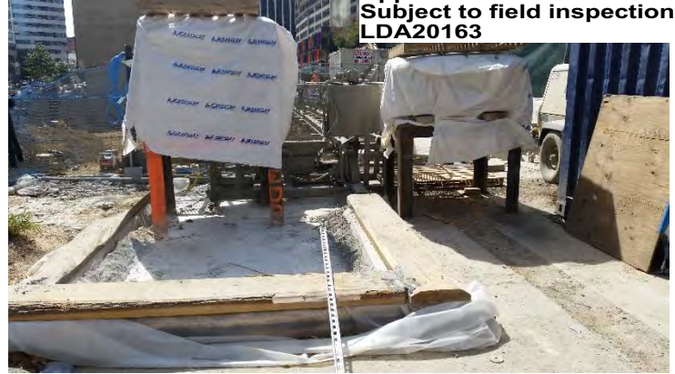
Chemical storage example. Containers are closed, covered by a tarp, and off of the ground.
