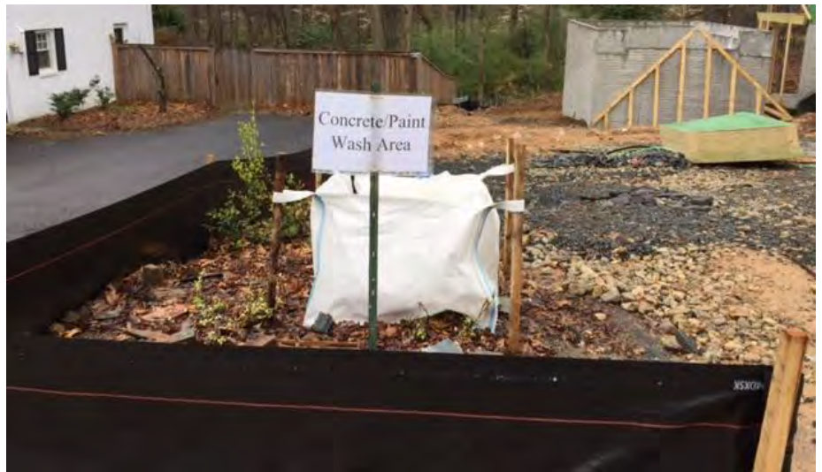
Example small-scale concrete and paint washout area.
