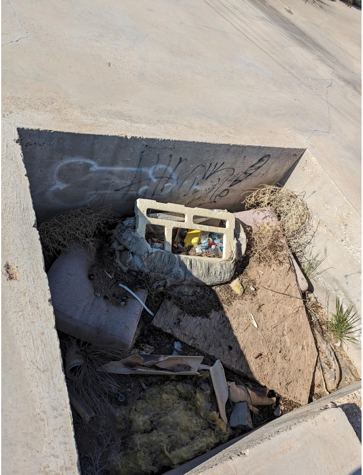
Trash in concrete slab lot 9A .jpg
