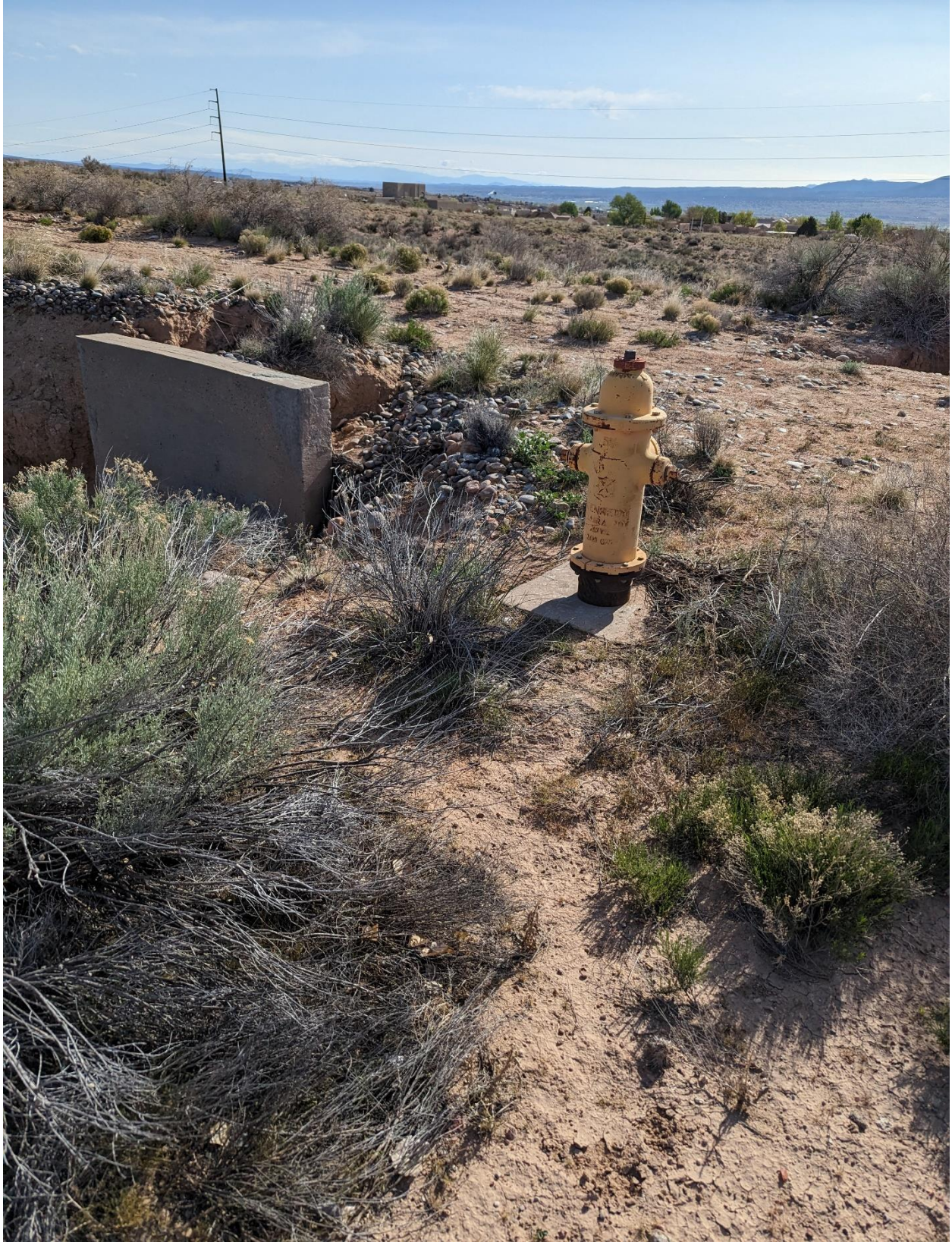
Fire hydrant by southeast side of storm drain.jpg
