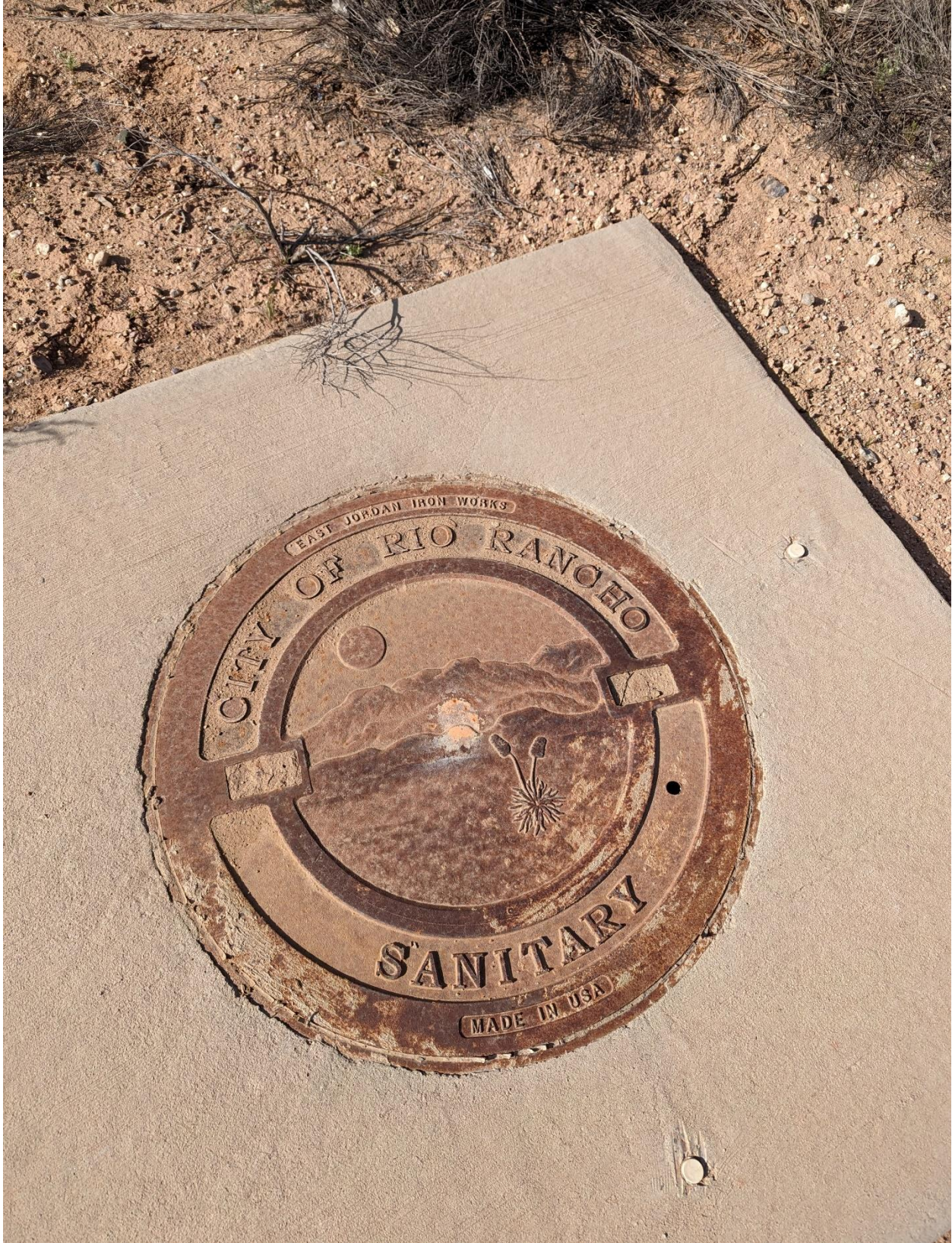
City of Rio Rancho Sanitary Sewer on southwest corner of lot 9A.jpg
