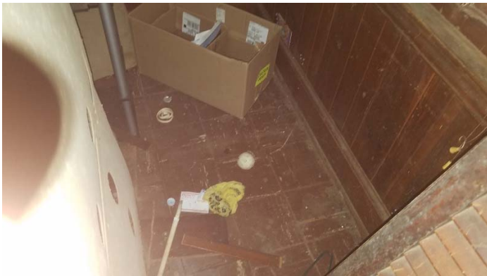
Photo 9 – Front right room burgundy 9"x 9" floor tile and mastic.
