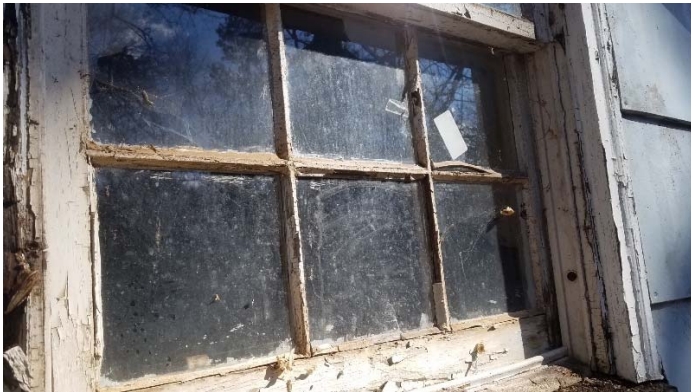
Photo 3 – Window glaze and caulk.
