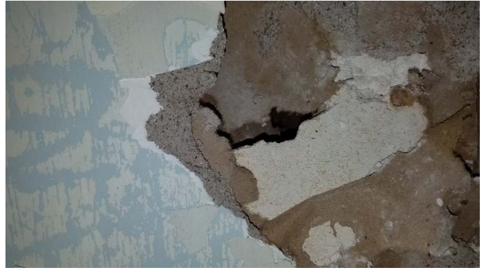
Photo 14 – Plaster over unfinished drywall.
