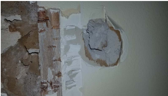
Photo 15 – Transition from plaster over drywall to drywall with joint compound at front window repair.
