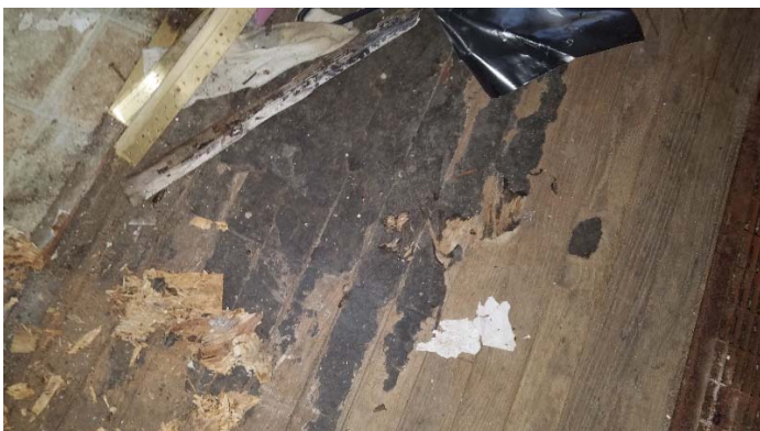
Photo 11 – Black felt on wood flooring in bathroom, hallway and hall closet floor.
