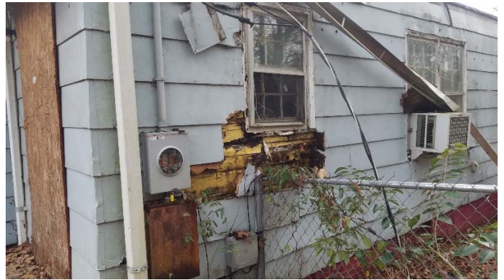
Photo 2 – Black felt under wood siding.
