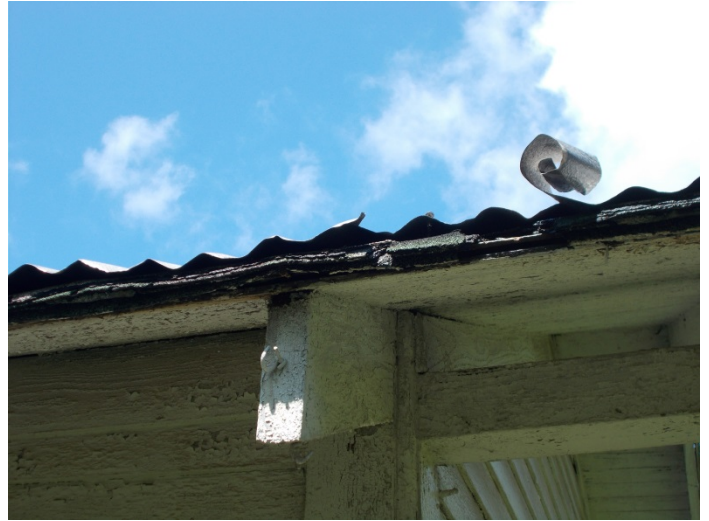
Photo 8 - Four layers of shingles and a layer of felt on the pitched wooden roof.
