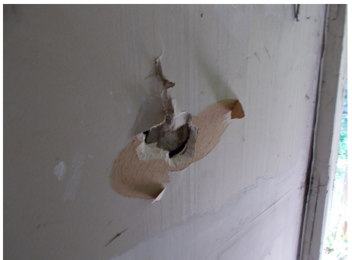
Photo 6 – Drywall with joint compound in the back room.
