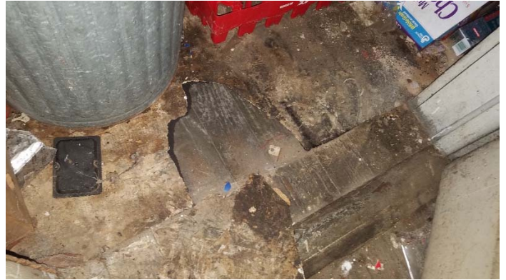
Photo 8 – Back porch closet flooring.
