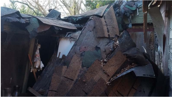
Photo 7 – Back porch collapsed roof.
