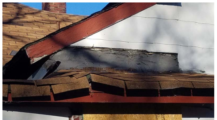
Photo 6 – Assumed asbestos back porch roof flashing tar.
