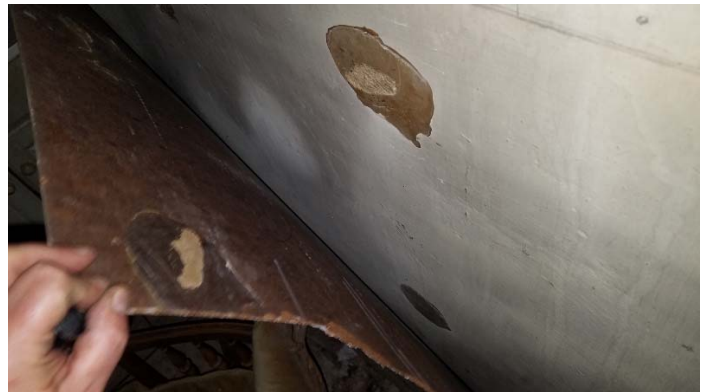
Photo 10 – Bathroom mastic behind wall-board.
