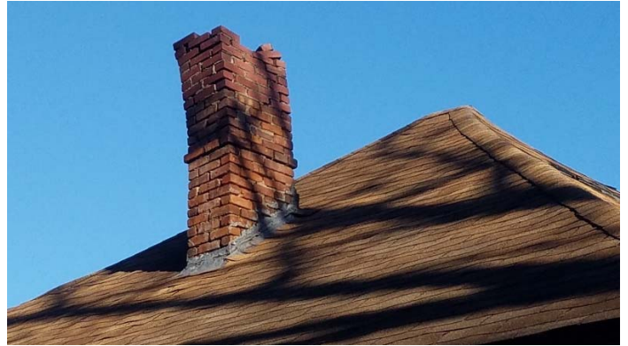
Photo 2 – Shingled Roof and assumed asbestos black tar on damaged, leaning chimney. 2 chimneys exist.
