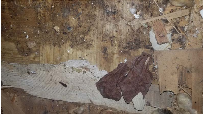
Photo 7 – Kitchen wood pattern roll vinyl flooring with mastic under tile and wood sub-floor.
