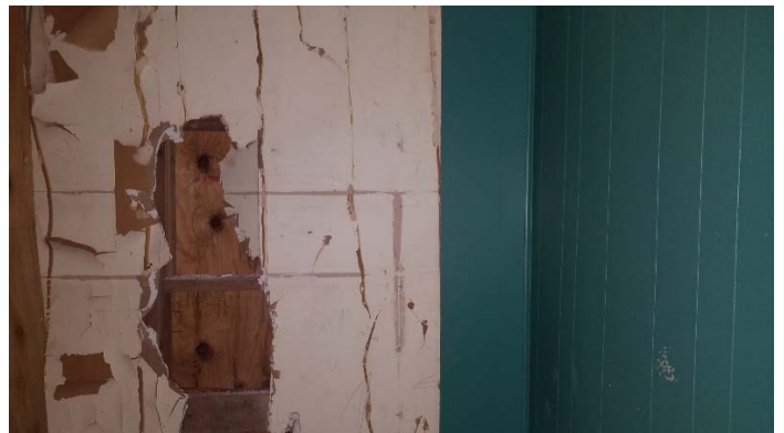
Photo 6 – Mastic behind wooden wall paneling.
