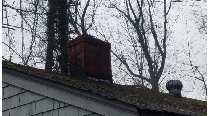
Photo 2 – Assumed asbestos chimney tar.
