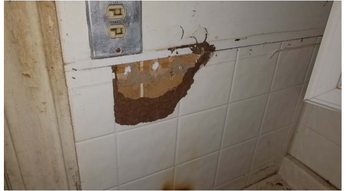
Photo 8 – Bathroom mastic behind wall-board.
