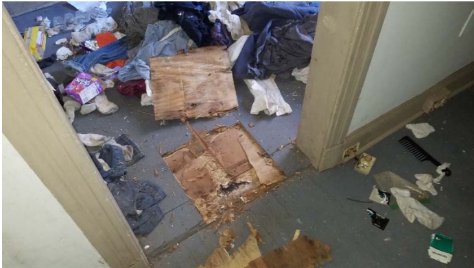
Photo 9 – Kitchen flooring under wood sub-floor.
