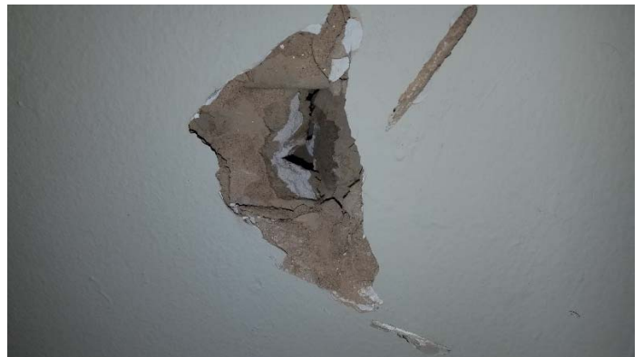
Photo 6 – Plaster over unfinished dry wall.
