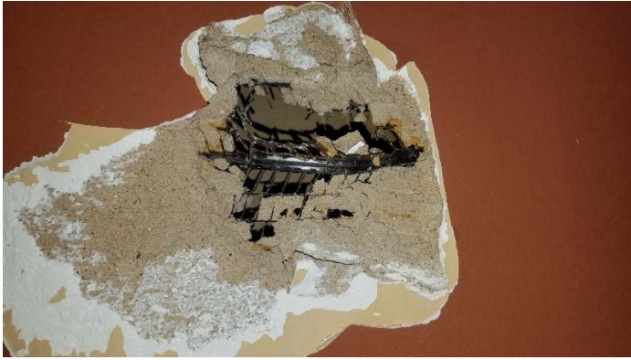
Photo 7 – Plaster over expanded metal without dry wall.
