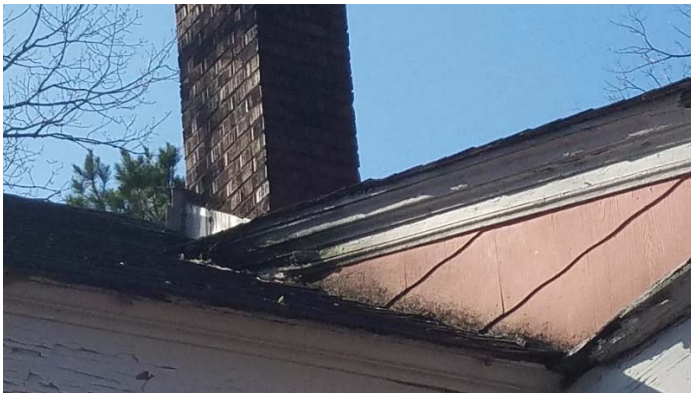
Photo 3 – 2 Chimneys with assumed asbestos chimney tar.
