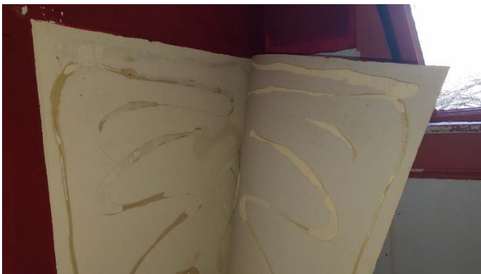
Photo 11 – Bathroom tub-surround mastic.
