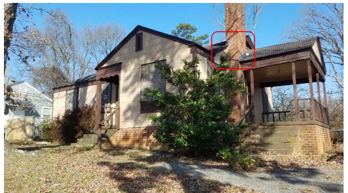
Photo 4 – Chimney flashing tar.
