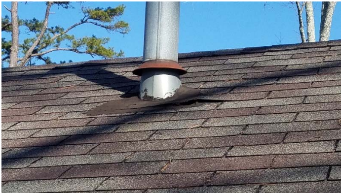
Photo 3 – Roof vent tar same as roof valley.
