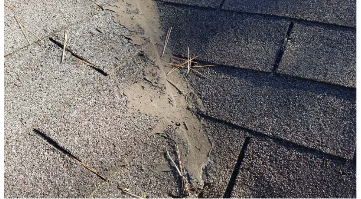
Photo 2 – Roof valley tar.
