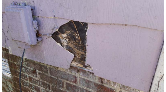
Photo 2 – Transite exterior siding with felt.
