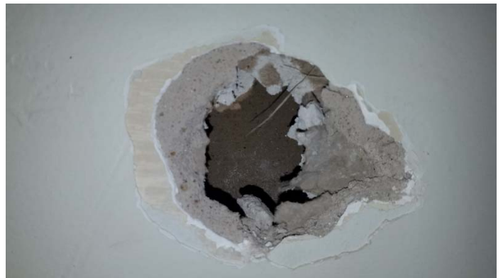
Photo 6 – Plaster over unfinished dry wall.
