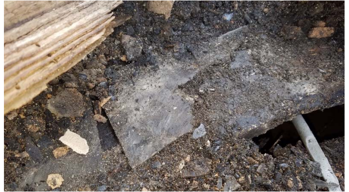
Photo 8 – right middle room flooring.
