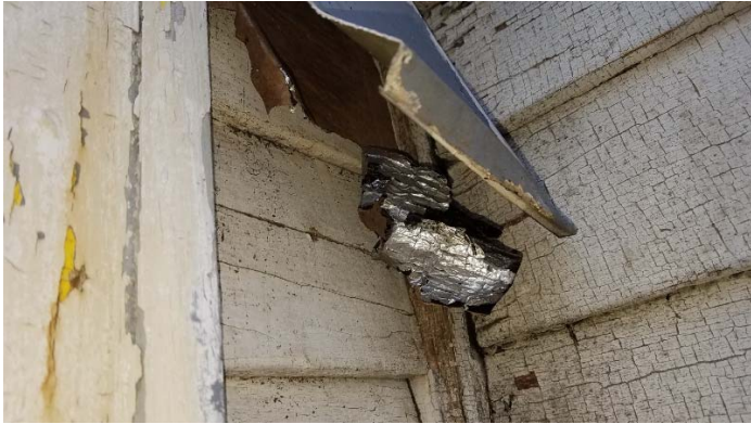
Photo 7 – Aluminum wrap with black layer under exterior siding.
