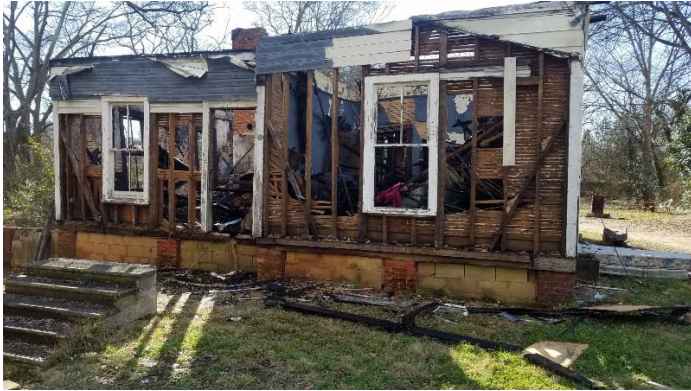
Photo 1 – 938 Ansel Street in Spartanburg, South Carolina. Typical view of fire damage throughout the residence.
