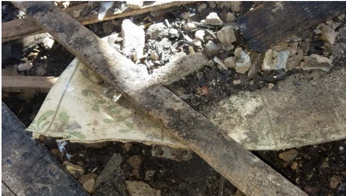
Photo 9 – right rear room flooring.
