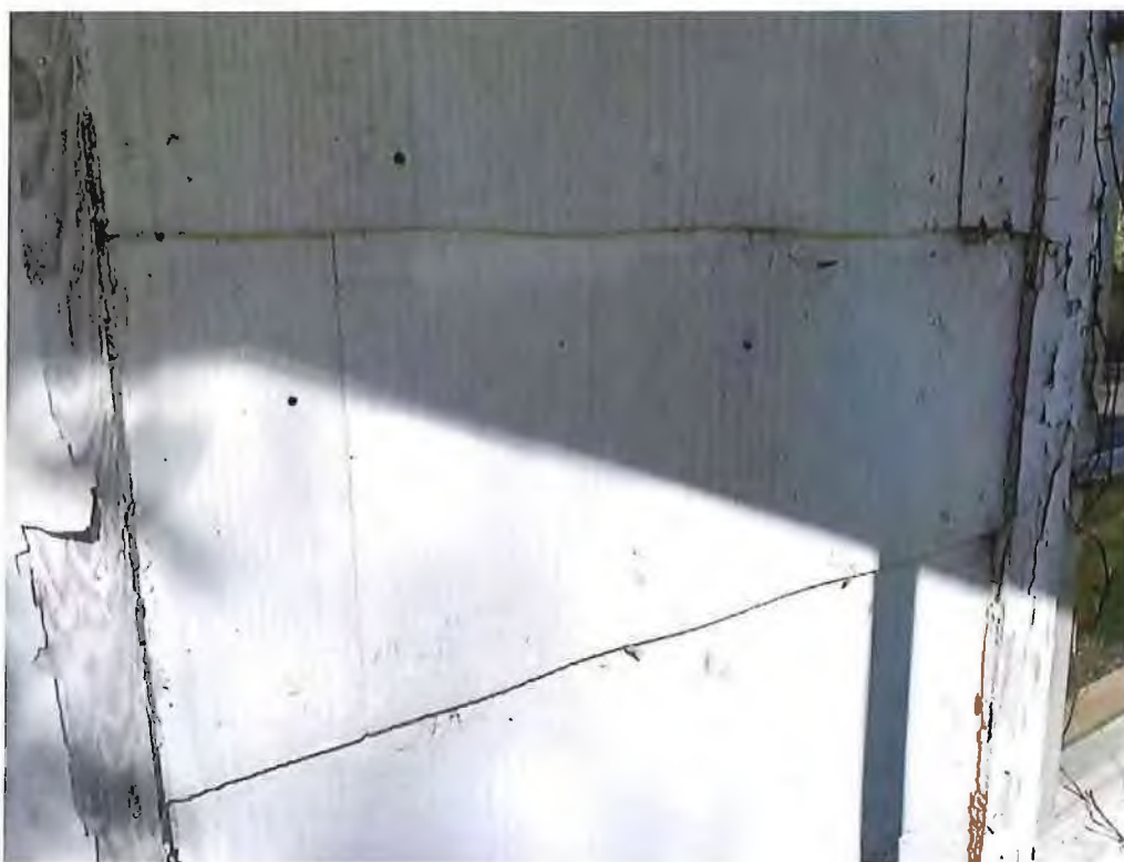
Asbestos Containing Exterior Transite Siding, Radio House
