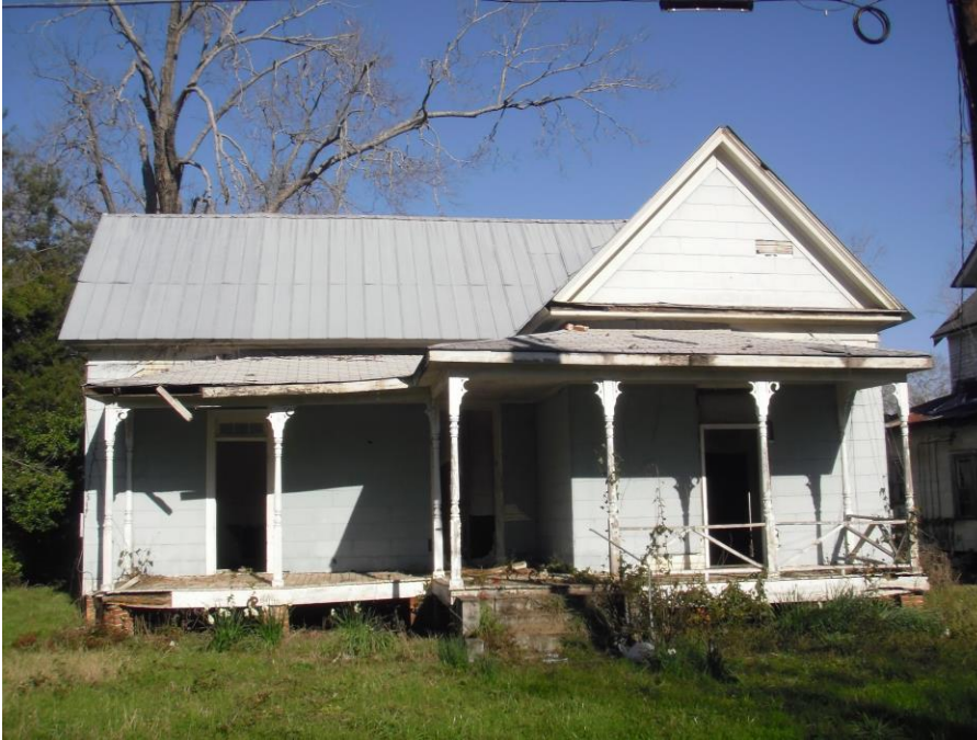
303 E. Johnson St. – siding tested positive for asbestos
