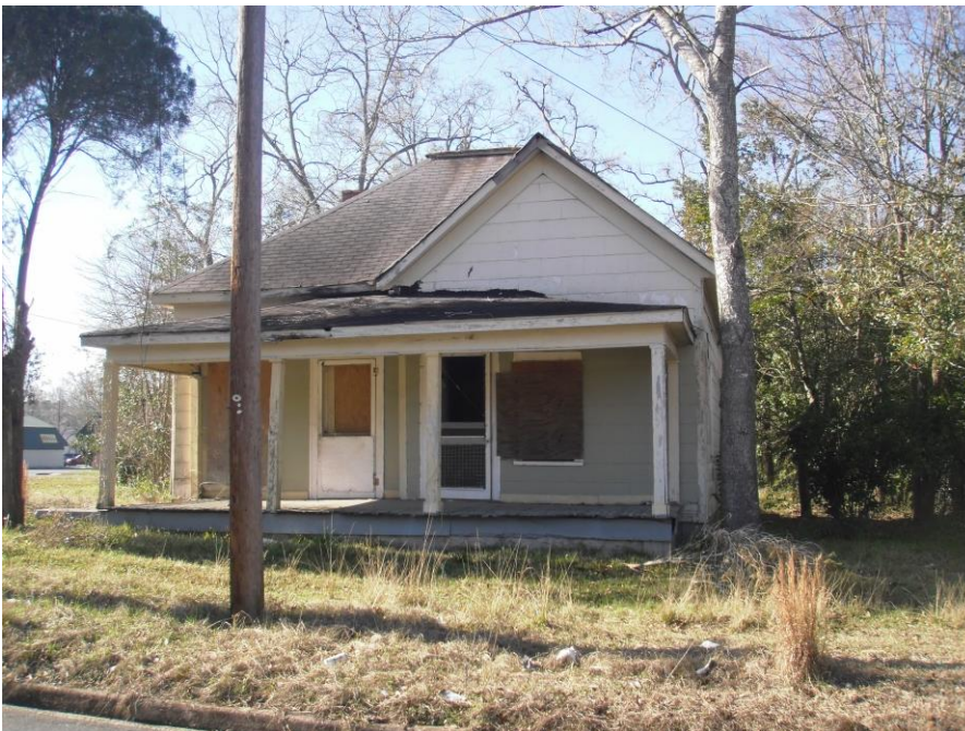
910 N. Franklin St. - siding tested positive for asbestos
