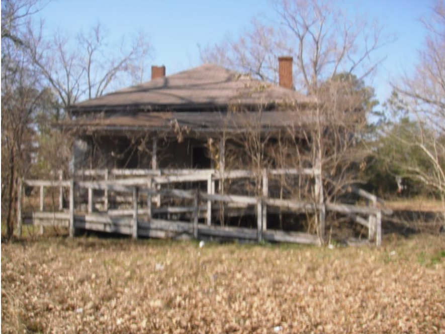
101 Forest Ave. – siding tested positive for asbestos
