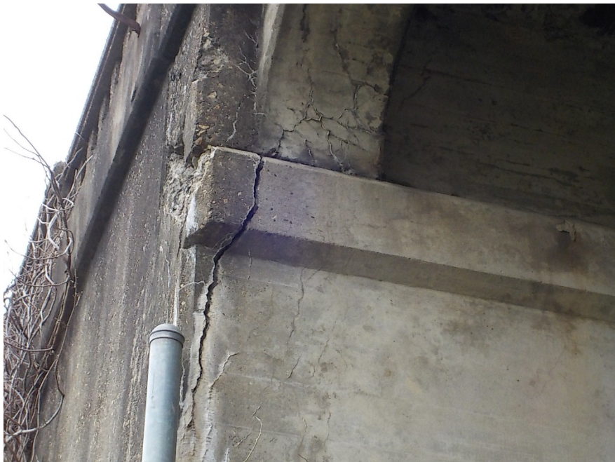
ABUTMENT 1 BREASTWALL CRACK
