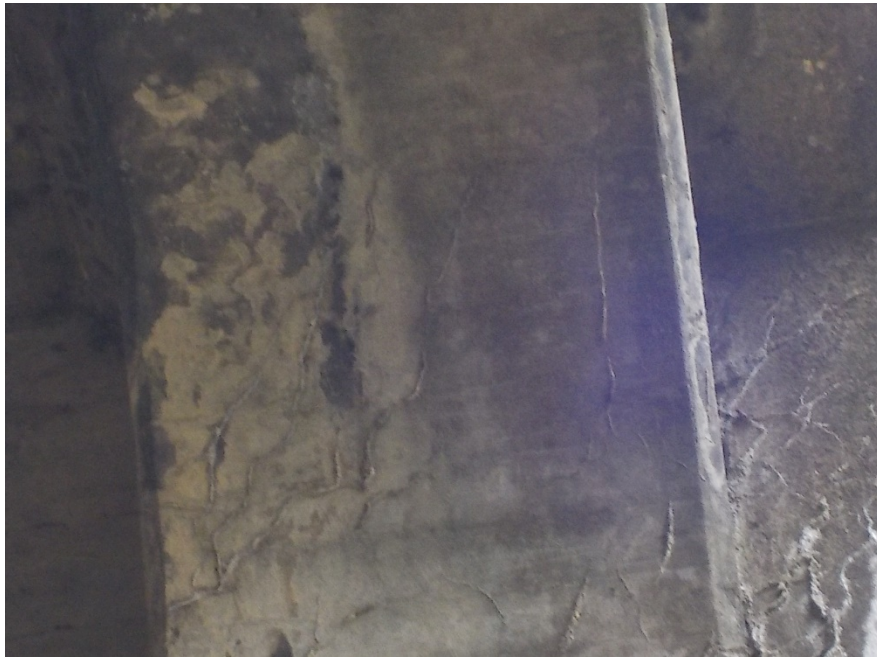
OUTSIDE BEAM CRACKING TYPICAL
